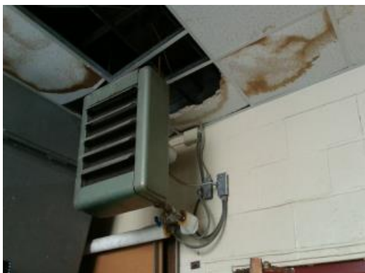
Original Unit Heater
