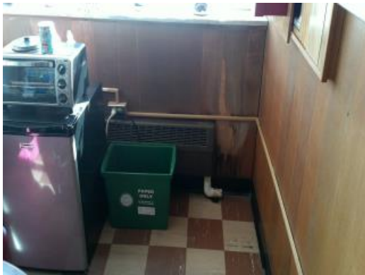
Damaged Wood Panel Walls
