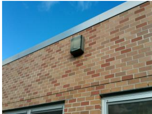
Building Mounted Light
