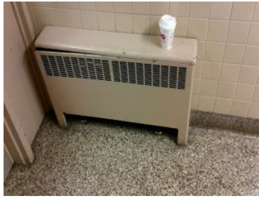
Damaged Radiant Heater
