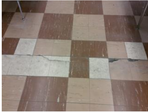
Chipped And Cracked 9X9 Tile
