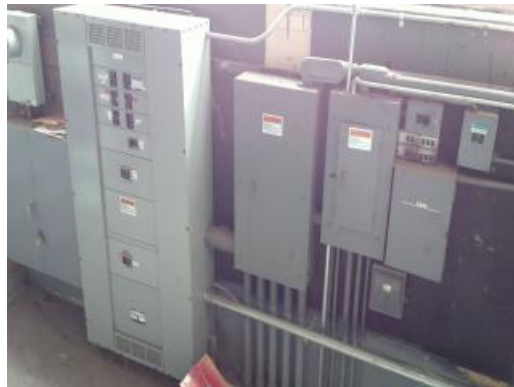
Boiler Room Panels
