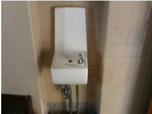
Broken Drinking Fountain
