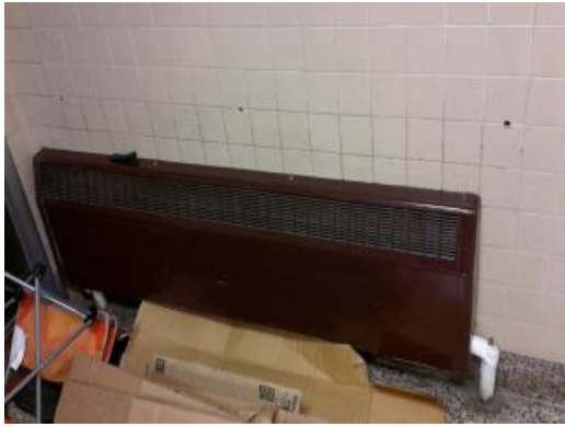
Original Radiant Heater
