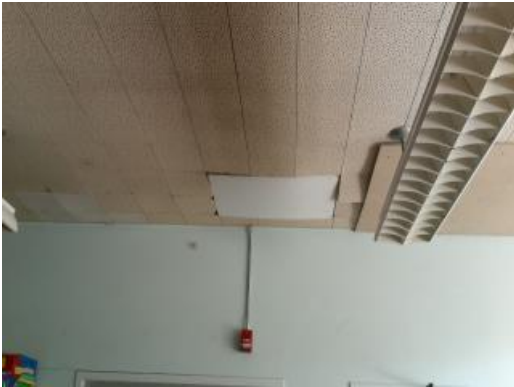
Discolored and Falling Adhered Ceiling Tiles
