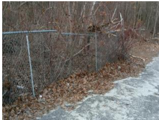
Failing Chain Link Fence
