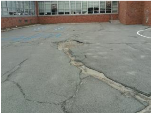
Worn Play Area Asphalt
