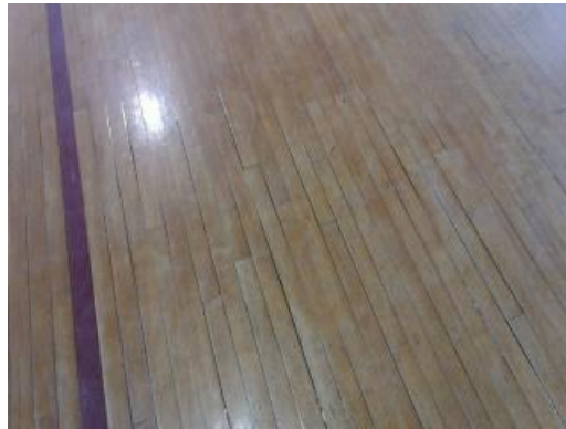
Worn Gym Floor
