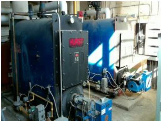
Hot Water Boilers
