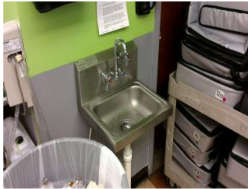
Kitchen Hand Washing Sink
