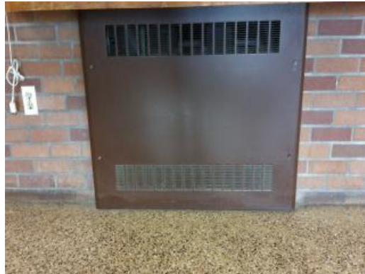
Original Unit Heater
