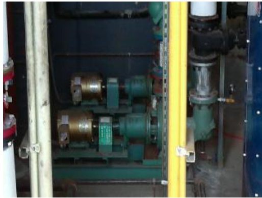
Heating Hot Water Pumps
