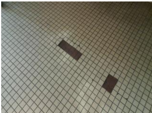
Missing Ceramic Tiles
