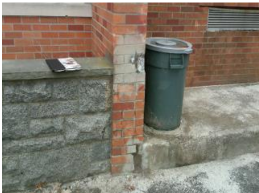
Damaged Brick Wall
