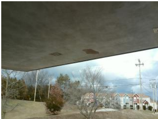
Water Damaged Soffit
