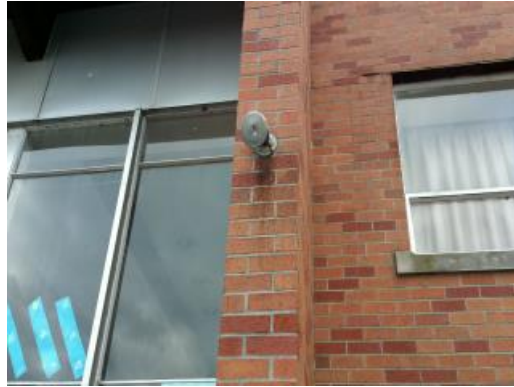
Original Building Mounted Lights
