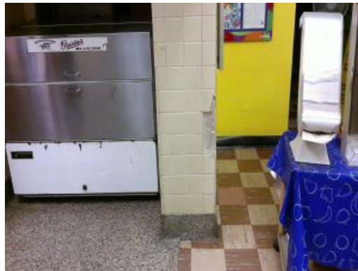
Damaged Ceramic Tile Wall
