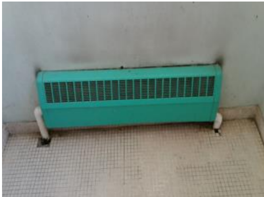
Original Radiant Heater
