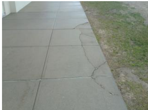
Cracked Concrete Walkway
