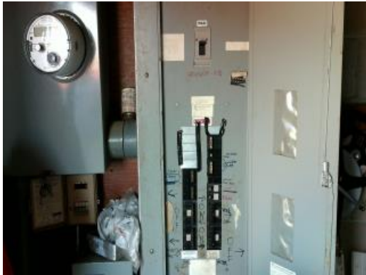
Building 02 - Outdated Panelboard
