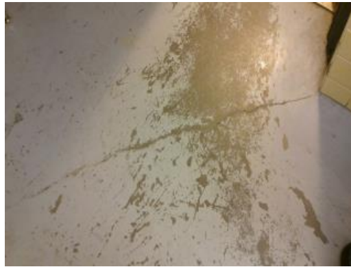
Main Building - Crack In Concrete Floor
