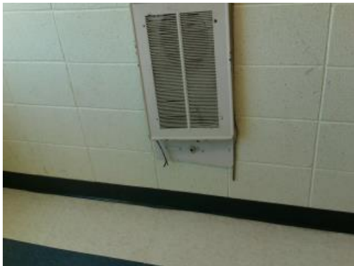
Main Building - Electric Unit Heater
