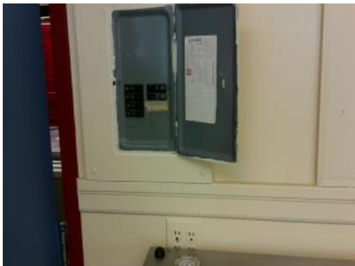
Main Building - Obsolete Panelboard
