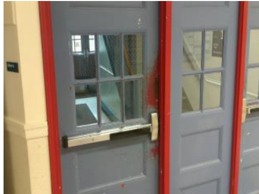
Main Building - Worn Interior Metal Doors
