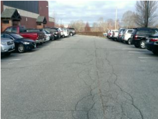
Cracked Asphalt Paving
