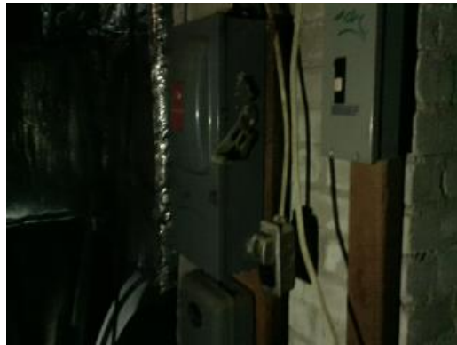
Main Building - Electrical Equipment In Attic
