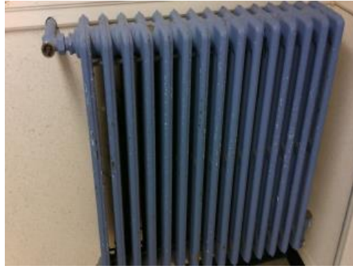
Main Building - Original Radiant Heater
