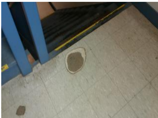
Main Building - Damaged VCT
