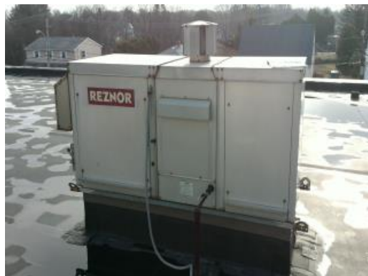
Main Building - Outdoor Air Handler
