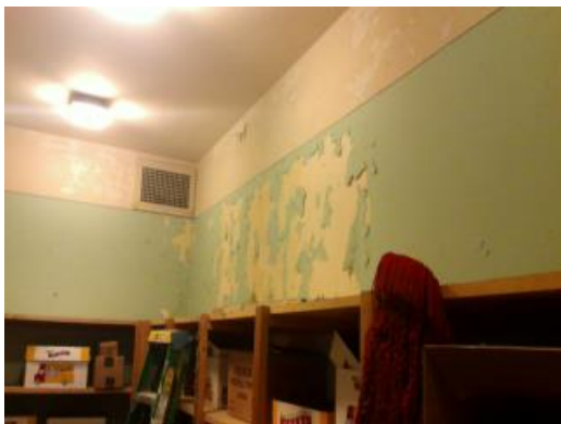
Main Building - Paint Peeling
