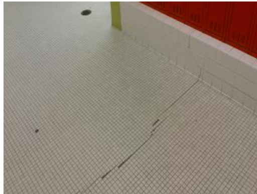
Main Building - Cracked Ceramic Tile Floor
