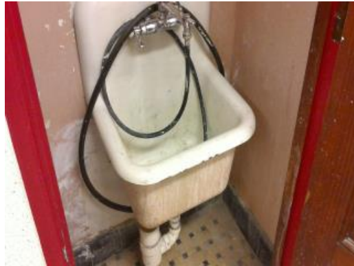
Main Building - Mop Sink
