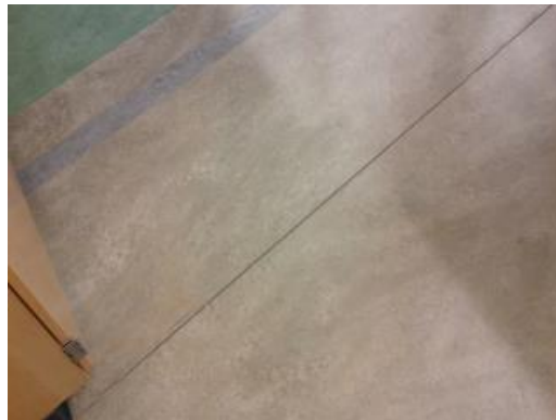
Main Building - Curling Floor Seam
