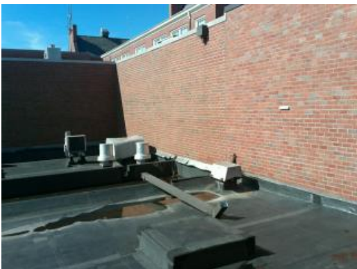
Main Building - Clogged Roof Drain
