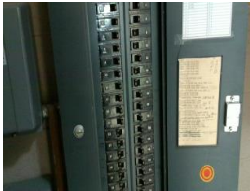
Main Building - Aged Panelboard
