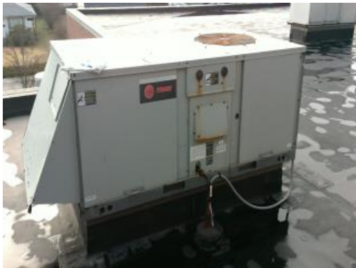
Main Building - Outdoor Air Handler
