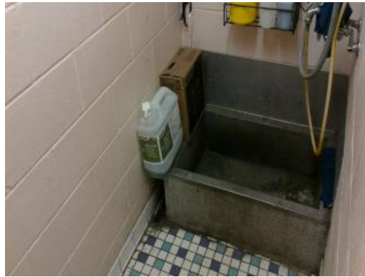
Stained Service Sink
