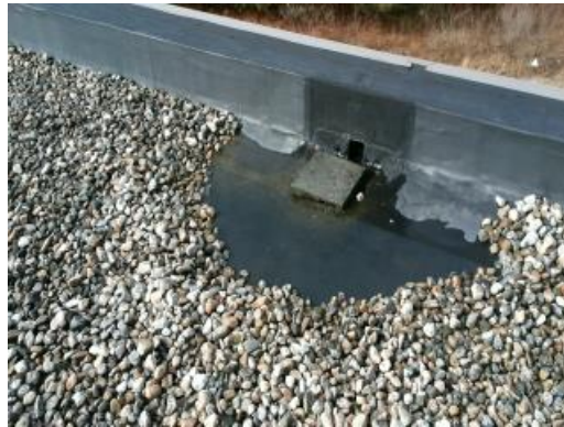
Clogged Roof Drain
