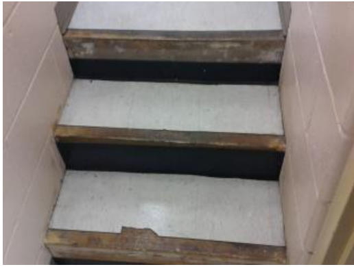
Chipped VCT On Stairs
