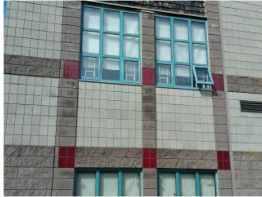
Upper Windows Seals Broken
