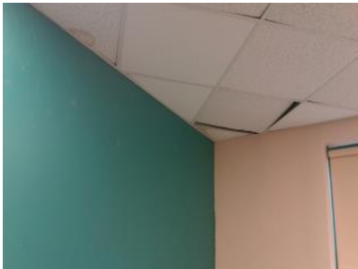
Displaced Ceiling Tiles
