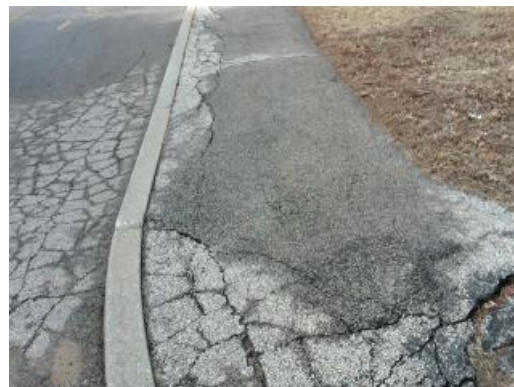
Cracked Asphalt Pavement
