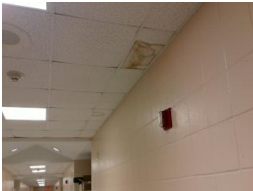
Stained Ceiling Tiles
