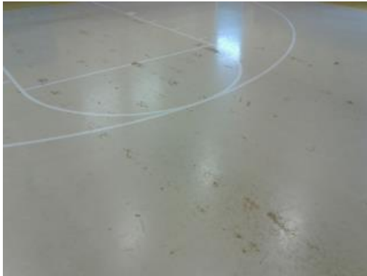
Worn Gym Floor
