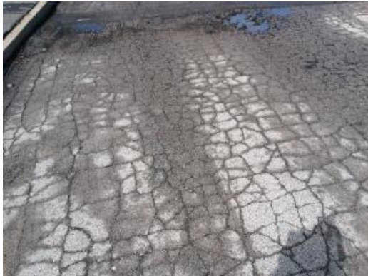
Alligatoring Asphalt Paving
