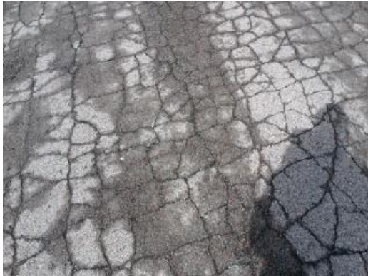
Alligatored Roadway Pavement
