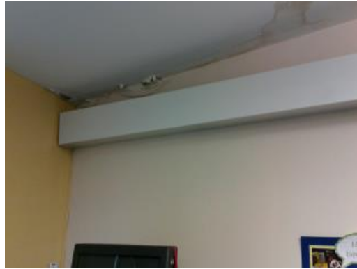
Damaged Gypsum Board Ceiling
