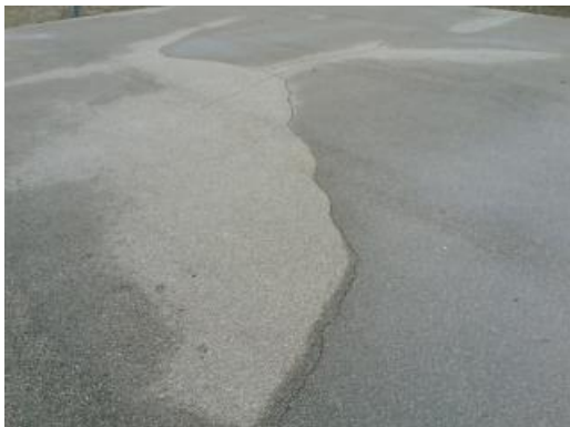
Cracked Paved Play Area
