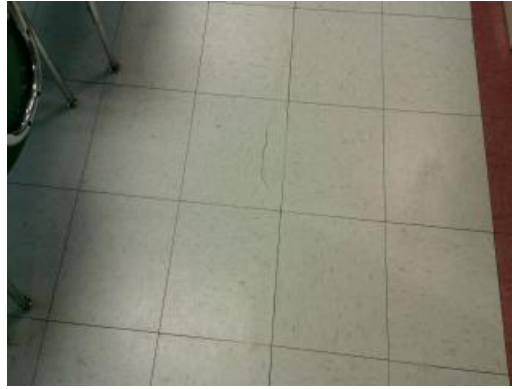
VCT Flooring Separation
