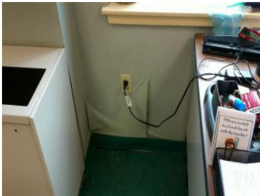
Peeling Wall Covering
