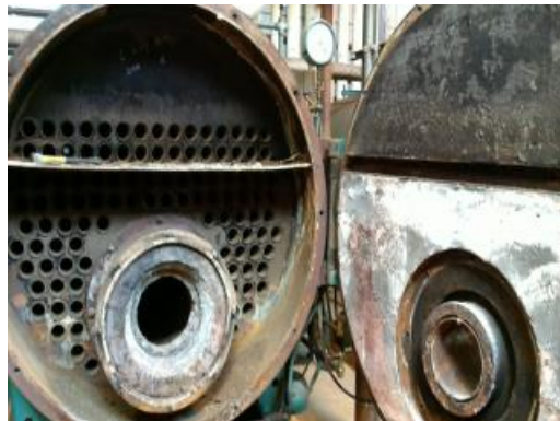
Boiler Out Of Service
