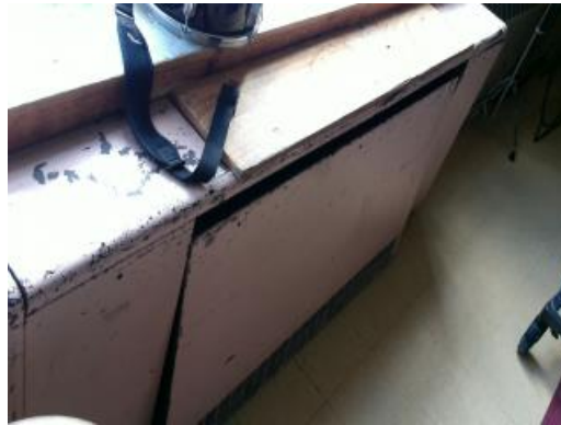
Old Unit Ventilator
