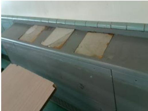
Boarded Up Unit Ventilator Out Of Service
