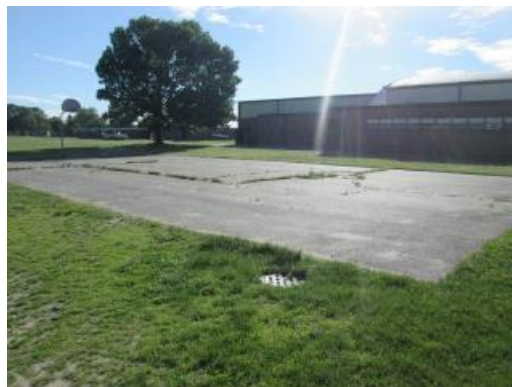
Deteriorated Basketball Court
