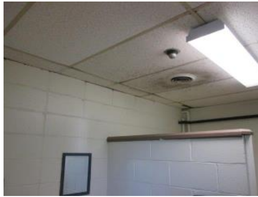
Deteriorated Acoustical Ceiling
