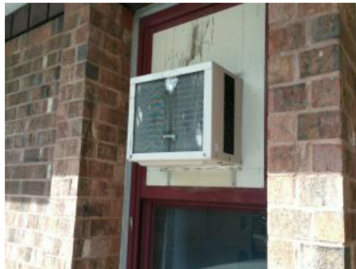
Window AC Unit
