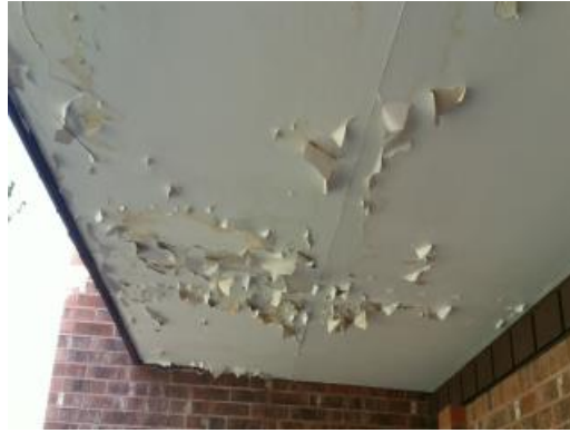
Water Damaged Soffit
