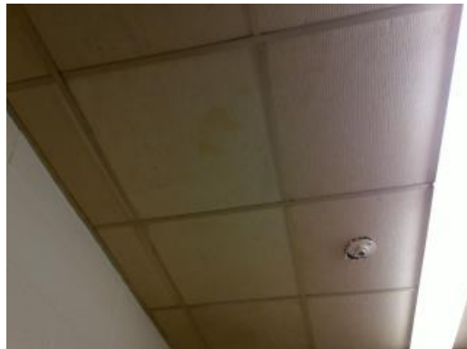
Stained Ceiling Grid
