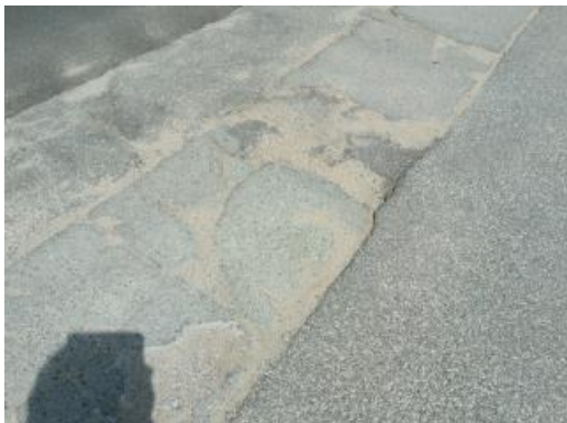
Damaged Asphalt Sidewalk
