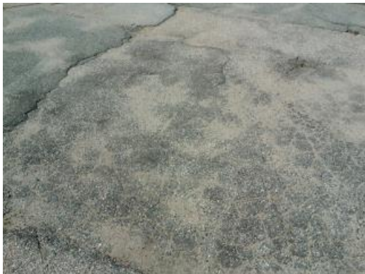
Weathered Asphalt Parking Lot
