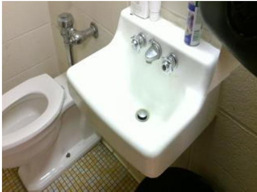
Aged Restroom Lavatory
