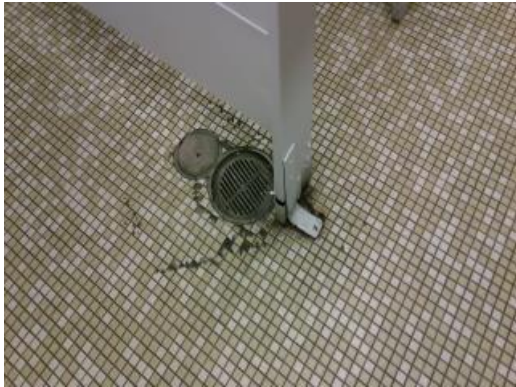
Cracked Tile Floor
