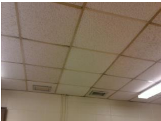
Stained Ceiling Grid
