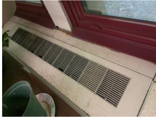
Aged Unit Ventilator
