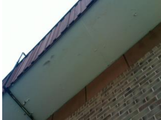
Peeling Soffit Paint
