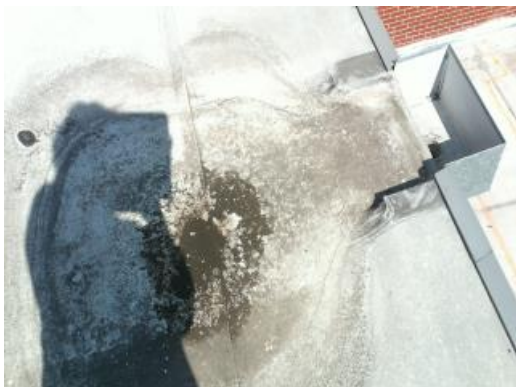
Staining At Drain
