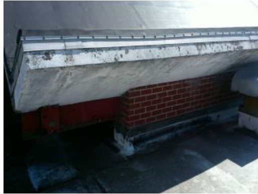
Damaged Soffit At Library
