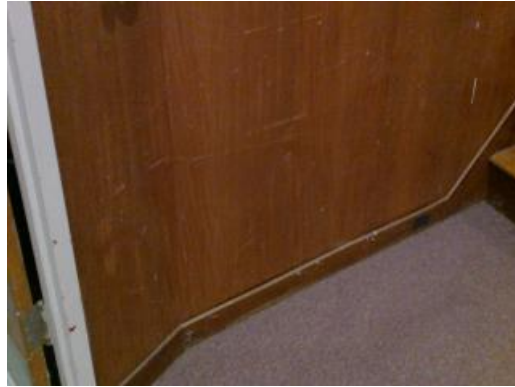
Scratched And Delaminating Wood Wall
