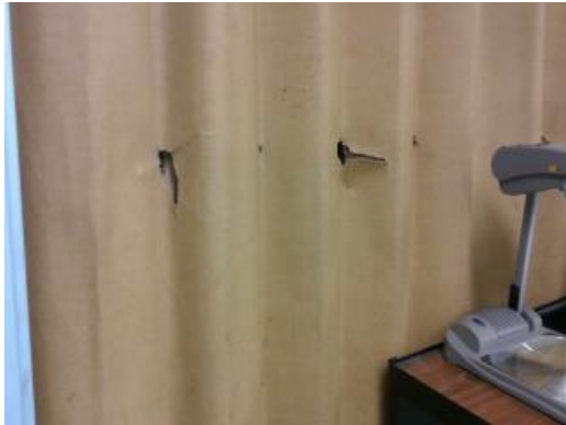
Typical Stained And Torn Partition
