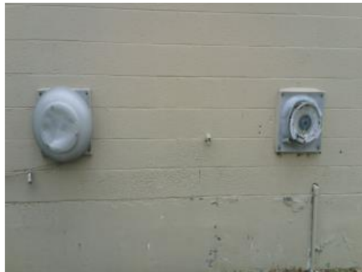
Septic House Exhaust Fans
