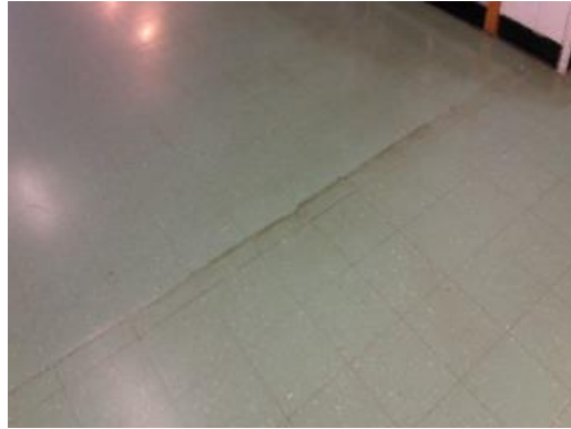
Cracked 9X9 Tile
