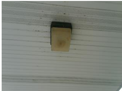
Original Canopy Lighting
