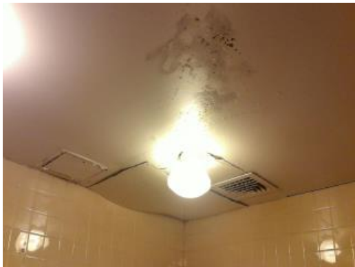
Stained Gypsum Ceiling
