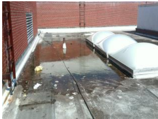
Ponding On Roof
