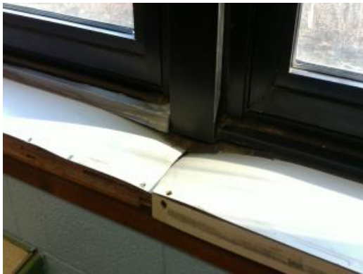
Water Damaged Sill
