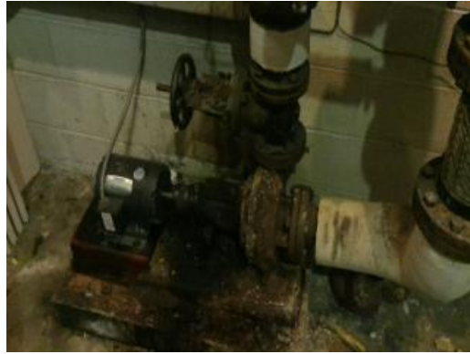
HVAC Circulating Pump
