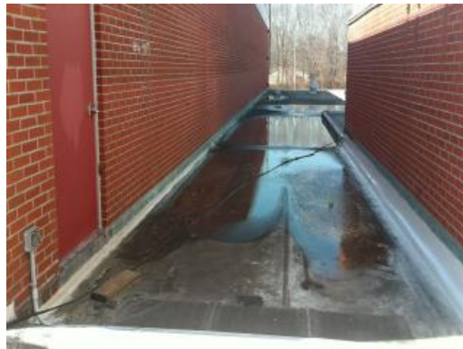
Ponding On Low Roof Above Music Room
