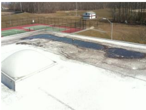
Ponding At Gym Roof Edge
