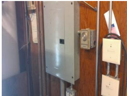
Maintenance Shed Electrical Panel
