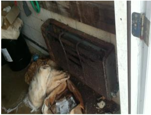
Septic House Electric Unit Heater
