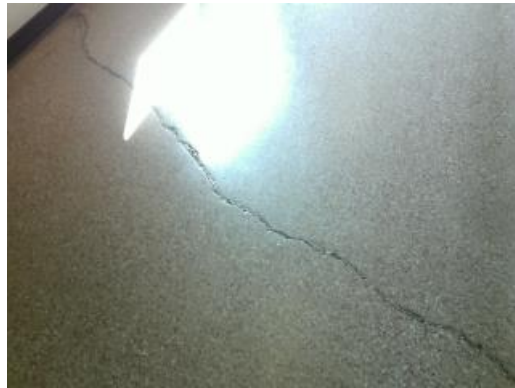
Cracked Terrazzo Flooring
