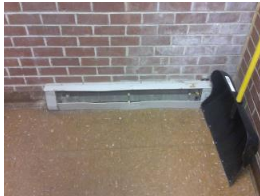
Original Radiant Heaters
