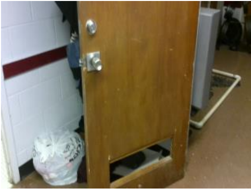
Chipped And Worn Wood Door
