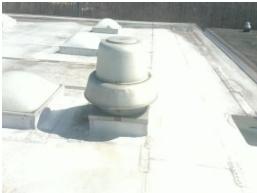
Non-Functional Exhaust Fan
