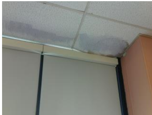
Stained Ceiling Tiles
