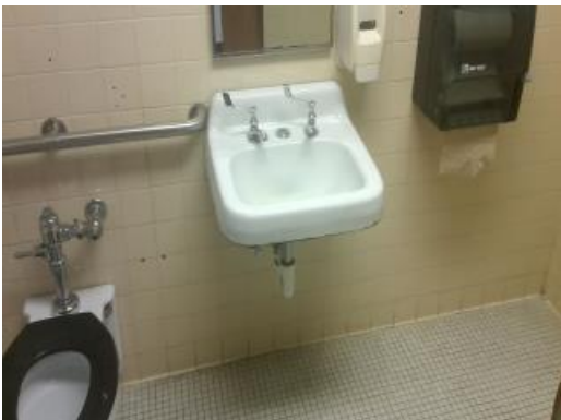
Maintenance Shed Restroom Fixtures
