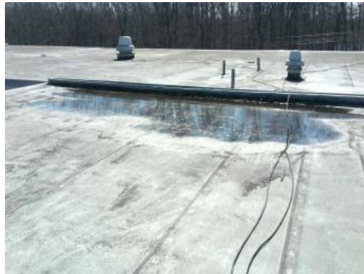
Ponding At Expansion Joint
