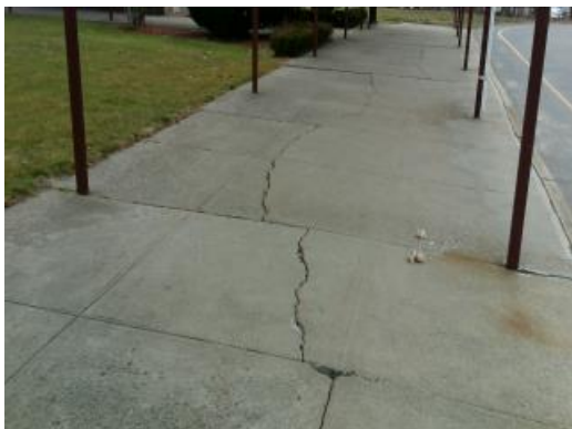
Front Entry Cracked Sidewalk
