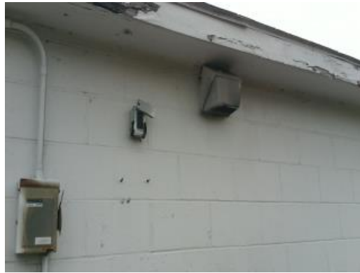
Building 3 Building Mounted Light
