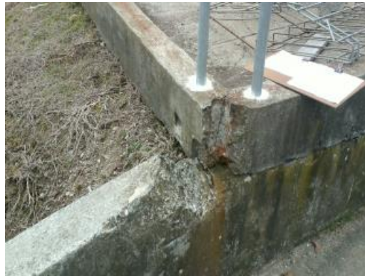
Broken Concrete Retaining Wall
