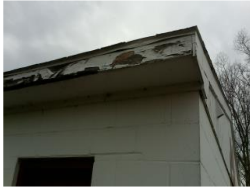
Building 3 Damaged Roof Fascia
