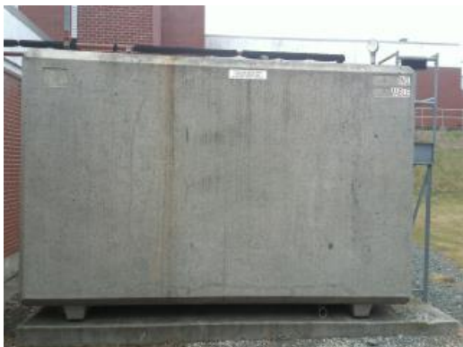
Diesel Storage Tank
