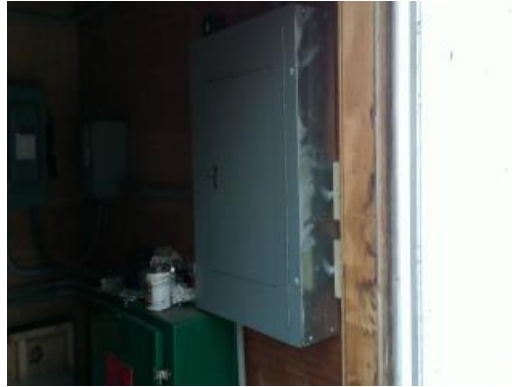
Building 4 Electrical Panel
