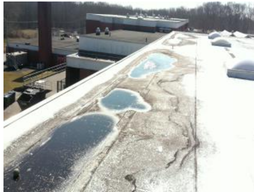
Ponding At Roof Edge
