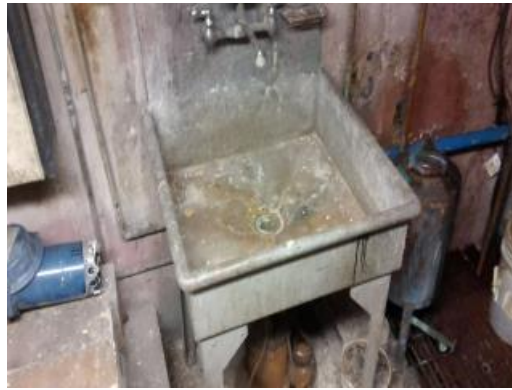
Corroded Utility Sink
