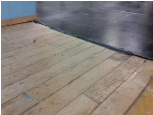
Worn Wood Floor
