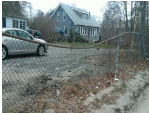
Rusted And Falling Fence
