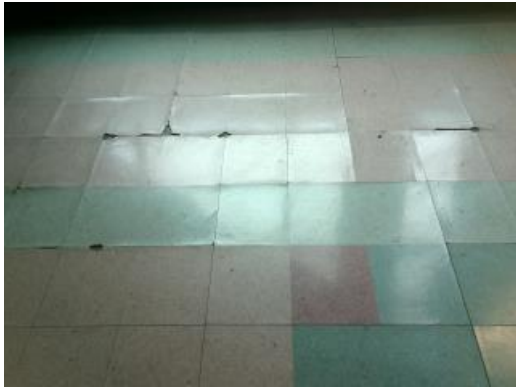
Chipped And Curling VCT
