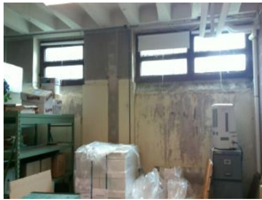
Peeling Paint In Storage
