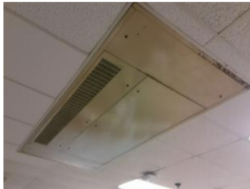
Rusted And Molding Split System
