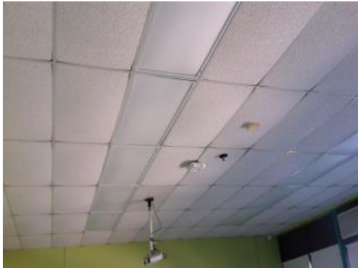
Stained And Sagging Ceiling Tiles
