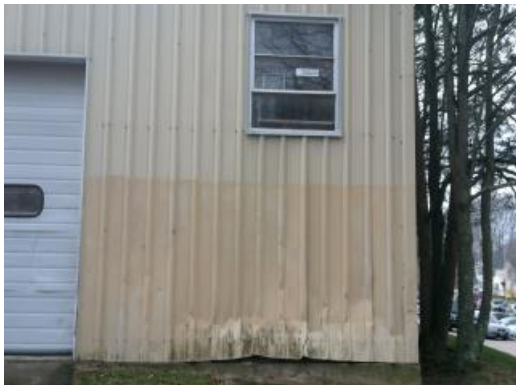
Damaged Metal Panel Wall
