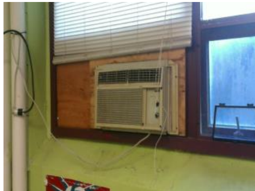
Failing Window Unit
