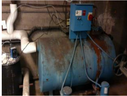
Rusted Condensate Receiver
