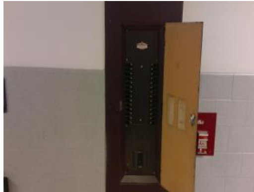
Aged 225 Amp Panelboard
