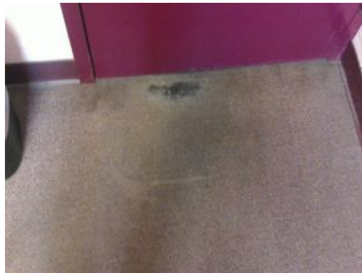
Worn And Stained Carpet
