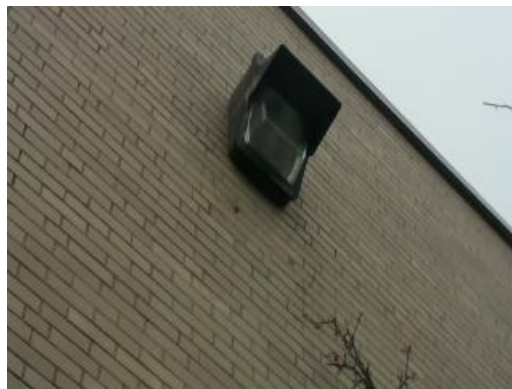
Building Mounted Light
