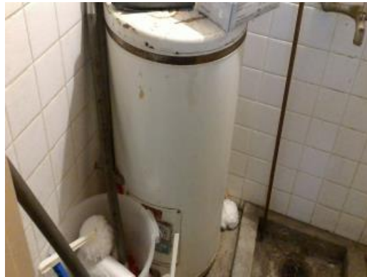
Typical Rusted Water Heater
