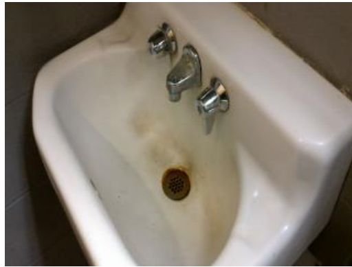
Stained Restroom Lavatory
