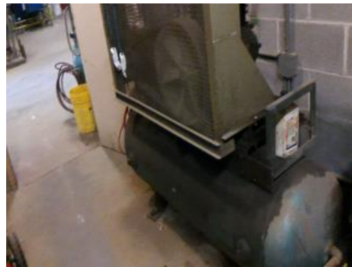
Abandoned Air Compressor
