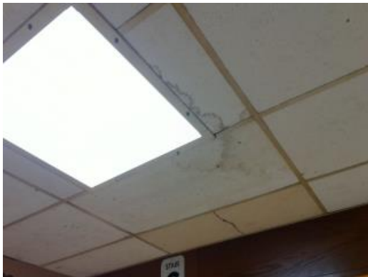
Aged And Stained Ceiling Grid And Tiles
