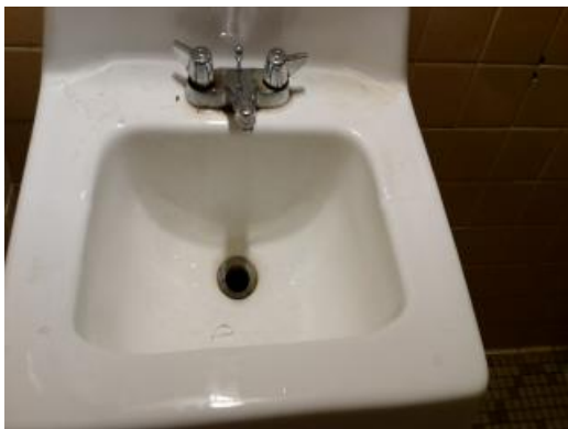
Cracked Restroom Lavatory
