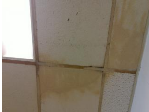
Stained Ceiling Tiles And Grid
