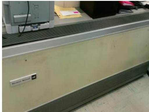
Typical Aged Heating Unit
