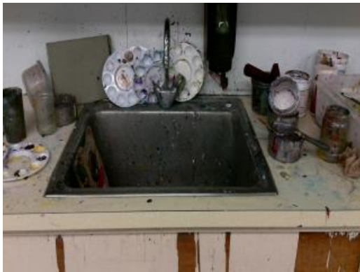
Stained Classroom Lavatory
