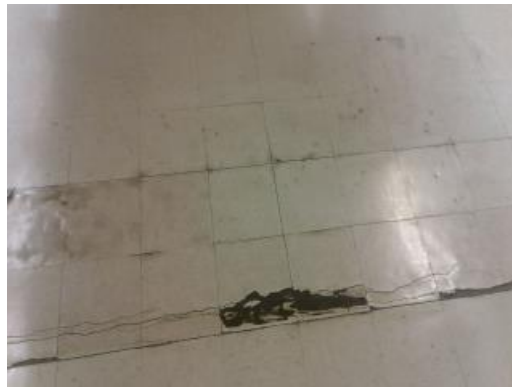
Cracked And Worn VCT
