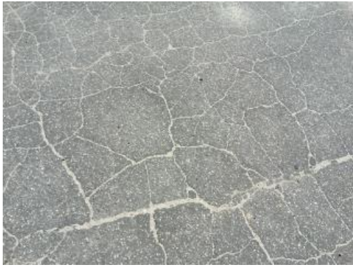
Alligatored Asphalt Pavement
