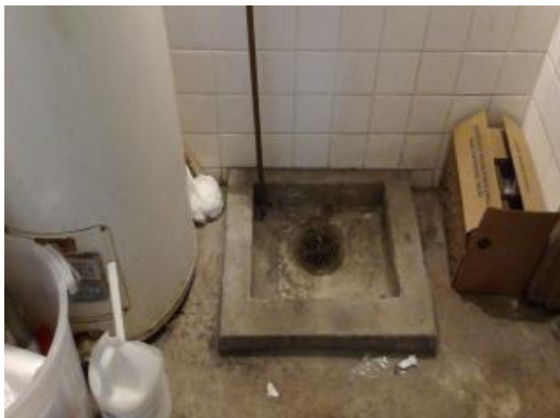
Corroded Mop Sink
