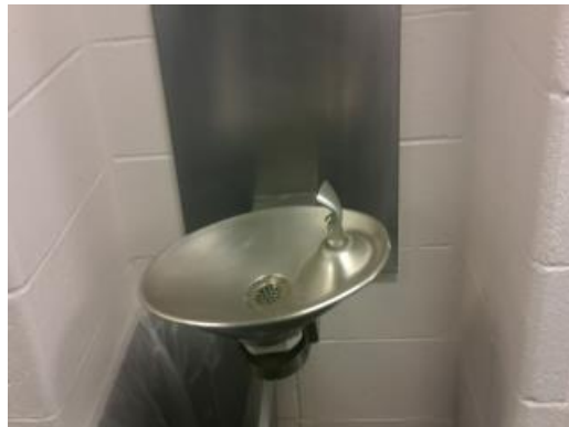
Non-Functional Drinking Fountain
