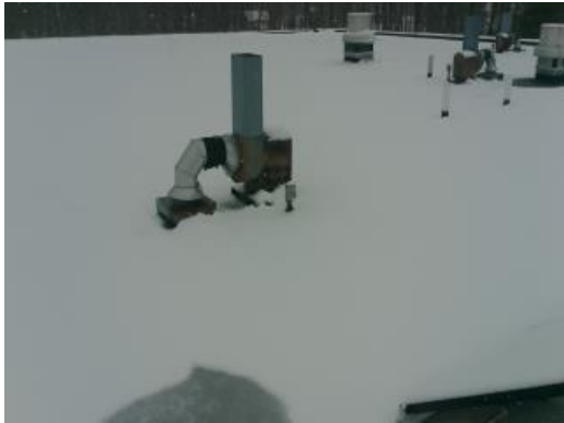
Lab Fume Hood Exhaust
