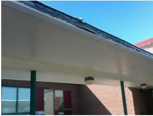
Damaged Canopy Roof Edge
