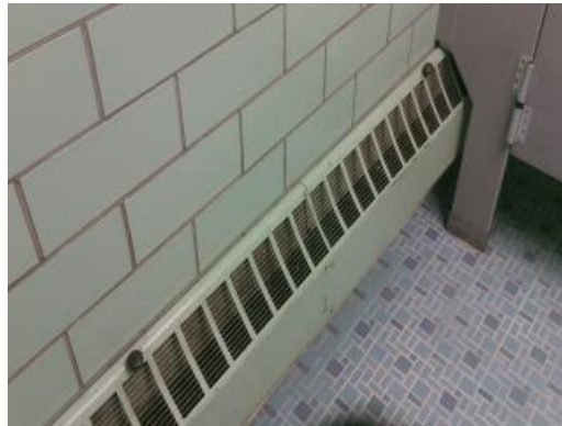
Typical Aged Radiant Heater
