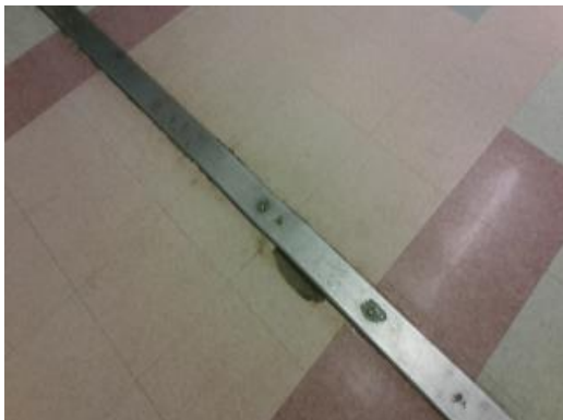
Lifted Joint Cover With Damaged VCT
