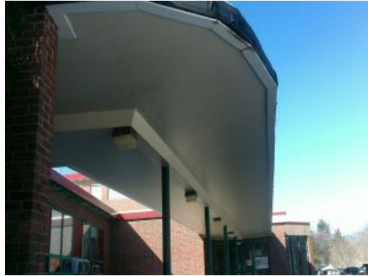
Damaged Canopy Roof Edge
