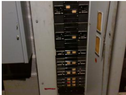
Aged Distribution Panel
