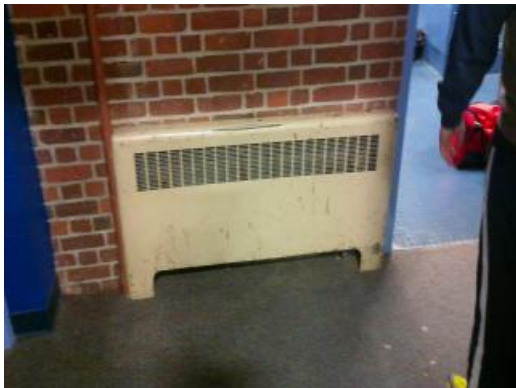
Typical Deteriorating Radiant Heater
