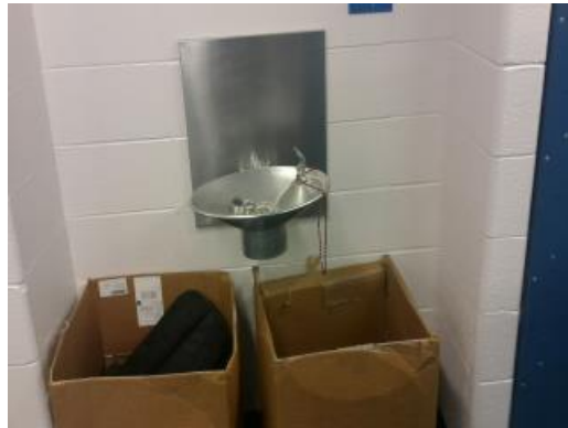
Non-Functional Drinking Fountain
