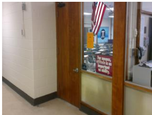
Non-Compliant Door Hardware
