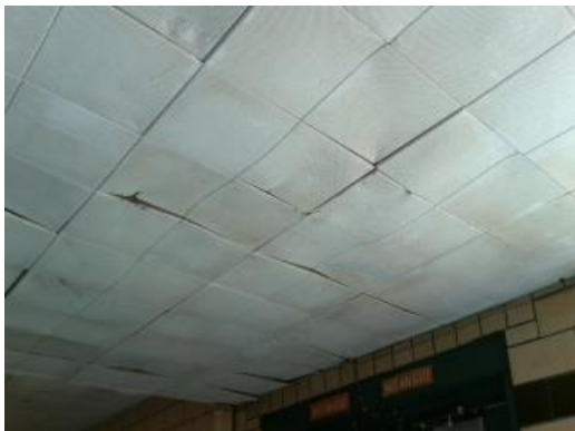
Stained And Warped Adhered Ceiling Tiles
