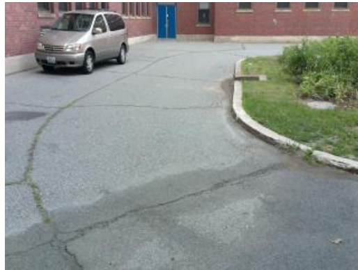
Cracked And Worn Asphalt Roadway
