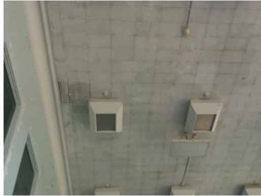
Worn Adhered Ceiling
