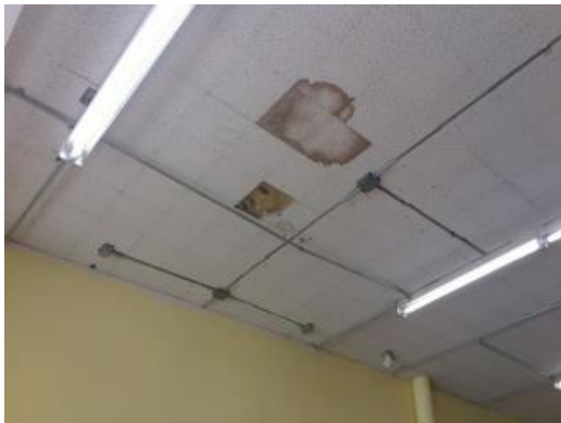
Stained And Missing Adhered Tiles
