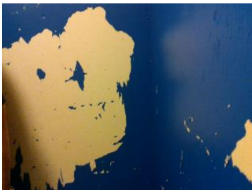
Peeling Wall Paint
