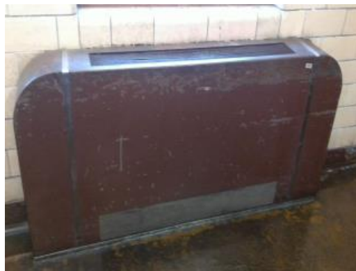
Original Unit Vent
