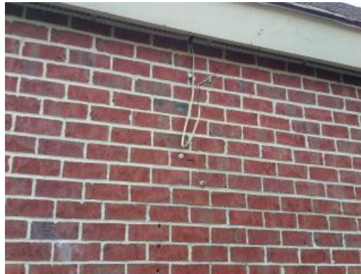
Missing Building Mounted Light Fixture
