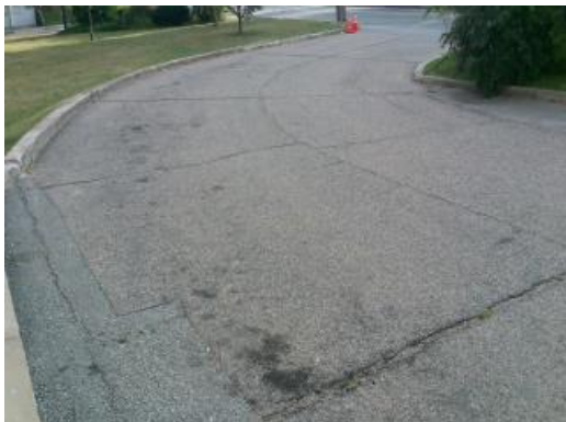
Worn Asphalt Drive
