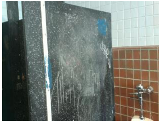
Graffiti On Toilet Partition
