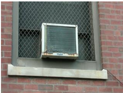
Damaged Window Unit
