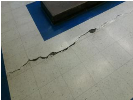
Cracked Floor In Girl's Locker Room
