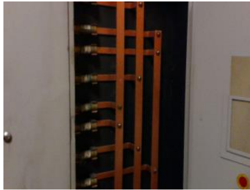
Abandoned Fuse Box
