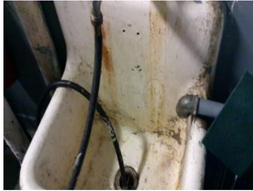
Rusted Mop Sink
