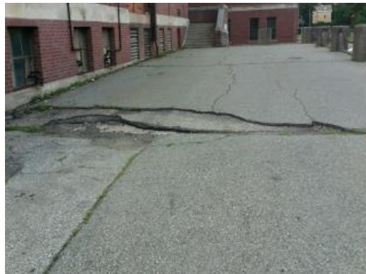
Cracking And Failing Asphalt Pavement
