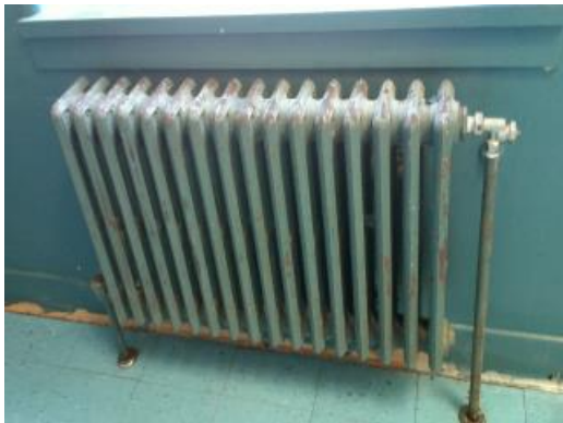
Rusted Radiant Heater
