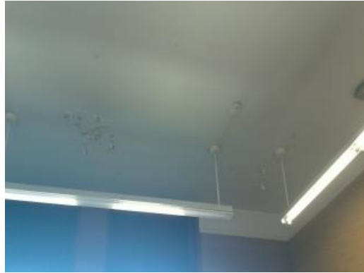
Peeling Ceiling Paint
