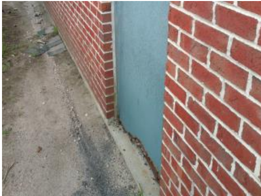
Rusted Exterior Door
