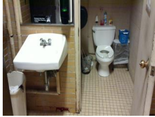
Damaged Ceramic Tile Flooring
