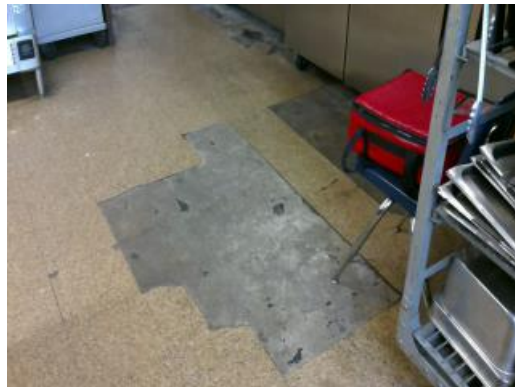
Damaged VCT Flooring
