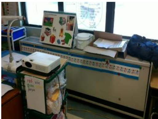
Heating Unit Ventilator
