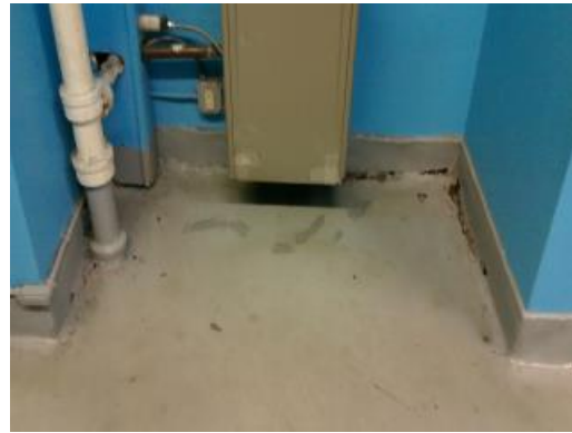
Damaged Epoxy Flooring
