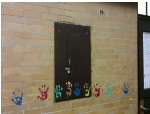
Electrical Subpanel in Corridors
