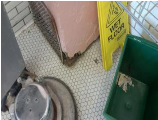
Damaged Ceramic Tile Flooring
