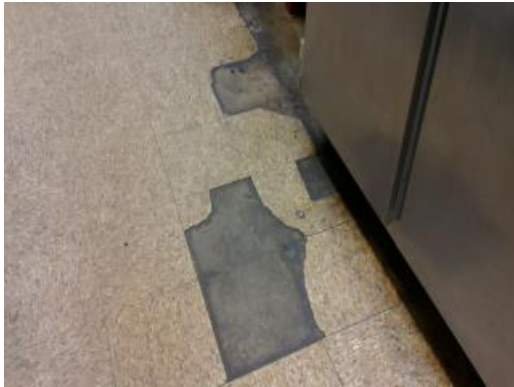
Damaged VCT Flooring
