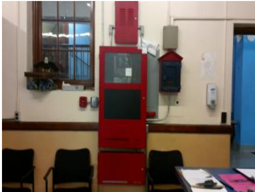
Fire Alarm Control Panel
