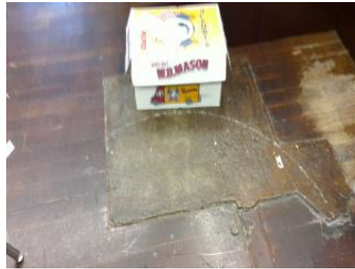
Damaged Wood Flooring
