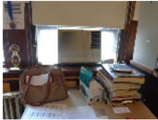
Window Air Conditioning Unit - Office
