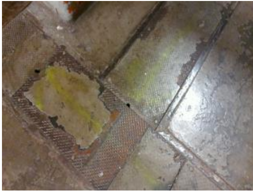
Damaged Epoxy Flooring
