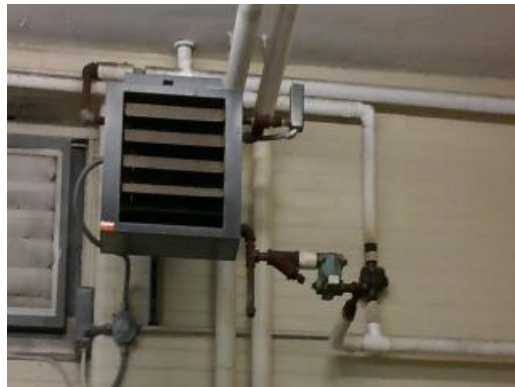
Rusted Unit Heater
