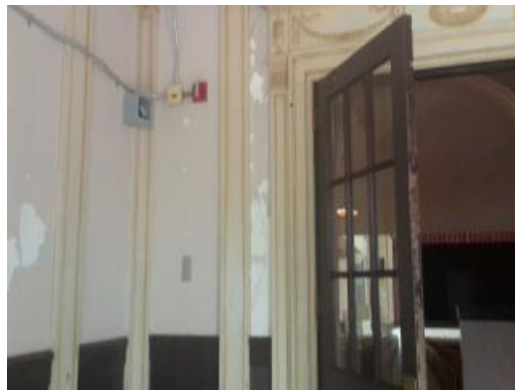
Damaged Plaster Wall
