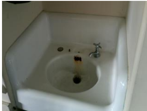
Rusted Classroom Lavatory
