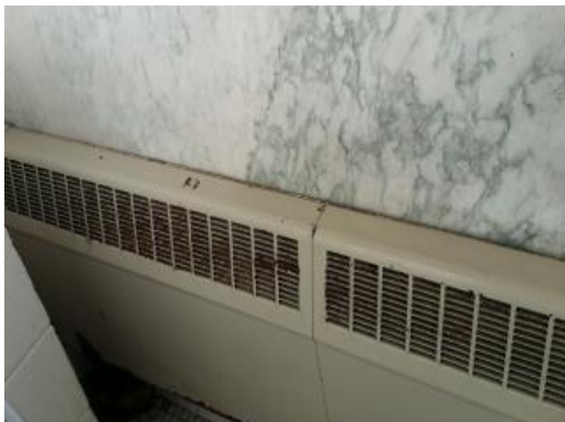
Rusted Fin Tube Heater
