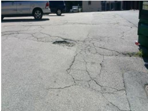
Cracked Asphalt Paving
