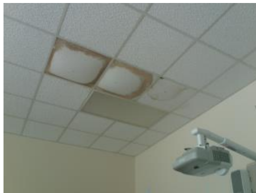
Stained And Sagging Ceiling Tiles
