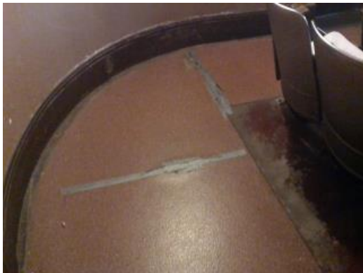
Cracked Vinyl Flooring
