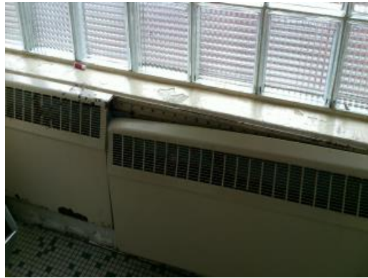
Damaged Fin Tube Heater
