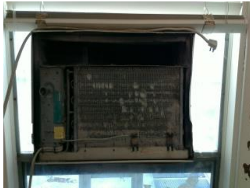
Damaged Window Unit
