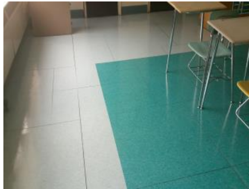
VCT Lifting At Seams
