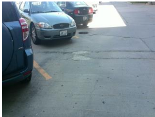
Cracked And Spalled Concrete Parking
