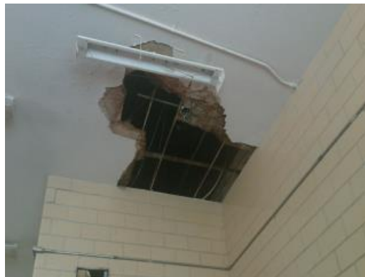
Damaged Plaster Ceiling
