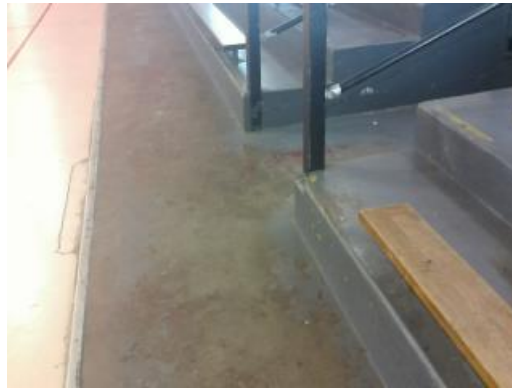
Worn Floor Finish
