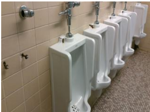
Broken And Missing Urinals
