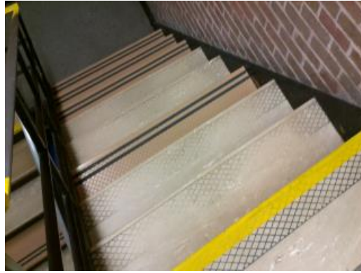
Worn Or Missing Stair Tread
