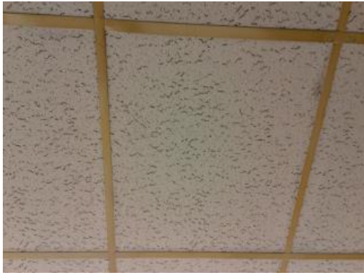
Stained Ceiling Grid
