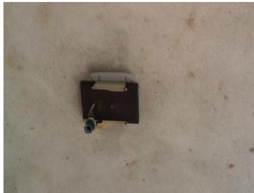
Broken Canopy Fixture
