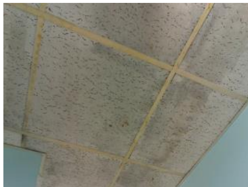
Stained Ceiling Tiles
