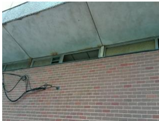
Aged And Rusted Windows
