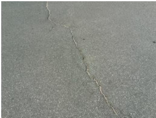
Weathered Parking Lot Pavement
