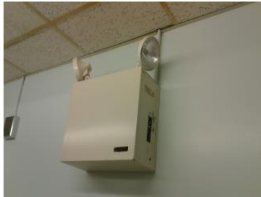
Typical Emergency Light
