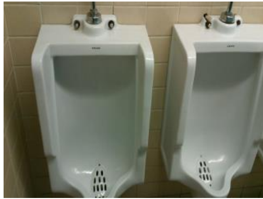
Typical And Broken Urinal
