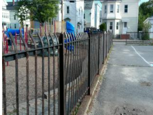
Rusted Ornamental Fencing
