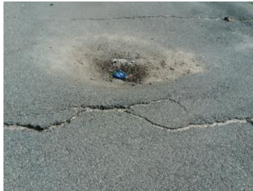
Cracks And Pothole In Parking Lot
