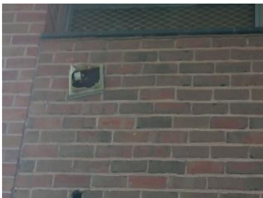
Broken Building Mounted Fixture
