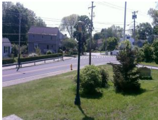
Non-Functional Pole Light
