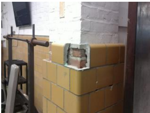
Broken And Missing Tile
