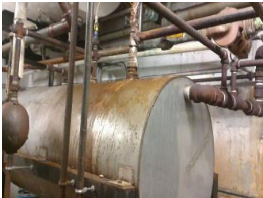
Rusted Condensate Tank
