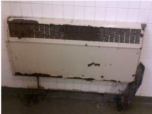
Rusted Fin Tube Heater
