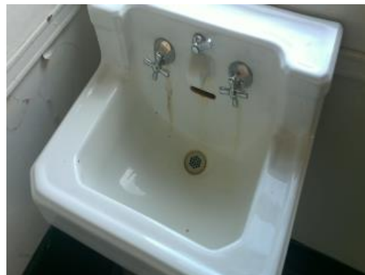
Aged Restroom Lavatory
