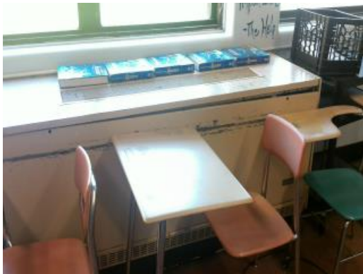
Non-Functional Unit Vent
