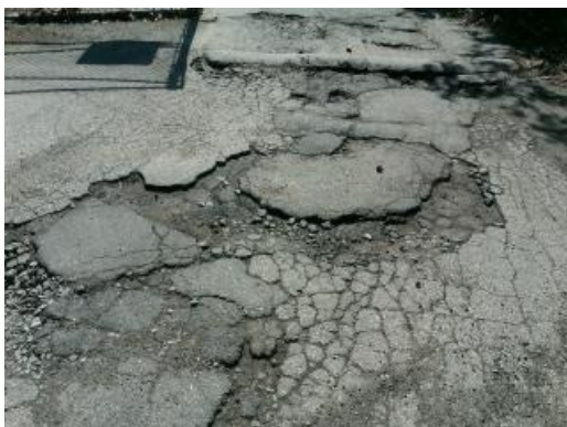
Deteriorated Parking Lot Asphalt
