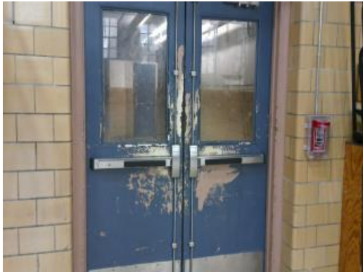
Worn Door Paint
