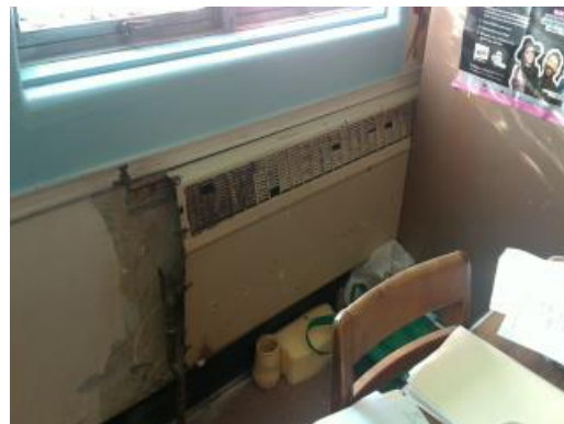
Broken Fin Tube Heater
