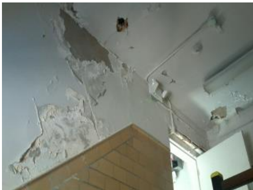
Peeling Wall Paint
