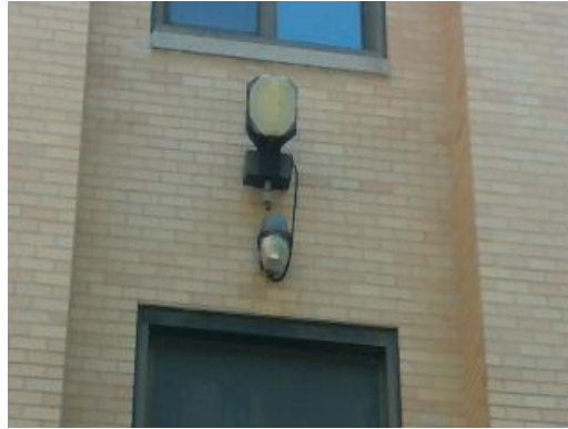
Building Mounted Fixtures
