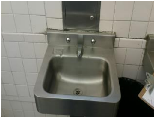
Rusted Restroom Lavatory
