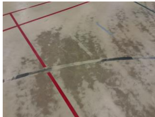
Worn Gymnasium Floor
