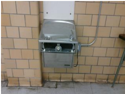
Broken Drinking Fountain
