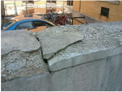
Cracked Concrete Wall
