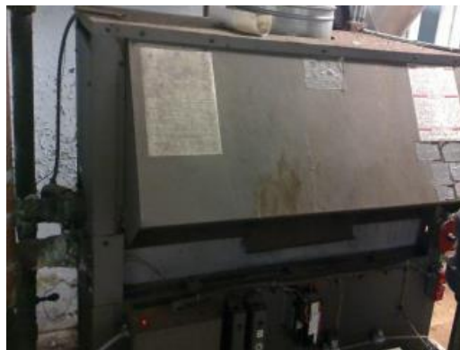
Domestic Hot Water Boiler
