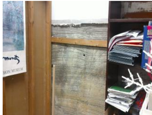
Missing Ceramic Tile
