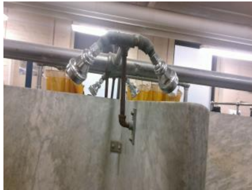
Aged Shower Fixtures
