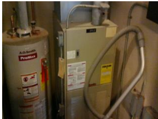
Furnace And Water Heater
