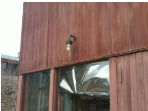
Building Mounted Light
