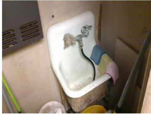
Stained Service Sink
