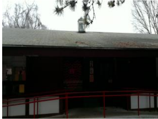
Shingles Missing From Building 2 Roof
