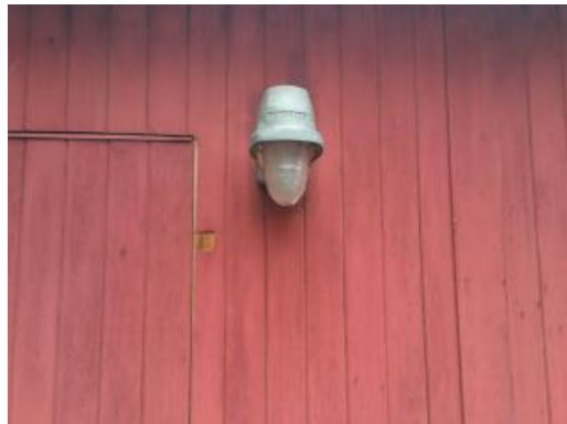
Building Mounted Light
