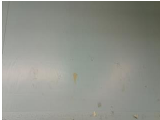
Chipped And Faded Interior Walls
