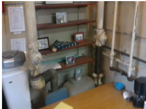
Gas Service Valve
