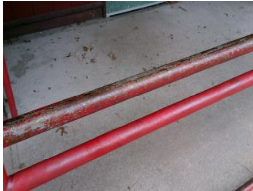
Typical Worn Handrail
