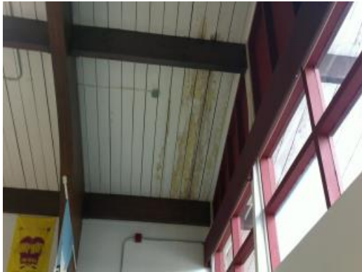
Stained Wood Decking
