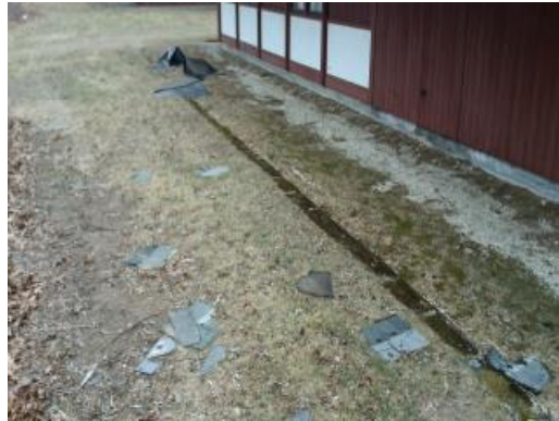
Displaced Roof Shingles
