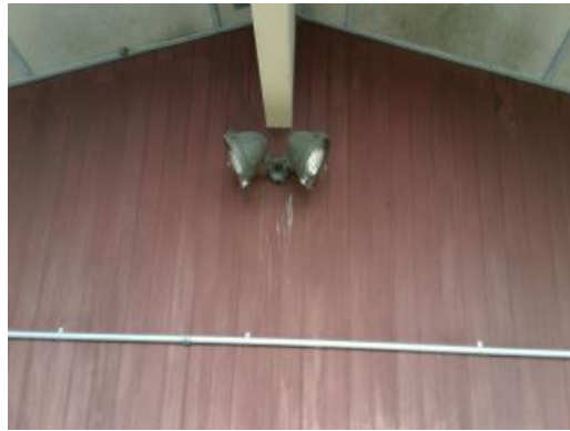
Building Mounted Light
