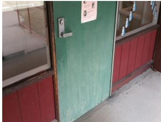
Faded Exterior Door
