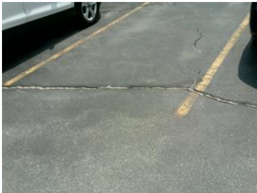
Weathered Parking Lot Paving
