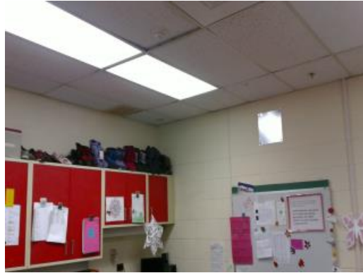
Stained And Sagging Ceiling Tiles
