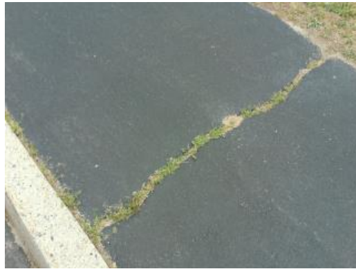
Cracked Asphalt Walkway
