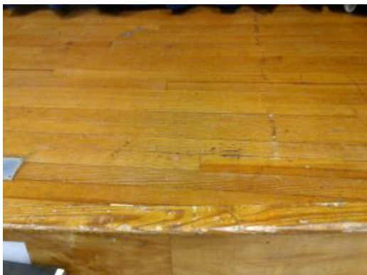
Worn Stage Floor
