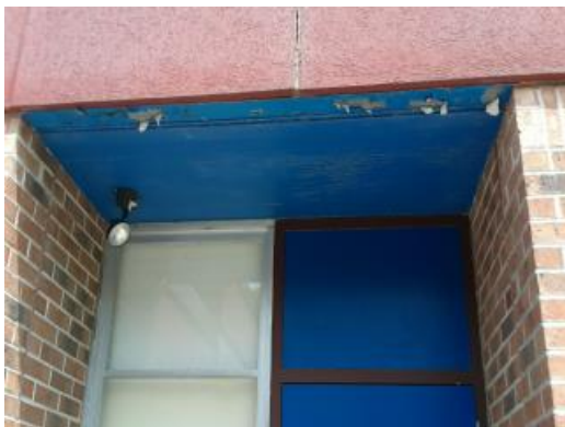
Peeling Soffit Paint
