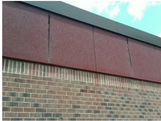
Weathered Caulking At EIFS
