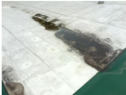
Pooling On Roof
