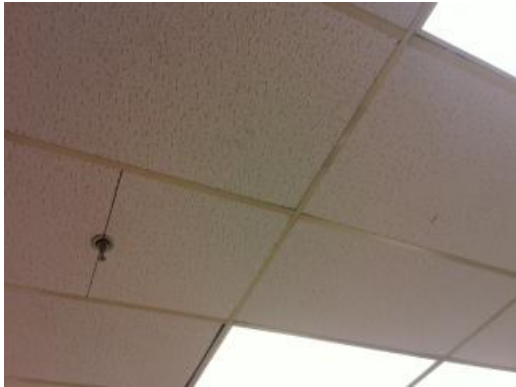
Stained Ceiling Grid
