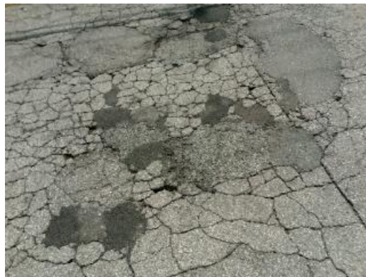
Alligatored Asphalt Paving
