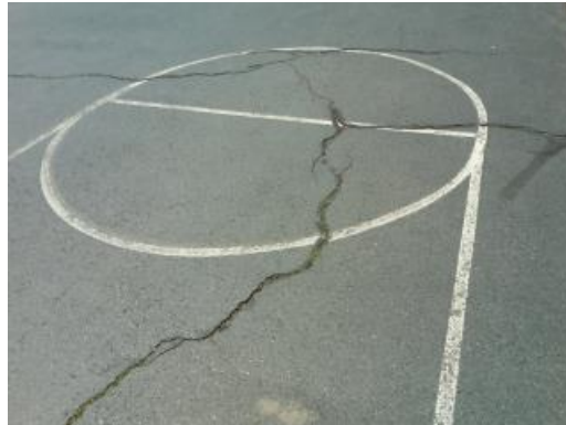
Cracked Paved Play Area
