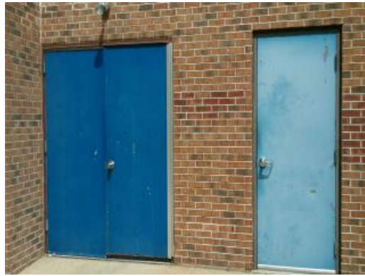
Aged Exterior Doors
