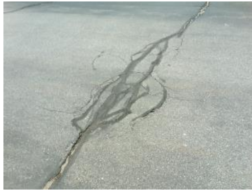
Cracked Asphalt Roadway
