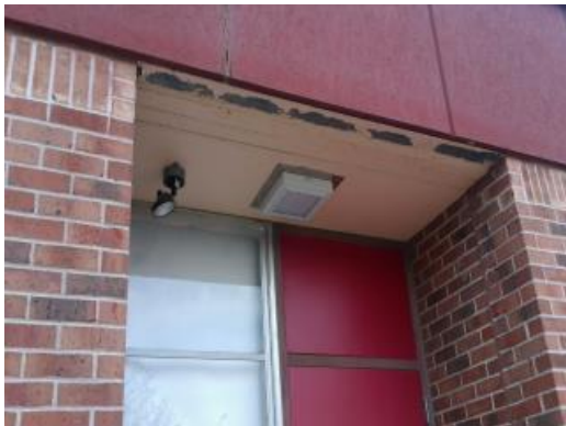
Peeling Soffit Paint
