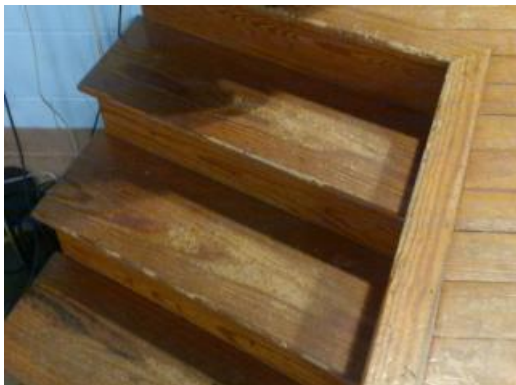
Worn Wood Stairs
