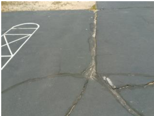
Cracked Play Area Asphalt
