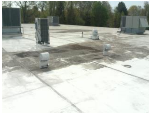
Ponding On Roof
