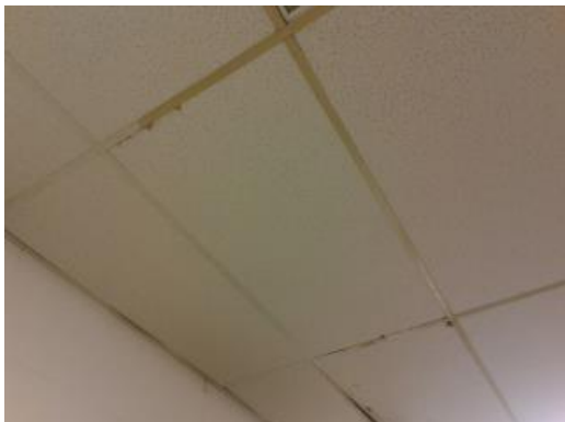
Stained Ceiling Grid
