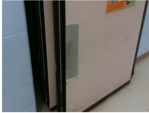
Damaged Partition Wall
