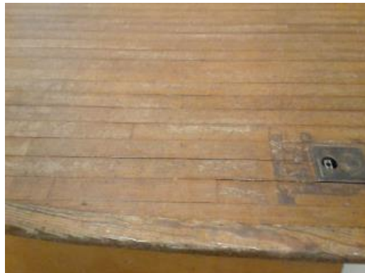
Worn Wood Floor
