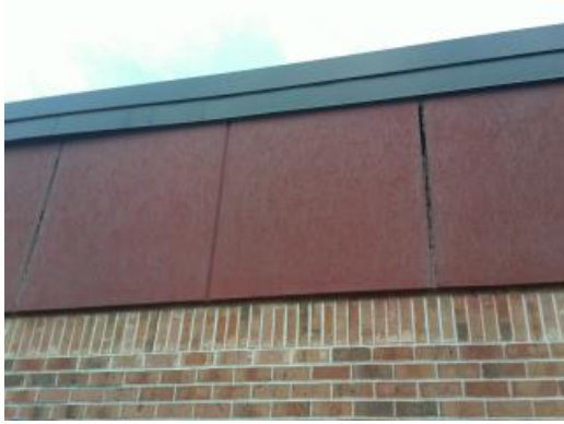
Failing Caulking At EIFS Panels
