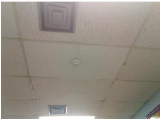
Sagging Mismatched Ceiling Tiles
