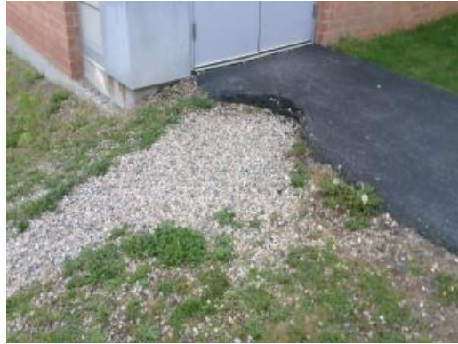
Damaged Asphalt Walks
