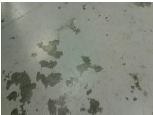
Worn Concrete Flooring At Lockers
