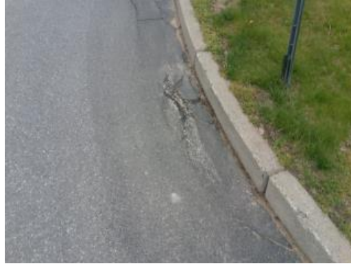
Worn Asphalt Roadway Pavement
