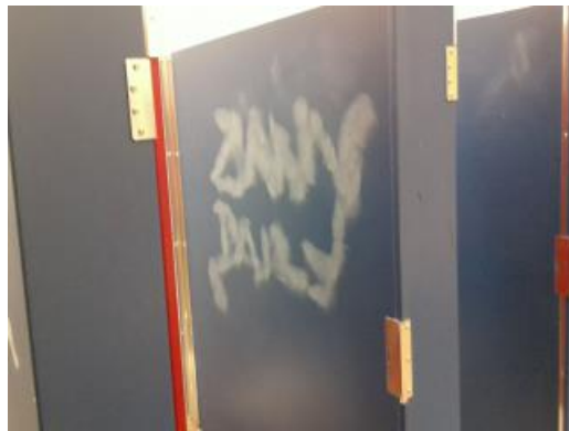
Damaged Partition At Girls Restroom
