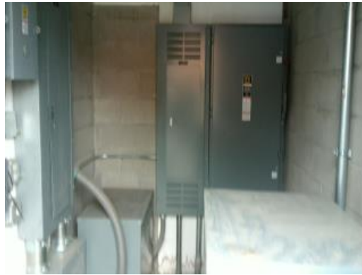
Utility Building-2 Electrical Panels
