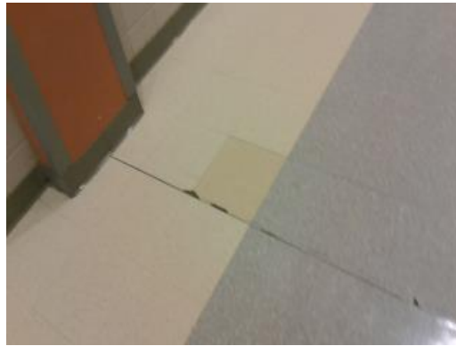
Cracked Flooring Outside of Cafeteria
