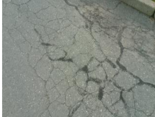
Worn Asphalt Parking Lot Pavement
