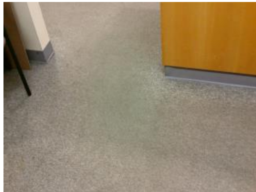
Worn Carpet At Main Office
