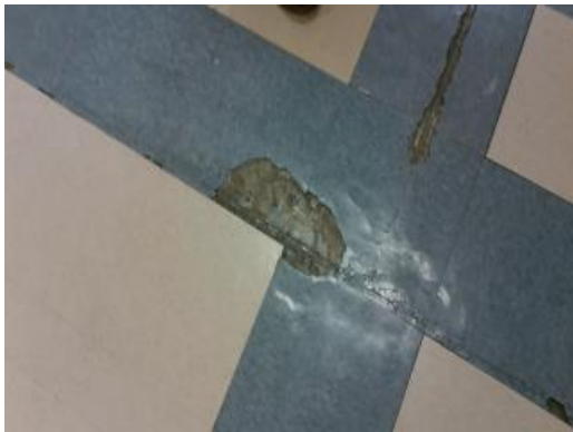
Cracked Flooring at Hallway Between Lockers
