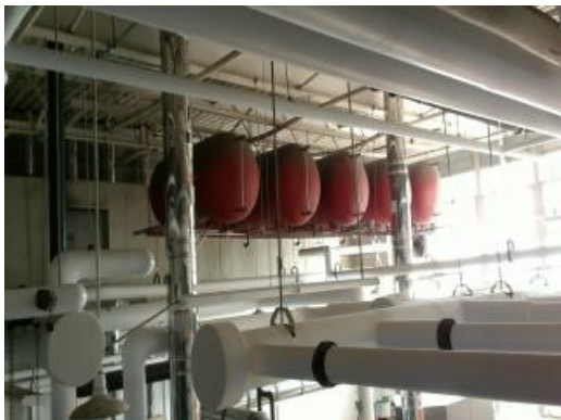
Hot Water Expansion tanks
