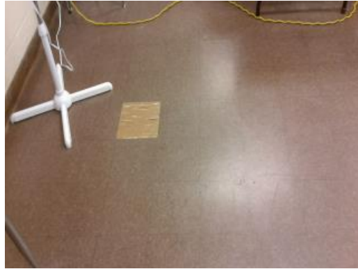
Worn Vinyl Flooring
