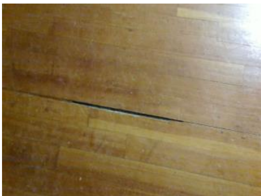
Worn Stage Flooring
