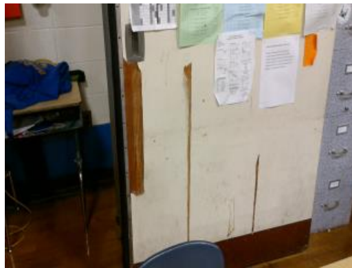
Damaged Moveable Gym Partition
