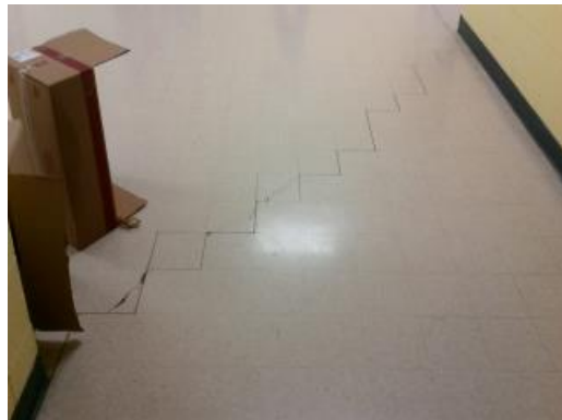
Cracked Flooring Outside of Cafeteria
