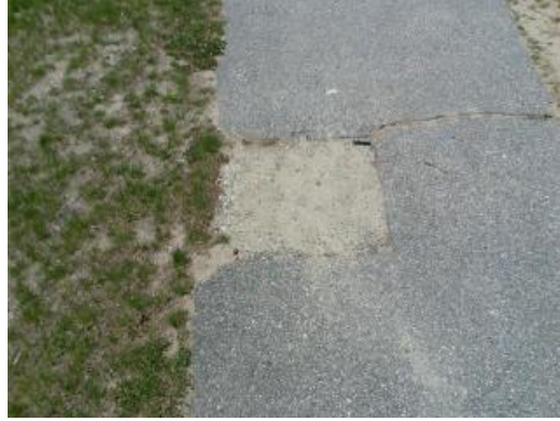
Asphalt Sidewalk Facing Park
