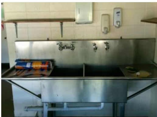
Sink in Room 164
