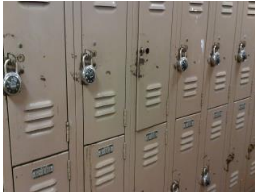
Corroded Lockers at Girls Locker Room
