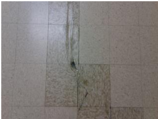
Cracked Flooring Outside Wood Shop
