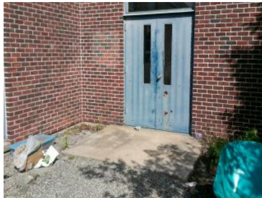
Corroding Exterior Door at Courtyard
