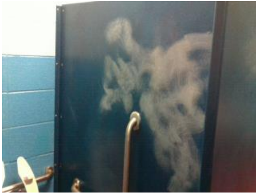
Damaged Toilet Partitions
