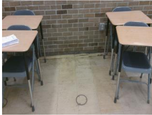
Settlement At Vocational Building
