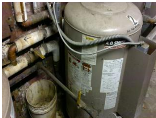
Failed Water Heater
