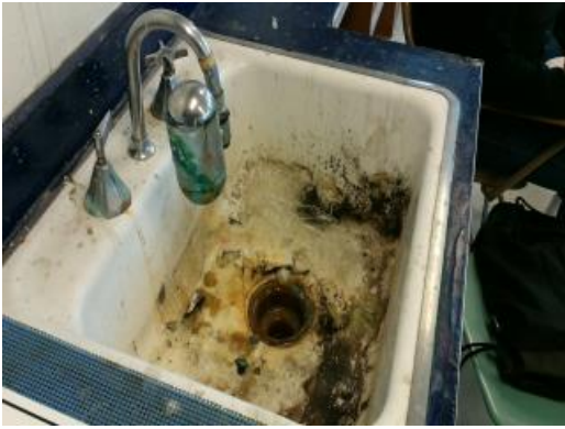
Corroded Custodial Sink
