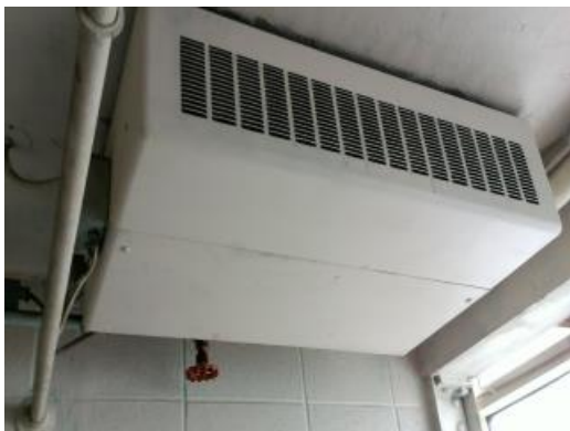
Ceiling Unit Heater
