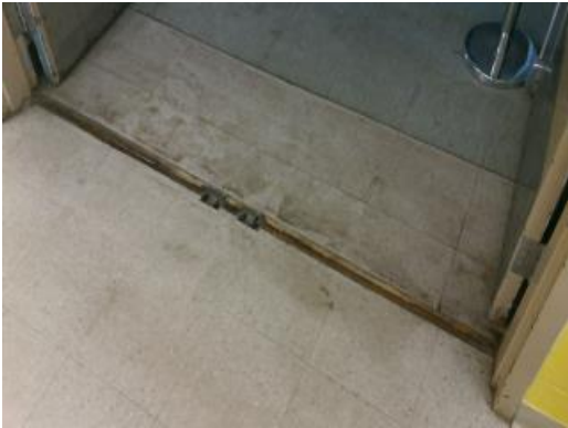
Worn VCT At Threshold
