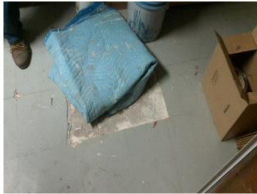
Chipped And Missing VCT
