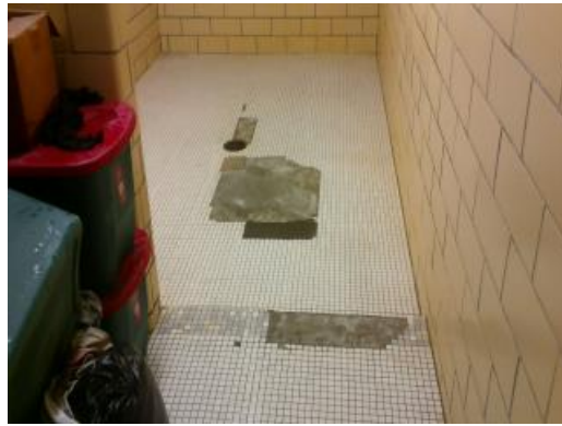
Damaged Ceramic Tile Flooring
