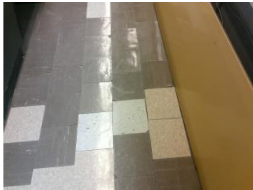
Worn And Lifting VCT Flooring
