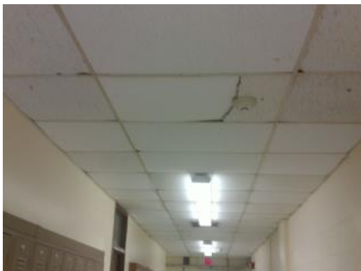
Broken Ceiling Tile
