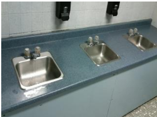
Typical Restroom Lavatories
