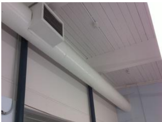
Ductwork For Exhaust
