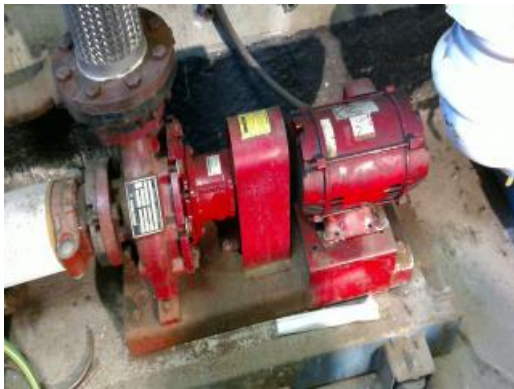
Hot Water Distribution Pump
