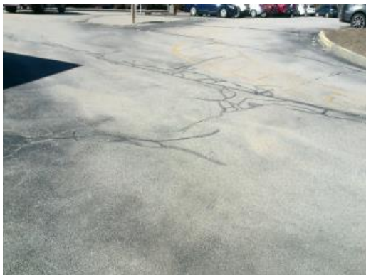
Cracked Asphalt Paving
