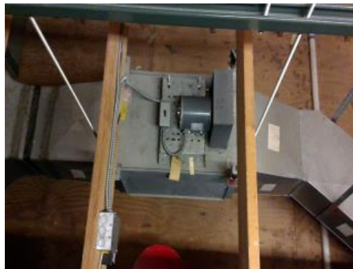
Exhaust System Ventilator For New Wing 4X
