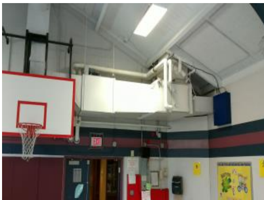
AHU In Gymnasium
