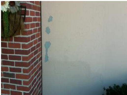
Chipped EIFS Wall
