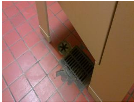
Broken Quarry Tile Flooring
