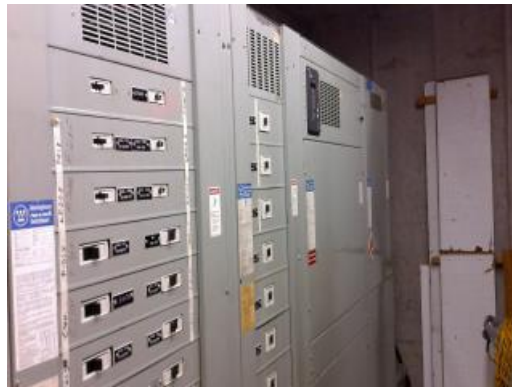
Main Electrical Service
