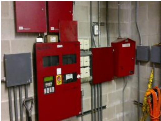
Fire Alarm Panel
