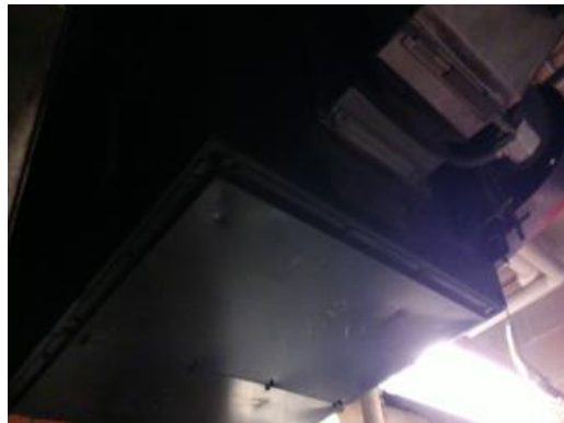
Make-up Air Unit
