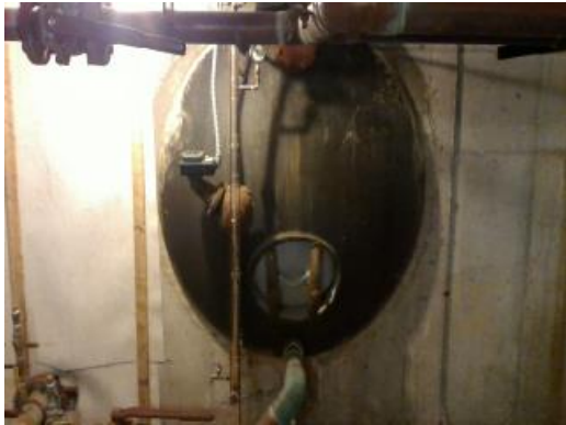
Building 04 - Domestic Water Storage Tank
