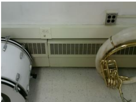
Main Building - Radiant Baseboards
