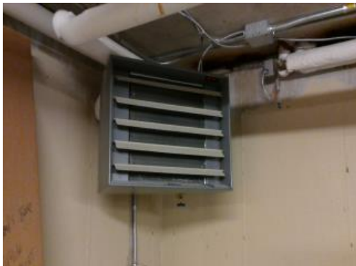
Building 02 - Hot Water Unit Heater
