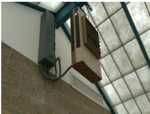
Main Building - Electric Unit Heater
