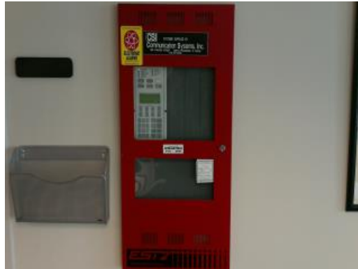
Building 02 - Electronic Alarm System
