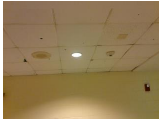
Main Building - Damaged Acoustical Ceiling Tiles
