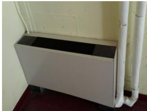
Main Building - Classroom Unit Heater
