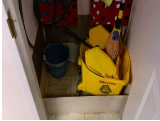
Building 02 - Mop Sink
