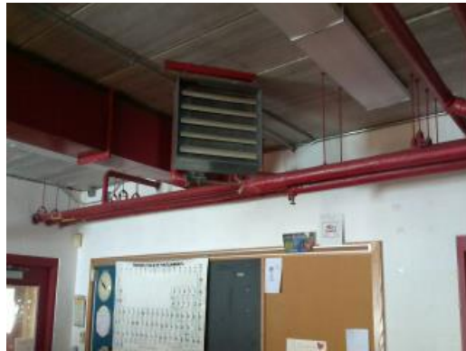
Main Building - Unit Heater
