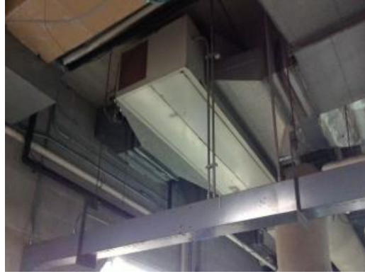
Main Building - Ducted Ceiling Hung Unit Heater
