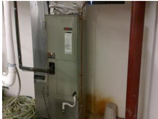
Building 02 - Air Handling Unit
