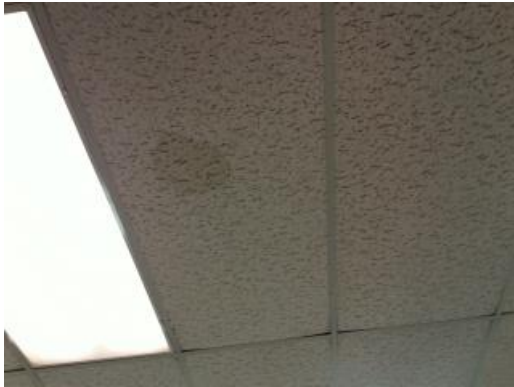
Stained And Sagging Ceiling Tiles
