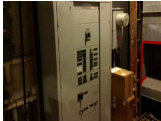
Aged Distribution Panel
