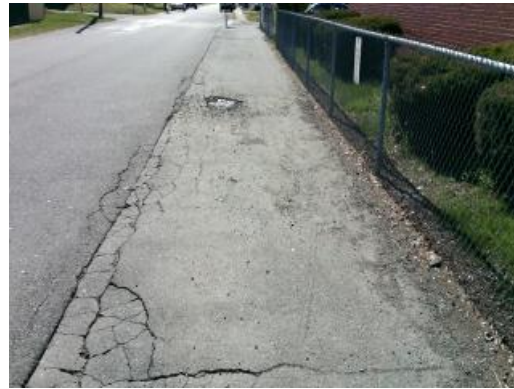
Sidewalk Cracks And Potholes
