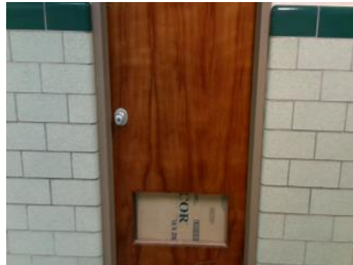
Aged Interior Door With Non-Compliant Hardware
