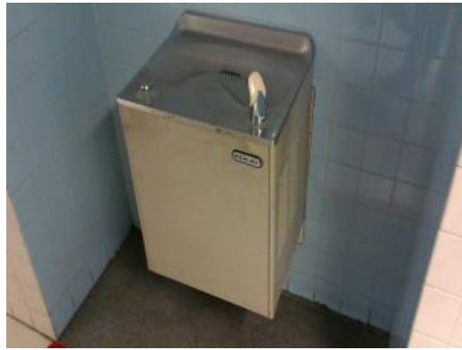
Aged Refrigerated Drinking Fountain
