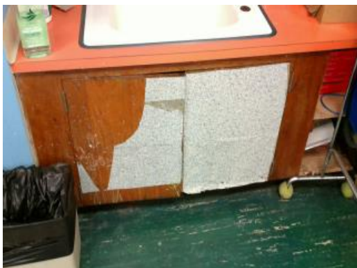
Damaged Original Cabinetry
