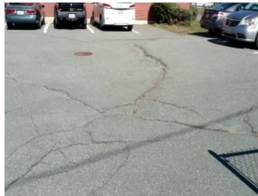
Cracked Asphalt Parking Lot
