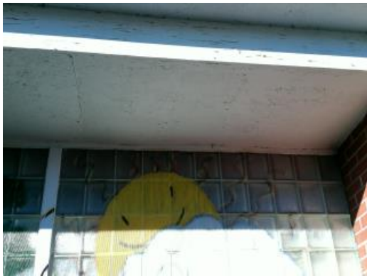
Peeling Paint At Soffit
