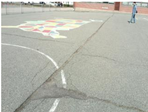
Cracks in Play Area Asphalt
