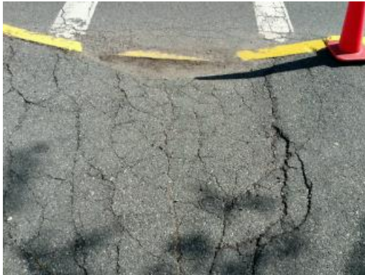
Alligatoring Asphalt Walkway
