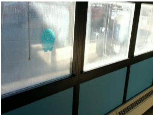
Damaged Window Panes
