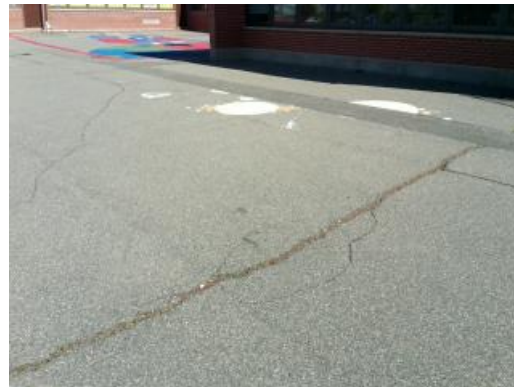
Cracks In Play Area Asphalt
