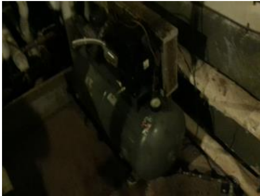
Aged Air Compressor
