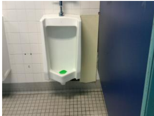
Ceramic Tiles Missing From Restroom Wall
