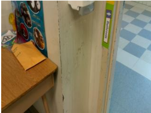
Chipped And Worn Interior Wall Paint
