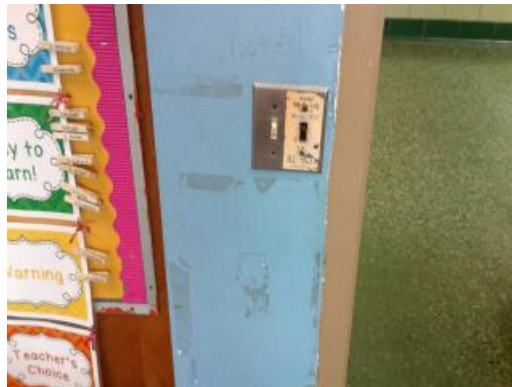
Chipped And Worn Interior Wall Paint
