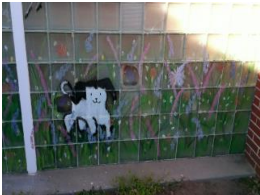
Damaged Glass Block
