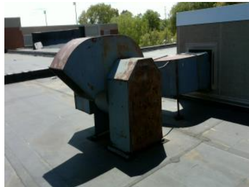
Roof mounted make-up air unit
