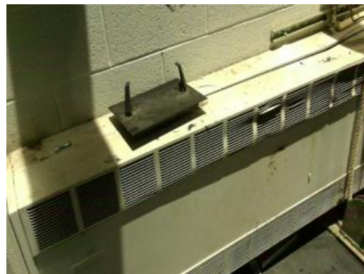
Auditorium Heating Unit
