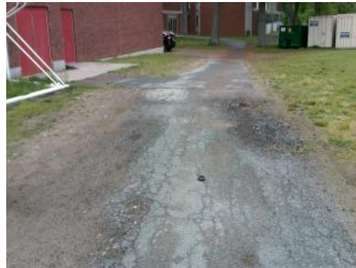
Damaged Asphalt Roadway
