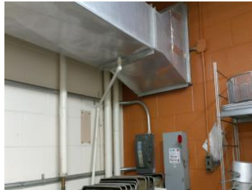
Kitchen Exhaust Fan and Switch
