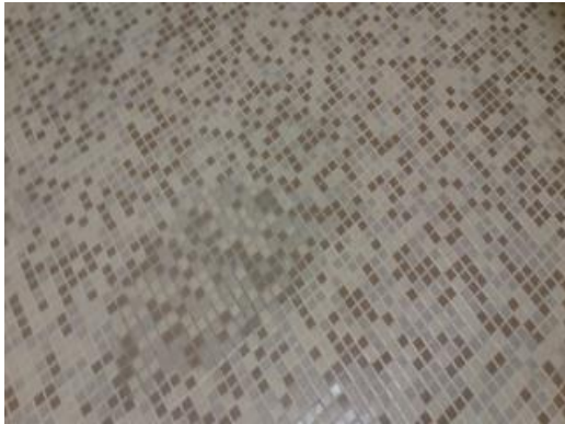
Worn Tile Flooring
