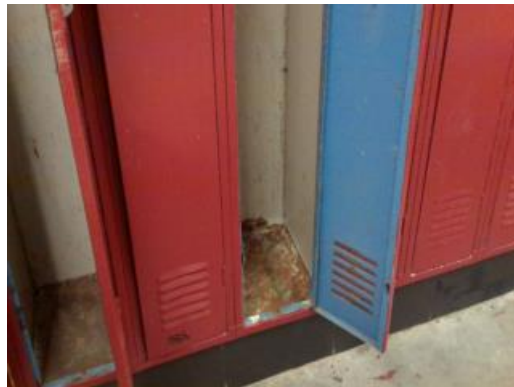
Corroded Locker at Boy's Locker Room
