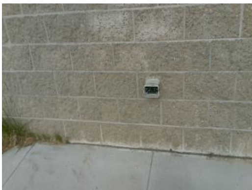
Exterior GFCI Receptacle
