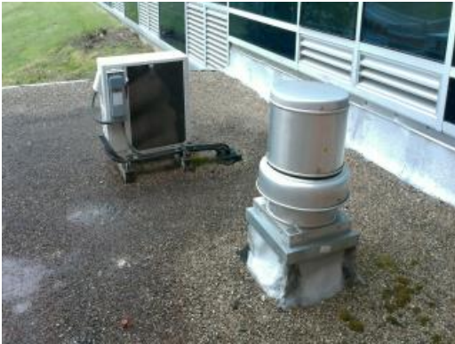
Condensing Unit And Exhaust Fan
