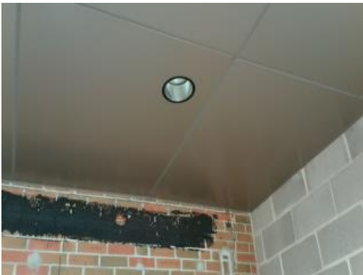
Canopy Mounted Fixture
