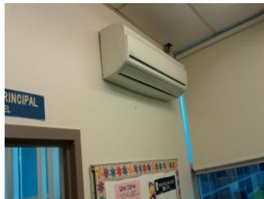
Ductless Split System
