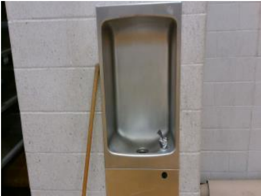
Typical Drinking Fountain
