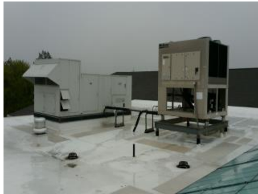
Air Handling Unit
