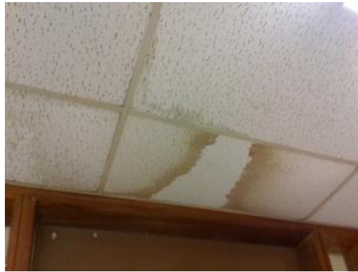
Stained Ceiling Tiles
