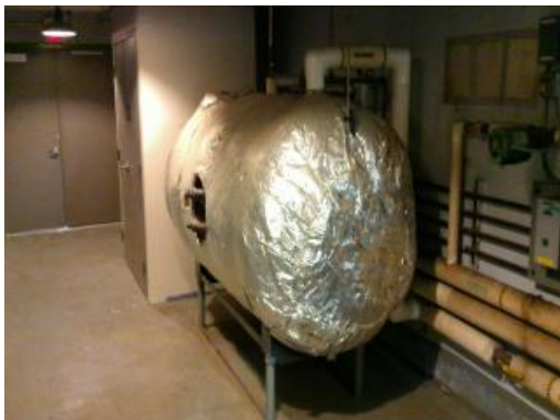
Hot Water Storage Tank
