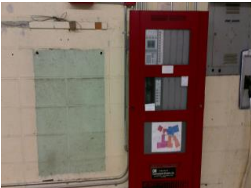
Fire Alarm Panel
