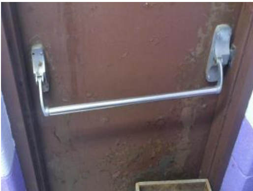
Corroded Exterior Metal Door
