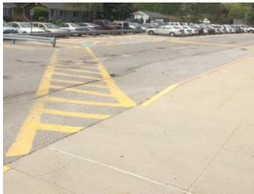
Asphalt Parking Pot Holes
