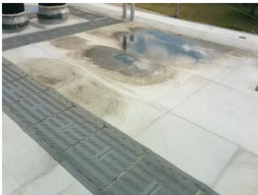
Ponding On Roof
