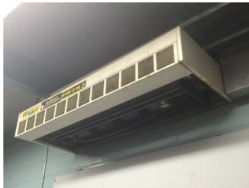
Aged Heating Unit
