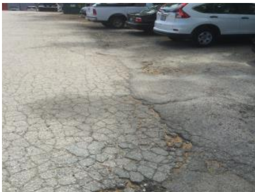
Alligatoring Parking Lot
