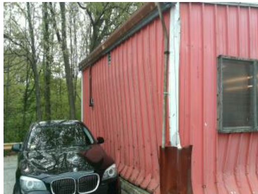
Damaged Metal Facade
