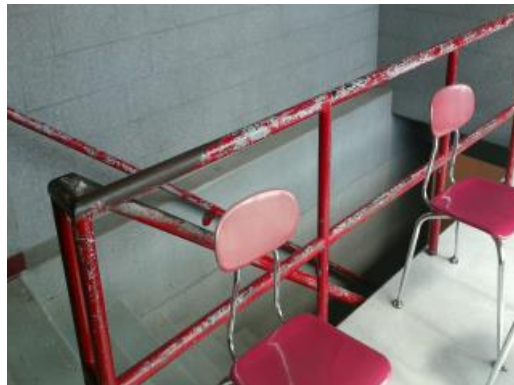
Chipped Handrail Paint
