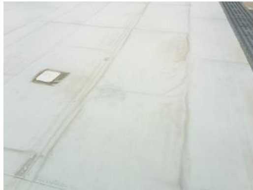
Weathered Gym Roofing
