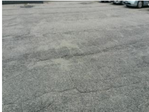
Weathered Roadway Asphalt
