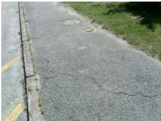
Cracked And Weathered Sidewalk
