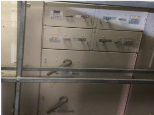
Aged Electrical Distribution
