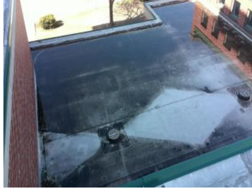
Ponding On Roof
