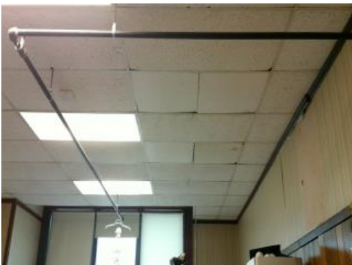
Art Director's Office Ceiling Tiles
