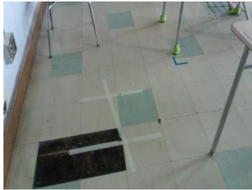
Damaged VCT In Classrooms
