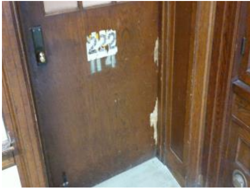
Damaged Interior Wood Door
