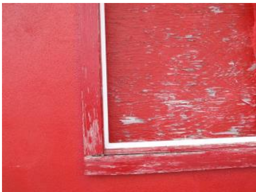
Worn Exterior Paint
