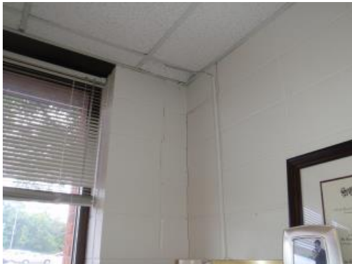
CMU Wall Crack
