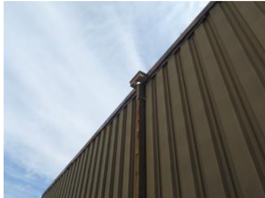
Rusted And Deteriorated Downspout
