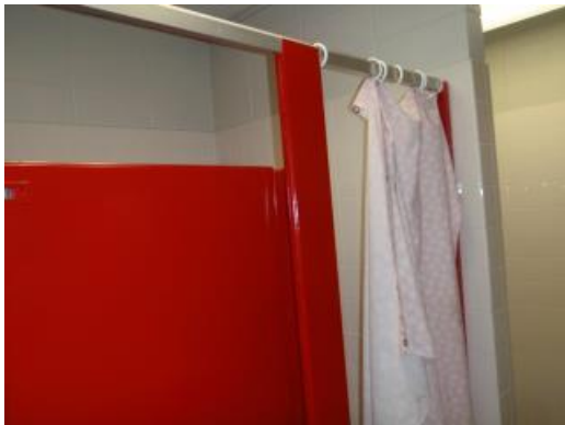
Missing Partition Door
