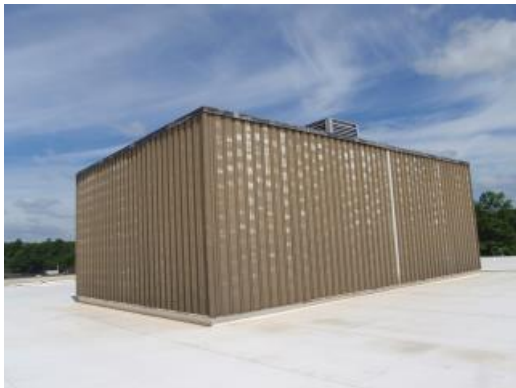
Rooftop Mechanical Enclosure
