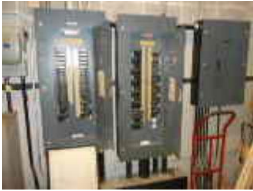
Carpentry Shop Panelboards
