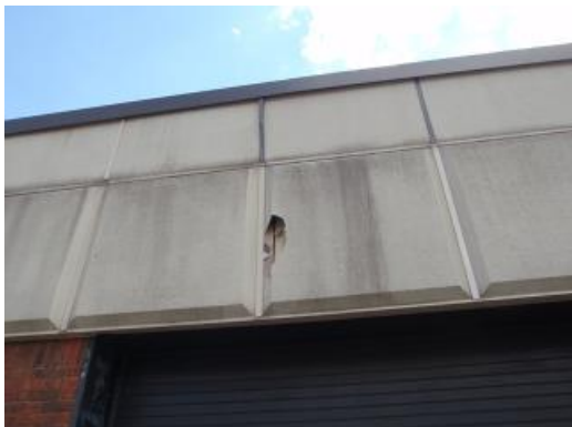
Damaged And Stained Exterior Roof Trim
