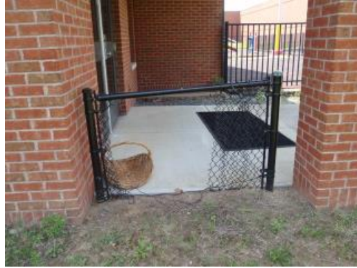
Damaged Chain Link
