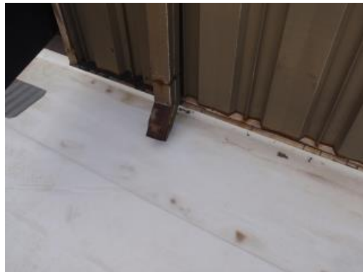
Missing Splash Block
