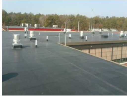
Roof Exhaust Fans
