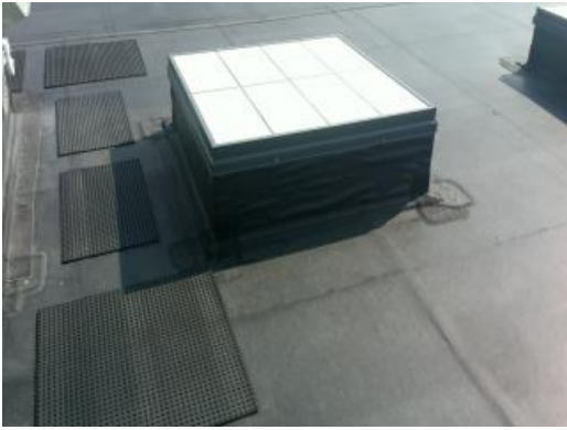
Ripples In The Membrane Flashing
