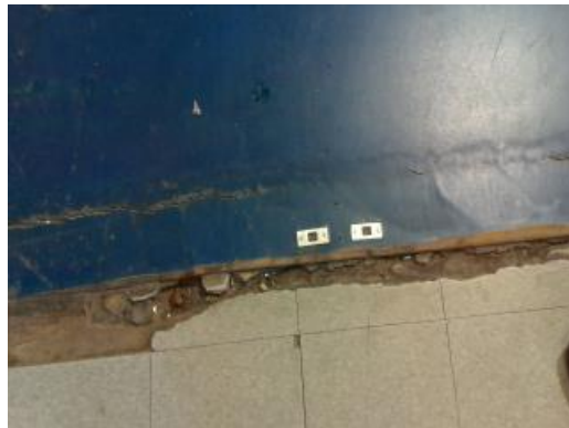
Damaged And Missing VCT
