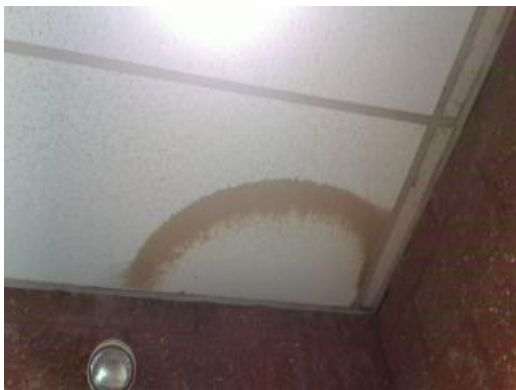
Water Damaged Ceiling Tile
