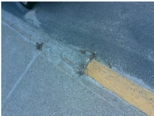
Faded Paint On Curbs
