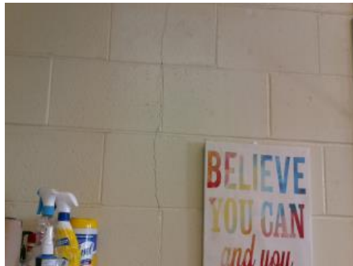
Cracking In CMU
