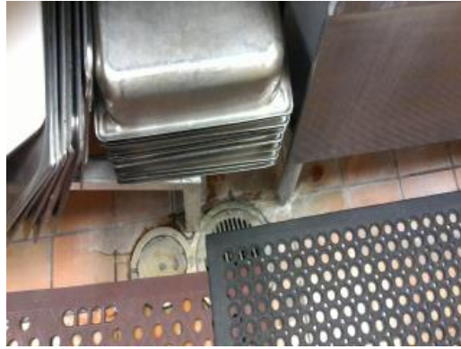
Floor Drain in Kitchen
