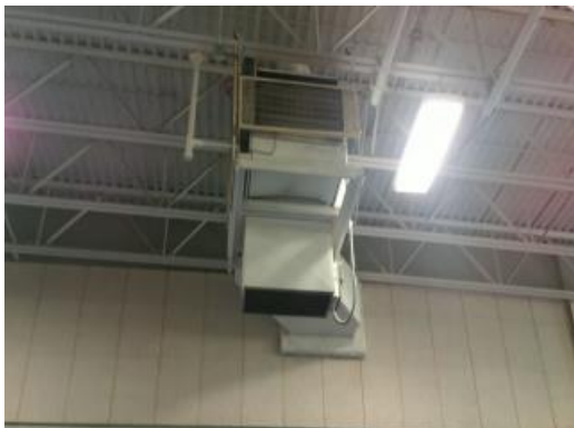
Rusted Make Up Air Unit
