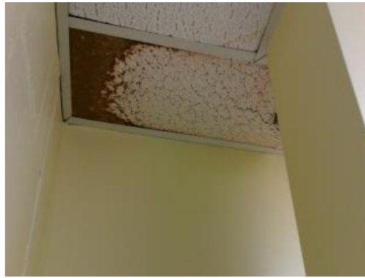
Water Damaged Ceiling Tile
