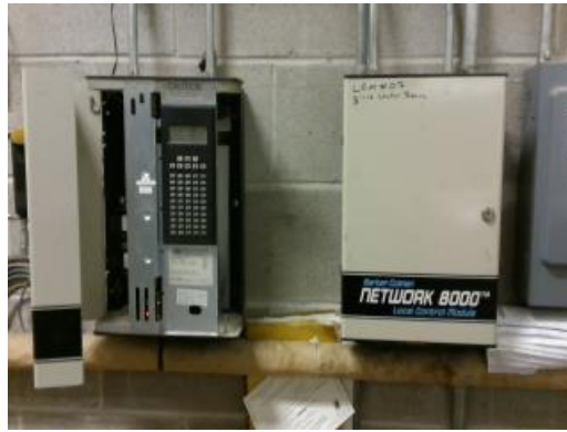
HVAC Controls For New Units
