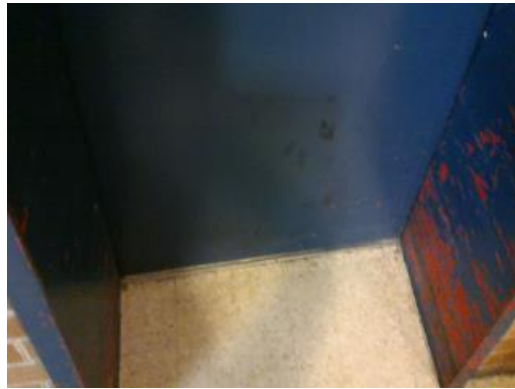
Non-Compliant Elevator Door
