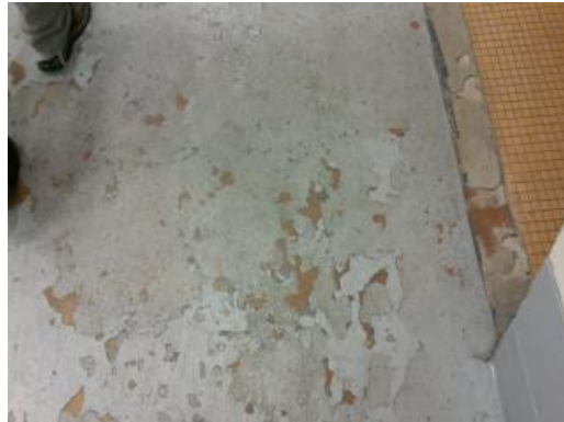
Worn Concrete Floor
