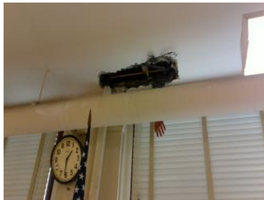
Hole In Gypsum Board Ceiling
