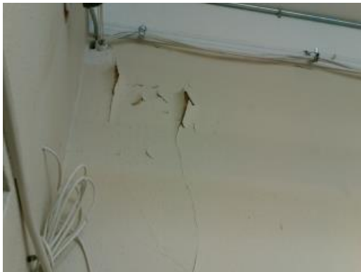
Cracking And Peeling Painted Walls
