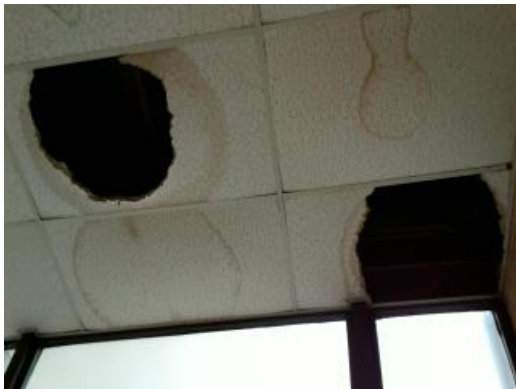
Stained And Broken Ceiling Tiles
