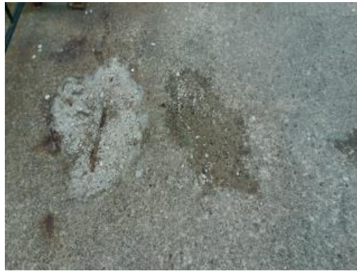
Worn Concrete At Main Entrance Stairs
