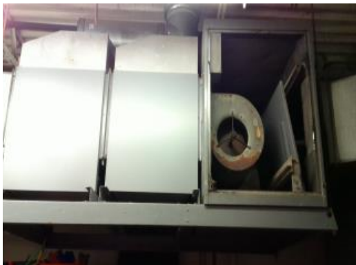
Rusted Make-Up Air Unit
