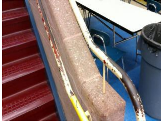
Worn Cafeteria Handrail
