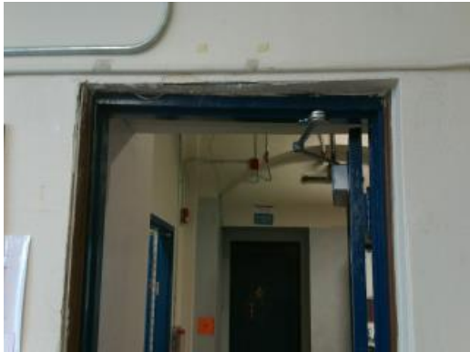
Door Frame Separated From Wall
