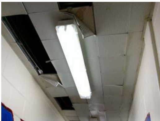
Failing Adhered Ceiling Tiles
