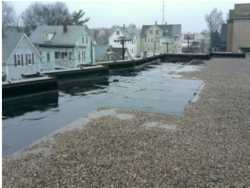
Ponding On Roof
