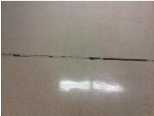
Cracks In VCT
