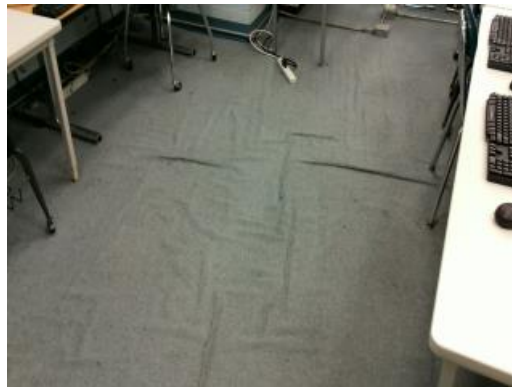
Buckled Carpet In Library
