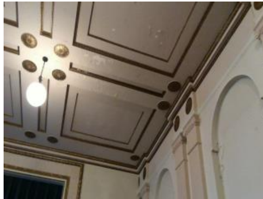
Cracked Ceiling In Auditorium
