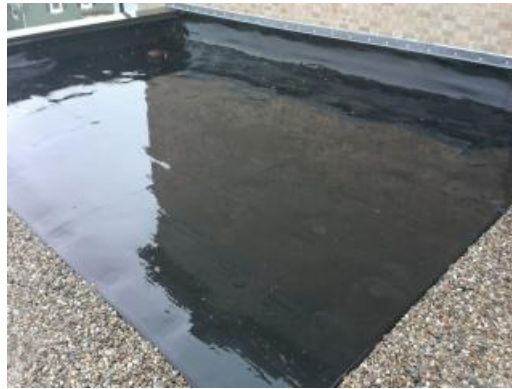
Water Ponding On Roof
