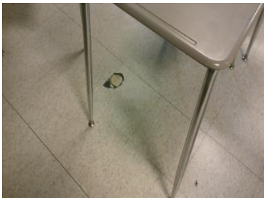
Chipped And Separating VCT
