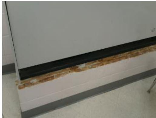
Damaged Cabinet Unit Ventilator
