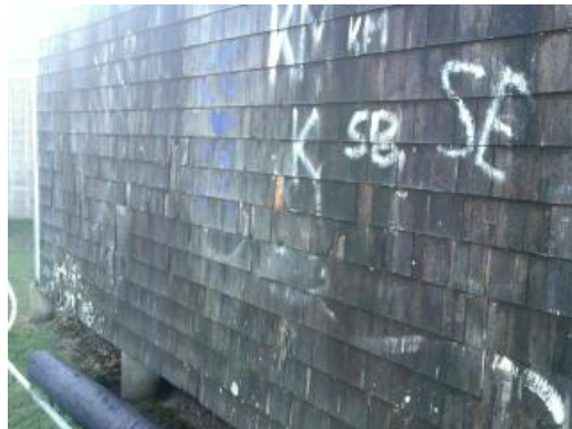
Weathered And Vandalized Wood Siding
