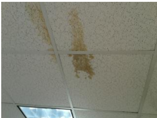
Stained Ceiling Tiles
