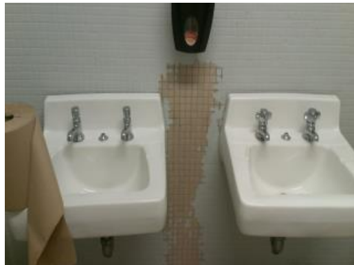
Peeling Wall Paint
