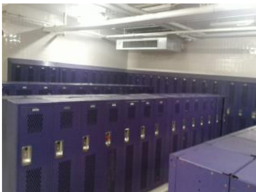
Damaged Locker Room Lockers
