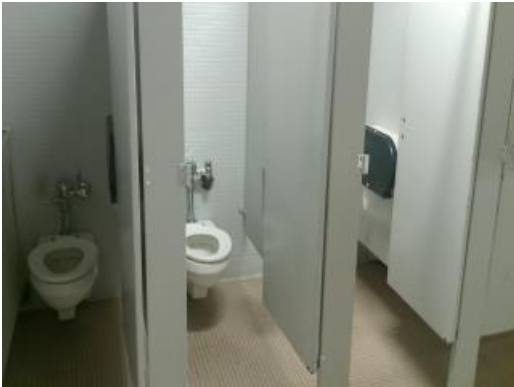
Non-Compliant Toilet Stalls
