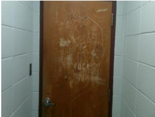
Vandalized Interior Door
