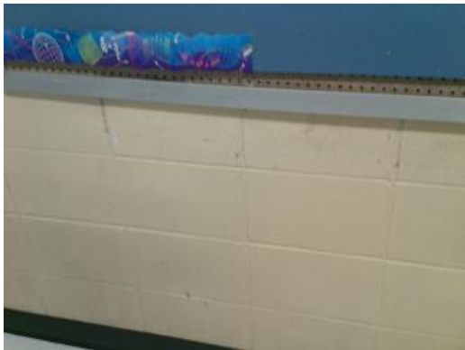
Worn CMU Wall
