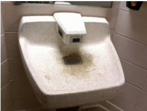
Worn Bathroom Sink
