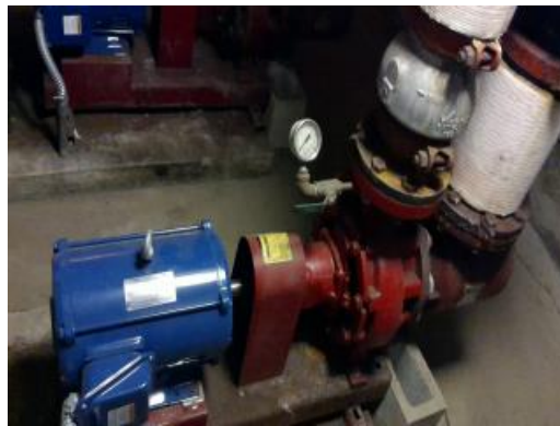
10 HP Circulating Pump
