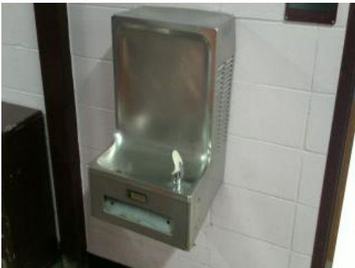
Damaged Drinking Fountain
