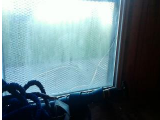
Cracked Window At Concessions Building
