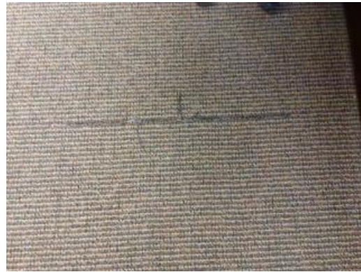
Frayed Carpet In Office
