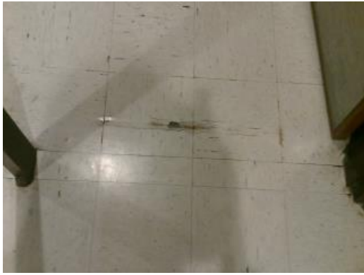
Cracked VCT Flooring
