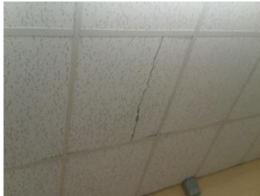
Broken Ceiling Tile
