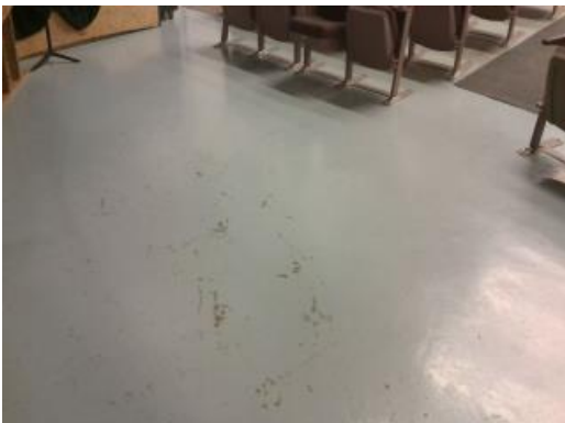
Chipped Paint On Auditorium Floor
