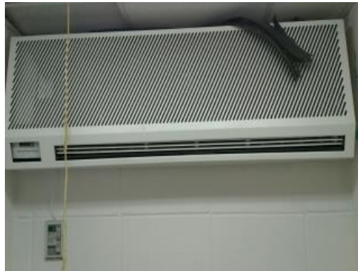
Aged Fan Coil Unit
