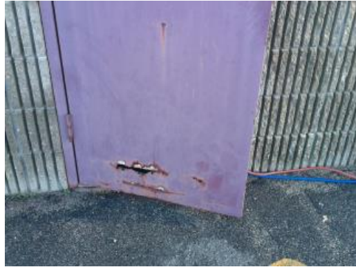
Rusted Exterior Door
