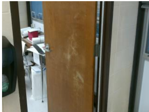
Worn Wood Door
