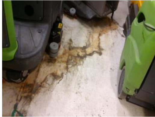
Stained And Broken VCT
