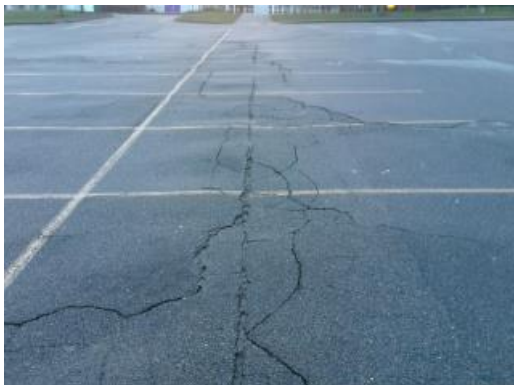
Cracked Parking Lot Pavement
