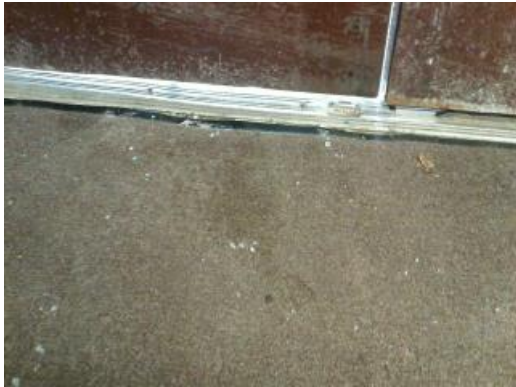
Exterior Door Rusted At Bottom
