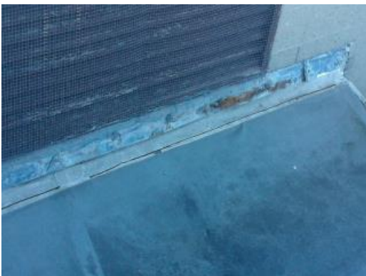
Corroded Metal At Termination Wall
