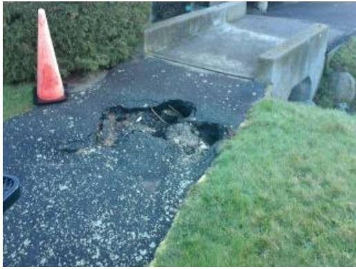
Pot Hole In Asphalt Walkway
