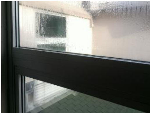
Poor Seals At Window
