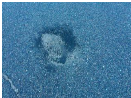
Pot Hole In Parking Lot
