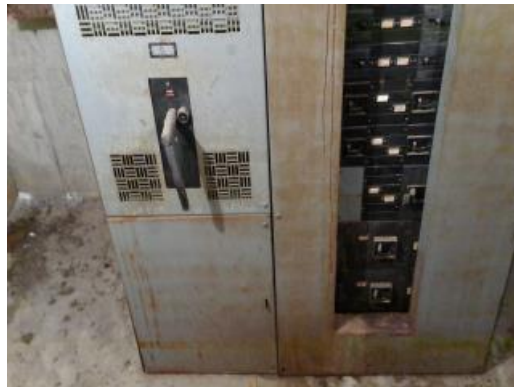
Main Building - Distribution Panel
