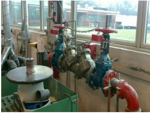
Main Building - Backflow Preventer
