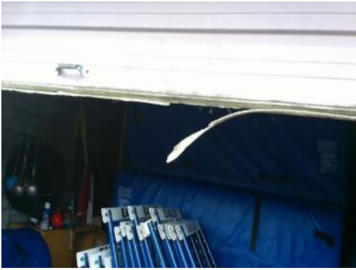
Building 03 - Soffit Damage
