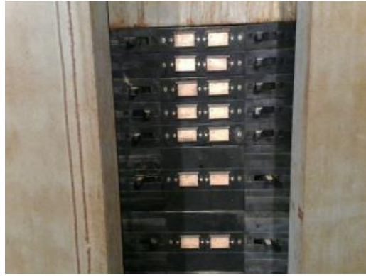
Main Building - Electric Panel
