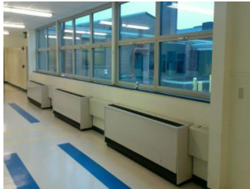
Main Building - Unit Ventilators
