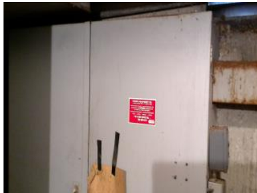
Main Building - Transfer Switch
