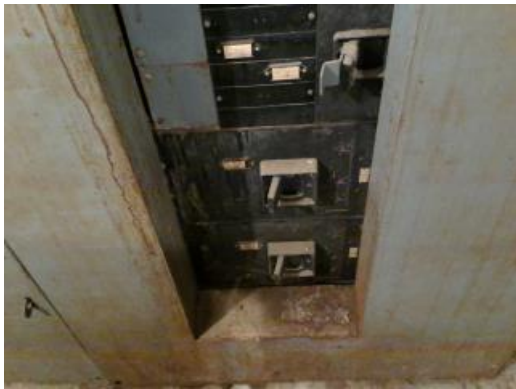
Main Building - Electric Panel
