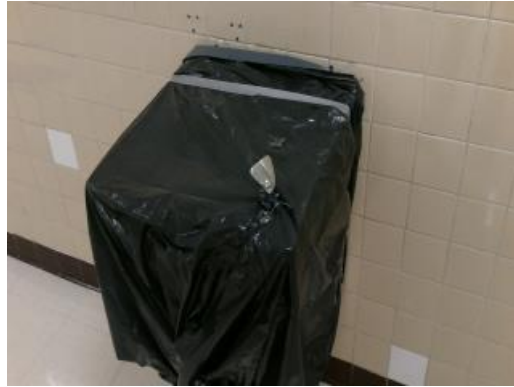
Main Building - Broken Water Cooler
