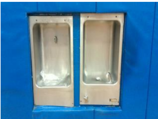
Main Building - Water Cooler
