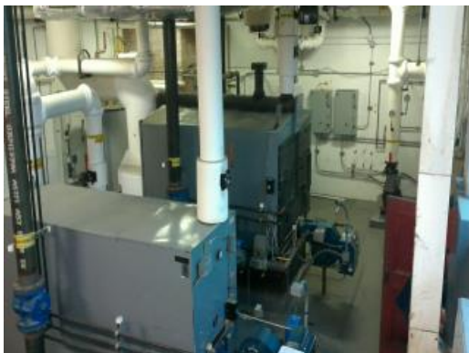
Main Building - Mechanical Room
