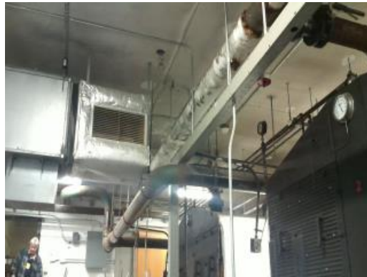
Main Building - Damaged Insulation
