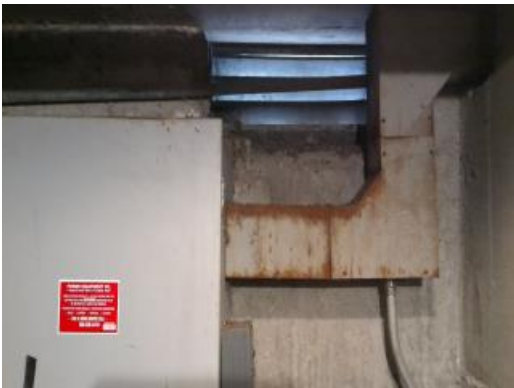
Main Building - Transfer Switch
