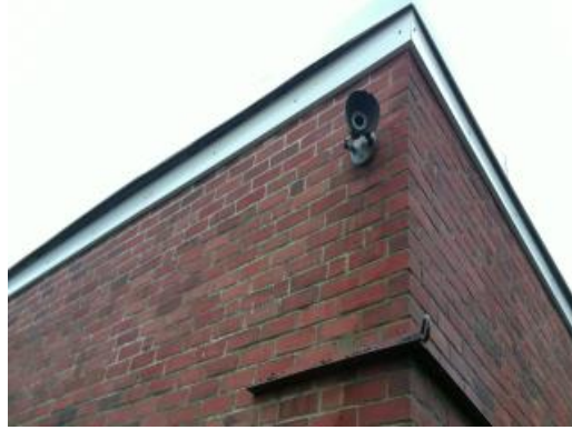
Main Building - Damaged Building Mounted Lighting
