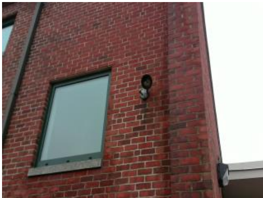
Main Building - Damaged Building Mounted Lighting
