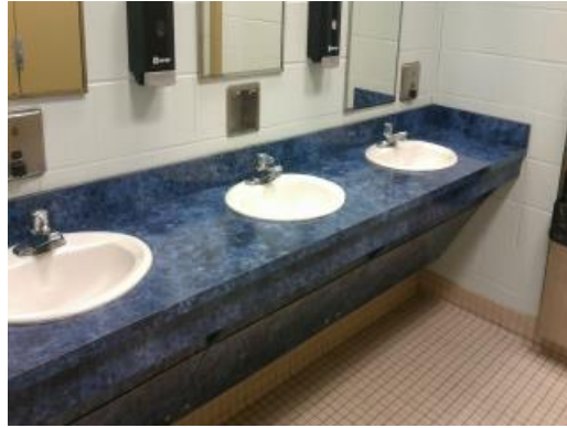
Main Building - Restroom Sinks
