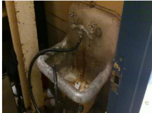
Main Building - Corroded Janitor Sink
