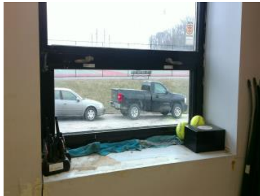
Evidence Of Water Damage At Window
