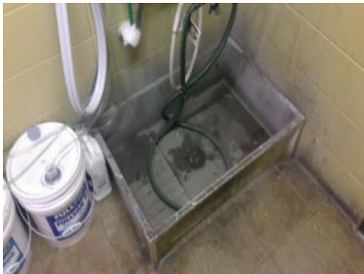
Stained Mop Sink
