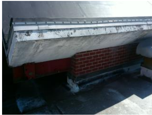
Damaged Soffit At Library
