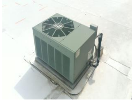
Condenser With Collapsed Coils
