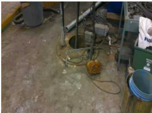
Failing Sump Pump
