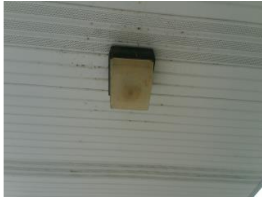
Original Canopy Lighting
