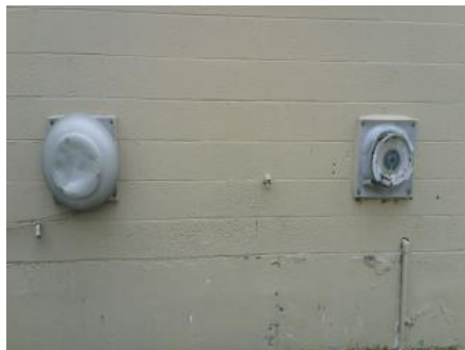
Septic House Exhaust Fans
