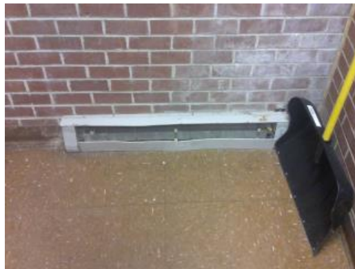
Original Radiant Heaters
