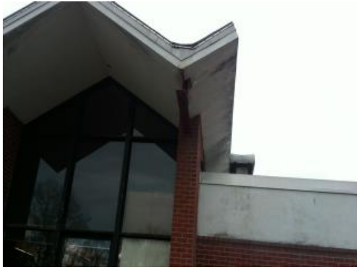
Damaged Library Roof Soffit
