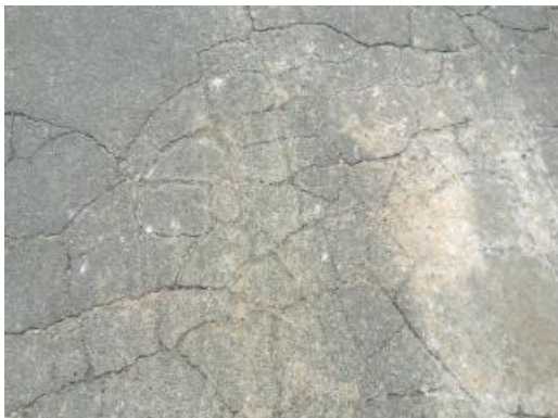
Alligatoring Parking Lot Pavement
