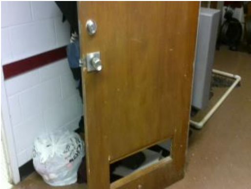
Chipped And Worn Wood Door
