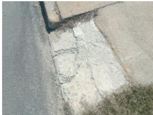
Cracked Concrete Walkway
