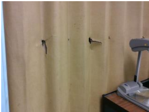
Typical Stained And Torn Partition
