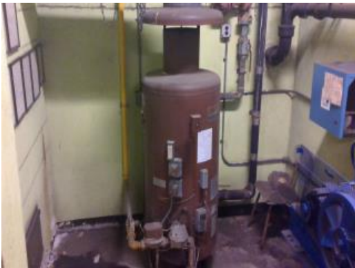
Aged Boiler For Hot Water
