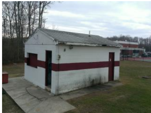
Building 3 Decaying Roof
