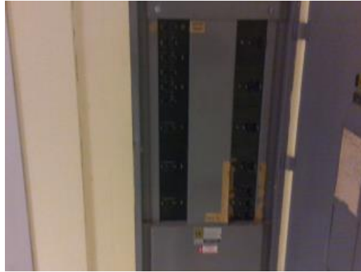
225A Panel With Corroded Connections
