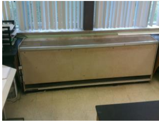
Aged Heating Unit
