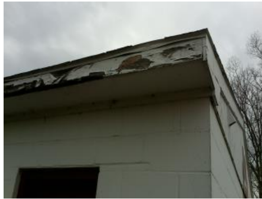
Building 3 Damaged Roof Fascia
