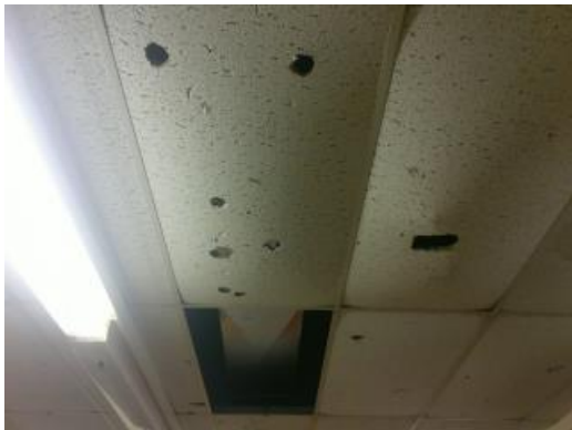
Damaged And Missing Ceiling Tiles
