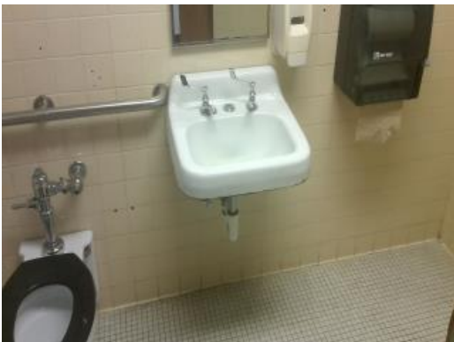
Maintenance Shed Restroom Fixtures
