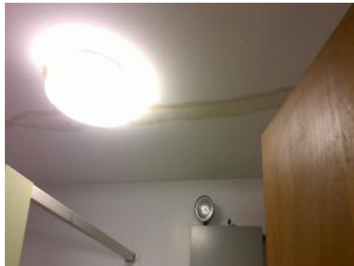
Stained Gypsum Ceiling
