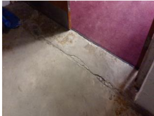
Cracked Concrete Flooring
