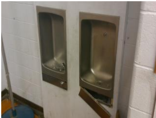
Damaged Drinking Fountain
