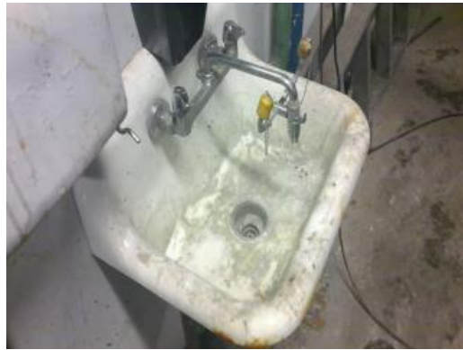
Stained And Corroded Service Sink
