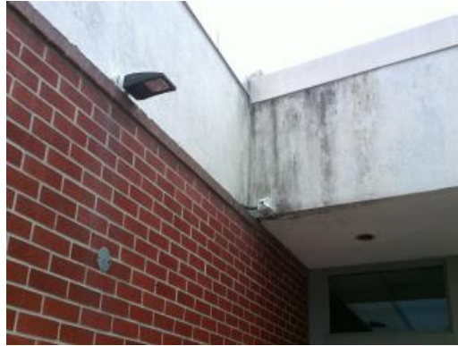
Stained And Weathered Stucco
