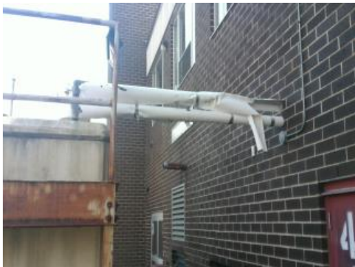
Damaged Insulation At Fuel Tank
