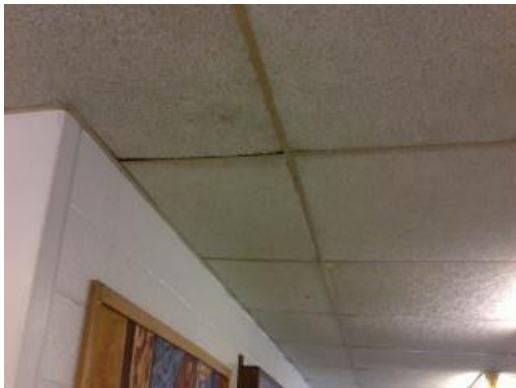
Stained Ceiling Grid
