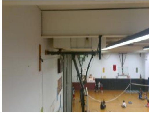
Non-Functional Make-up Air Unit
