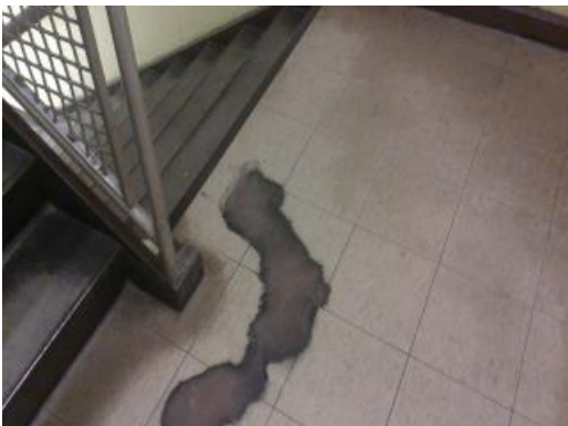
Worn VCT Flooring
