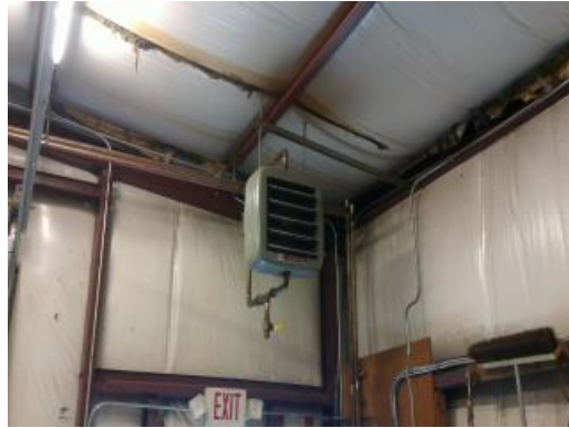
Maintenance Shed Unit Heater
