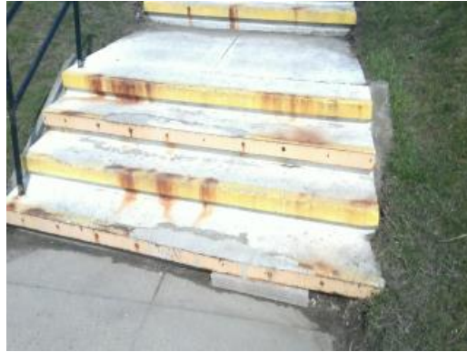
Concrete Stairs Settling
