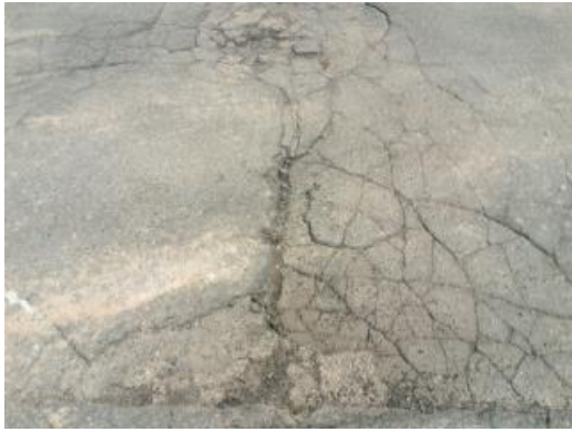
Cracked Roadway Asphalt
