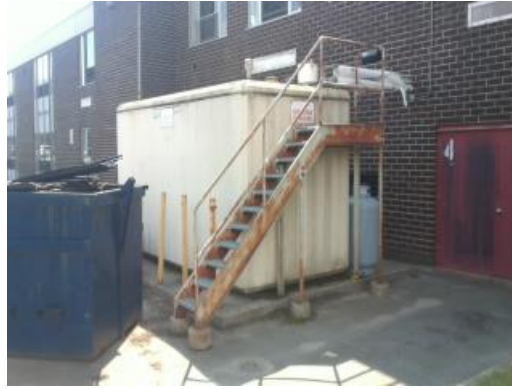
Fuel Storage Tank
