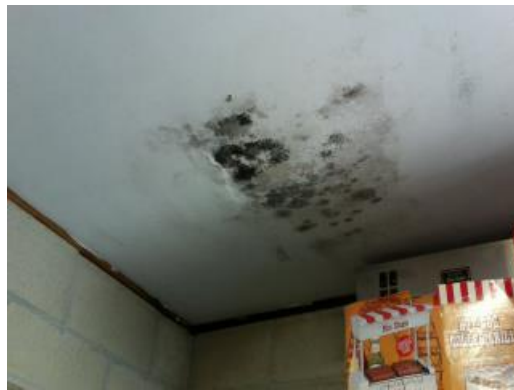
Building 3 Stained Concession Ceiling
