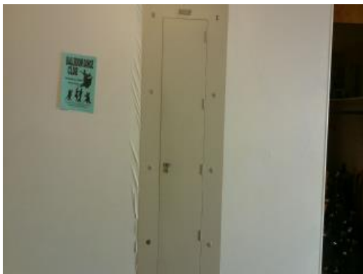
Peeling Wall Covering
