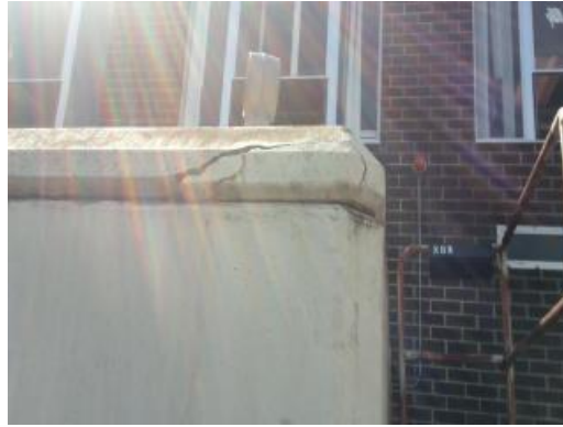
Cracked Concrete On Fuel Tank
