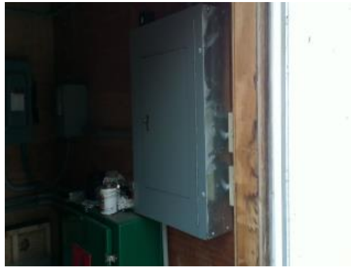
Building 4 Electrical Panel
