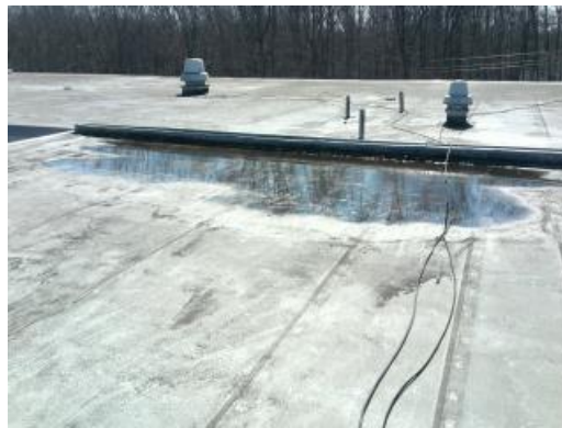
Ponding At Expansion Joint
