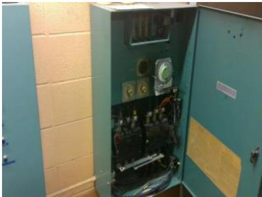
Transfer Switch With Burned Contacts
