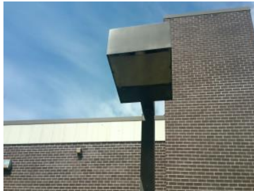
Aged Pole Mounted Lights
