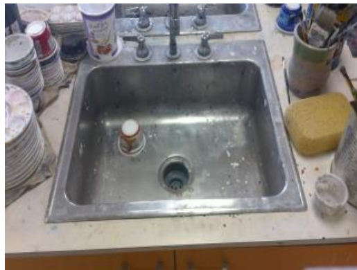
Stained And Worn Classroom Lavatory
