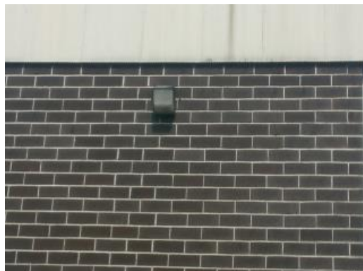
Typical Building Mounted Fixture
