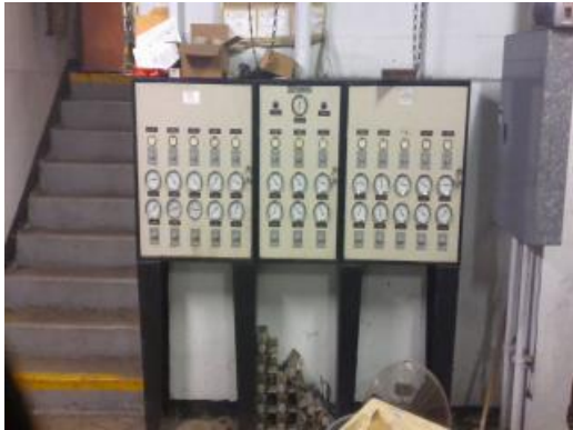
Pneumatic Controls Panel
