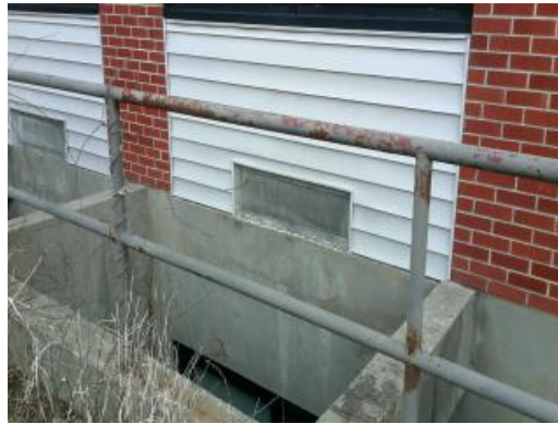
Chipped Paint Window Well Railing
