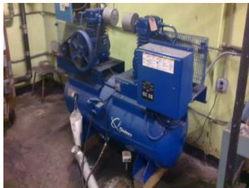
Compressor For Pneumatic Controls
