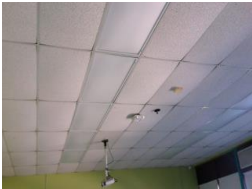
Stained And Sagging Ceiling Tiles
