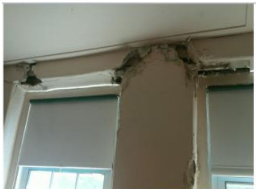
Water Damage At Basement Windows
