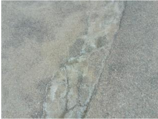
Cracked Asphalt Paving
