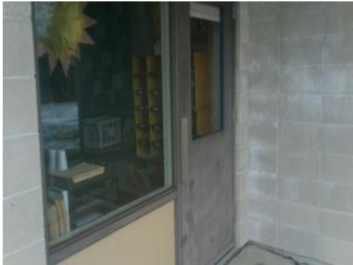
Faded And Worn Exterior Door
