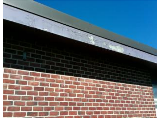
Peeling Exterior Paint
