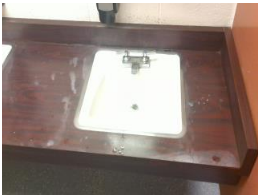
Aged And Stained Restroom Lavatory
