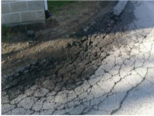
Roadway Alligator Cracking
