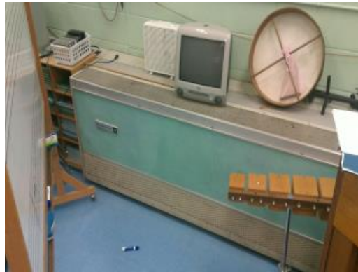
Aged Heating Unit
