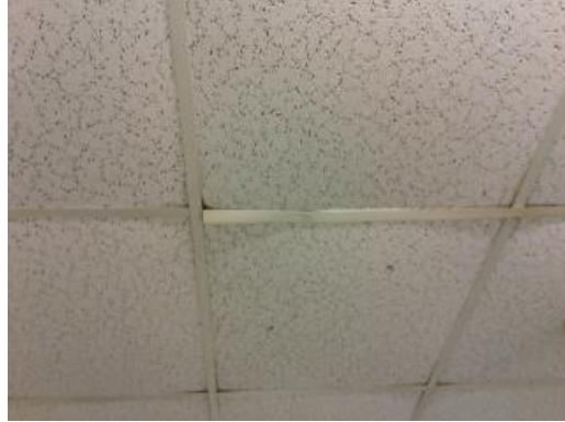
Broken Ceiling Grid
