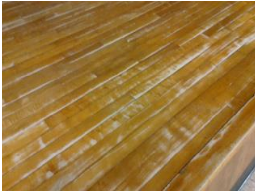
Worn Wood Floor At Stage
