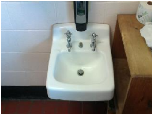
Typical Restroom Lavatory
