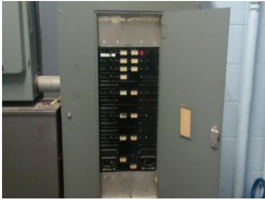
400 Amp Panel With Improper Repairs
