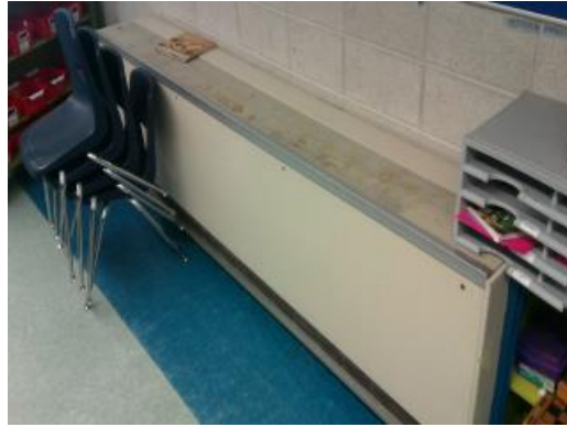
Aged Heating Unit
