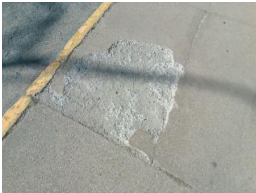
Spalling Concrete Walkway
