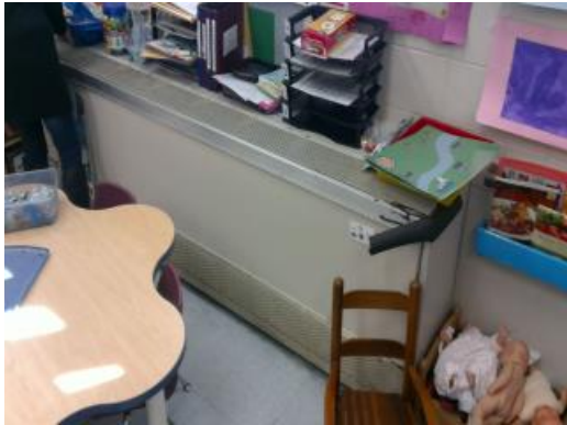
Unit Vent Heater Coils Clogged
