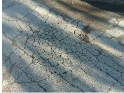
Parking Alligator Cracking
