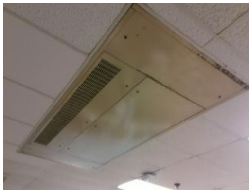
Rusted And Molding Split System
