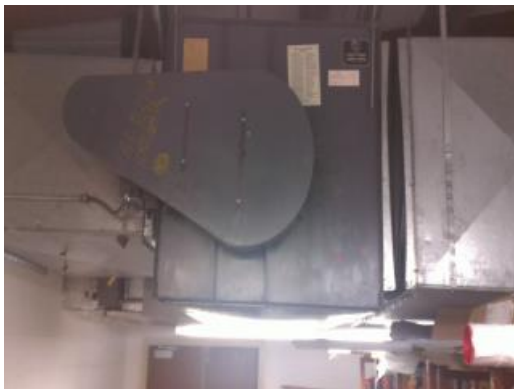
Air Handling Unit
