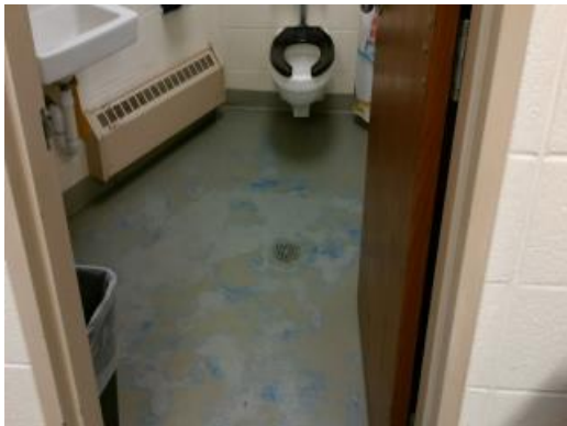
Worn Epoxy At Restroom
