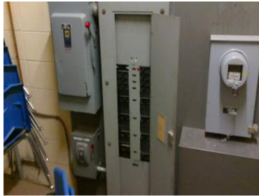
Aged Distribution Panel
