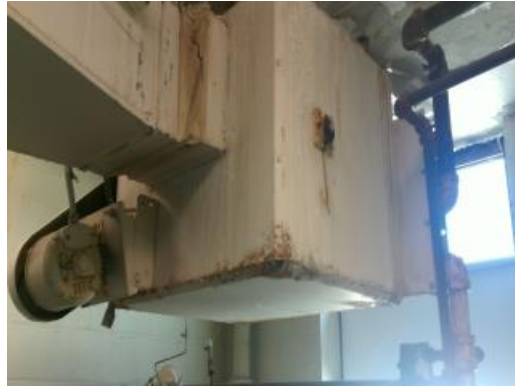
Corroded Make-Up Air Unit
