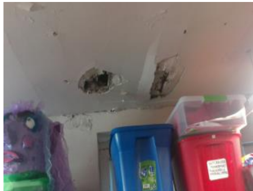
Holes In Gypsum Board Ceiling
