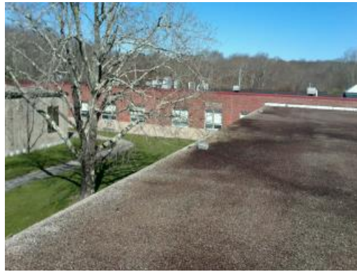
Evidence Of Ponding On Roof
