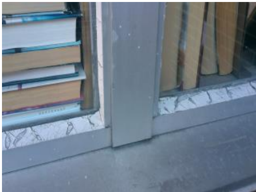
Failed Caulking At Windows
