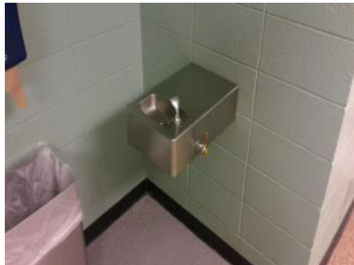
Stained Drinking Fountain
