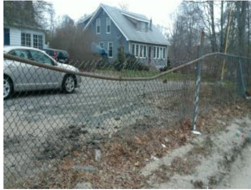
Rusted And Falling Fence
