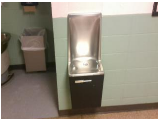
Drinking Fountain With Non-Functional Compressor
