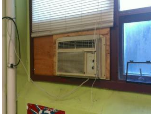
Failing Window Unit
