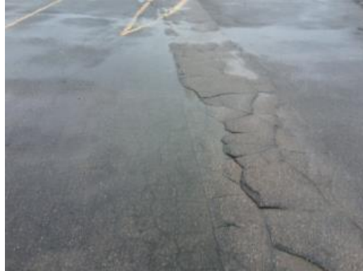
Sinking And Cracking Pavement
