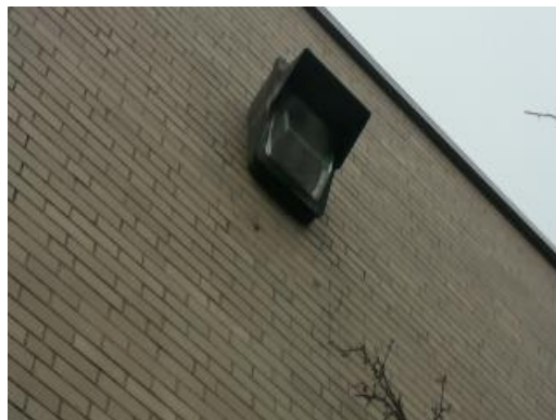
Building Mounted Light
