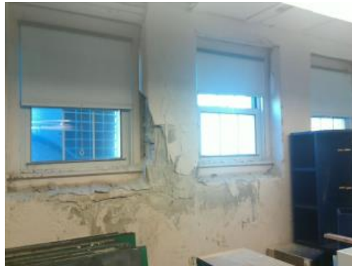
Water Damaged Basement Wall
