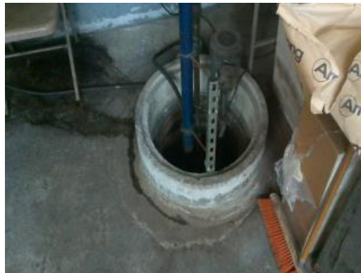
Non-Functional Sump Pump
