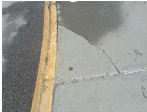
Cracked Concrete Walkway
