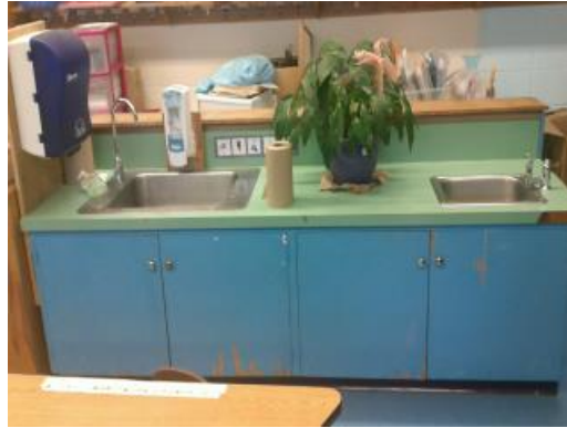
Damaged Classroom Cabinets
