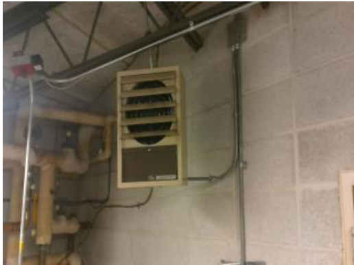
Non-Functional Electric Unit Heater
