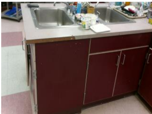
Chipped Art Classroom Cabinetry
