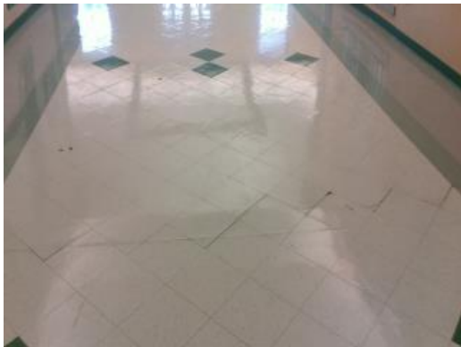
Typical VCT Damage
