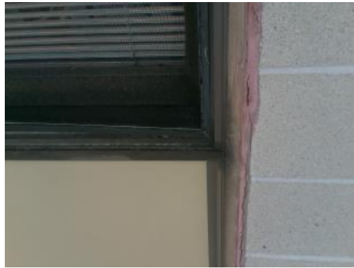
Failed Window Caulking
