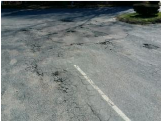
Alligatored And Patched Asphalt Parking
