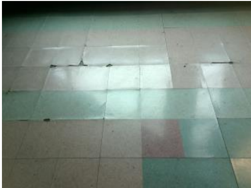
Chipped And Curling VCT
