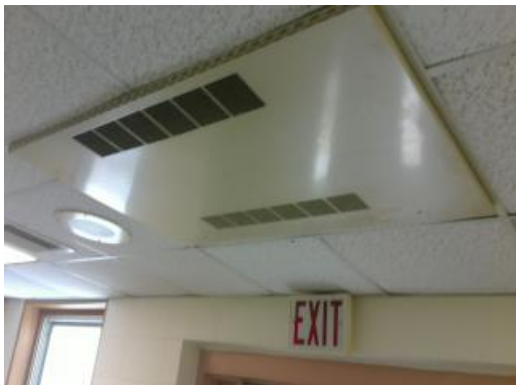
Heating Unit Vent
