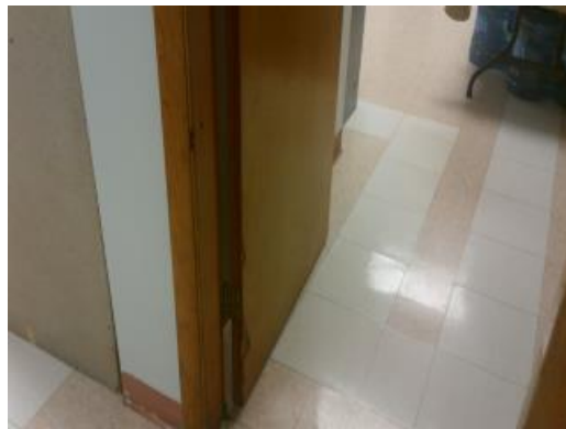
Chipped Laminate Wood Door
