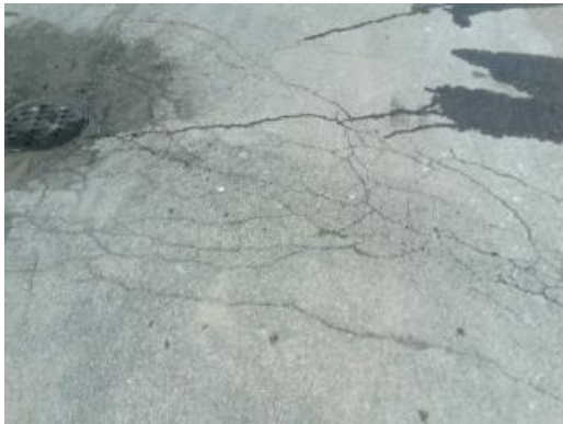
Cracked Parking Lot Asphalt
