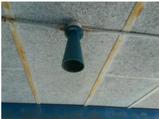
Non-Functional Canopy Light
