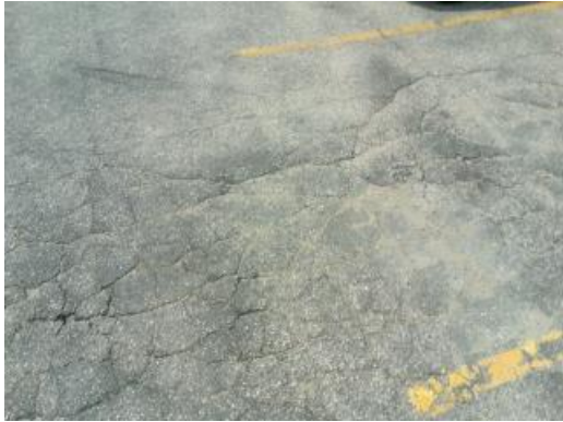
Alligatored Parking Pavement
