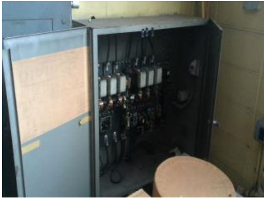
Transfer Switch With Burned Contacts
