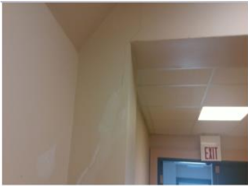
Crack At Stairwell Wall
