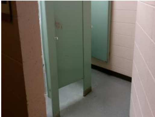
Faculty Restroom With No ADA
