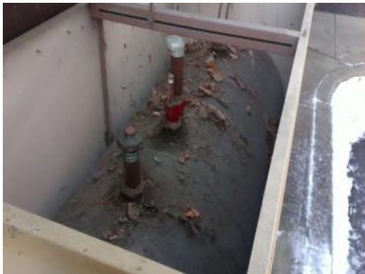
Rusting Fuel Tank
