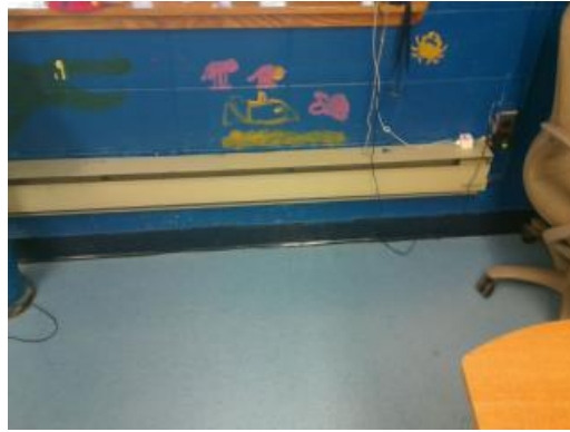
Damaged Radiant Heater
