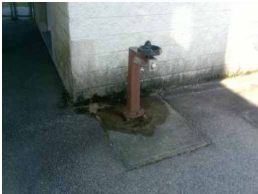
Exterior Drinking Fountain
