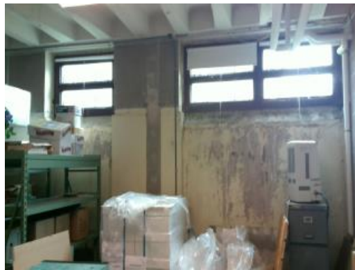
Peeling Paint In Storage
