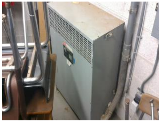
Federal Pacific Transformer
