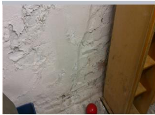
Damaged Basement Wall
