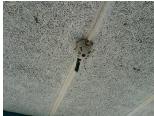
Broken Canopy Light
