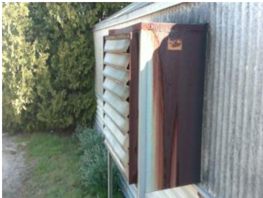
Rusted Wall Exhaust
