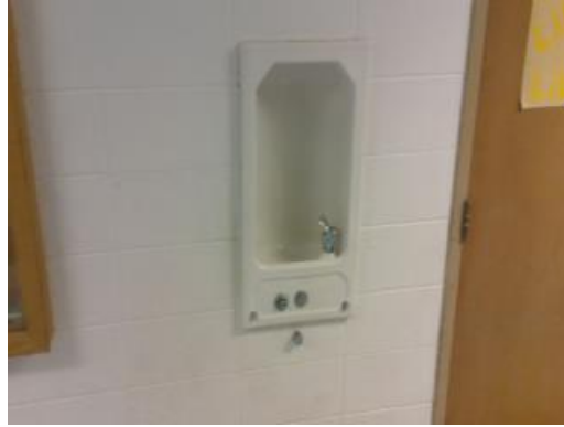
Hallway Drinking Fountain
