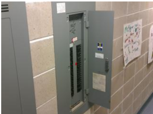
Federal Pacific Panelboard
