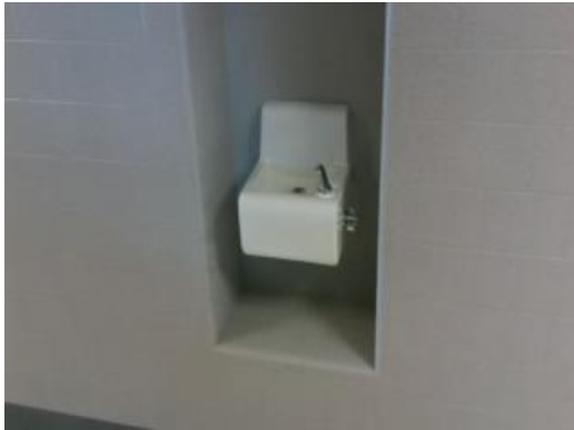
Non-Functional Drinking Fountain
