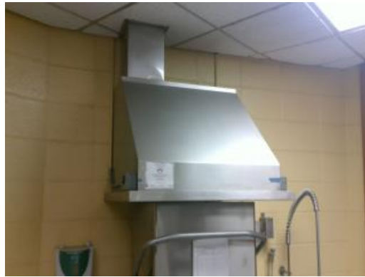
Kitchen Exhaust Hood
