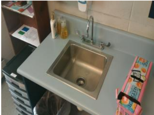
Stained Classroom Lavatory
