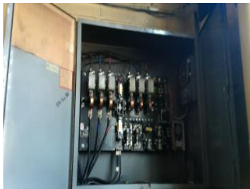
Non-Functional Transfer Switch
