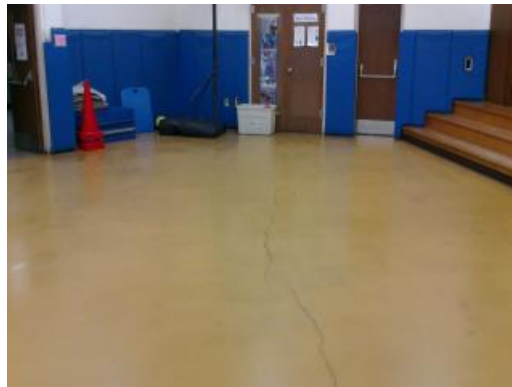
Cracked Gym Floor
