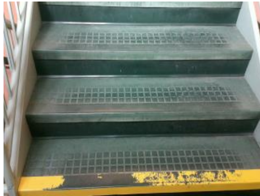
Worn Stair Treads
