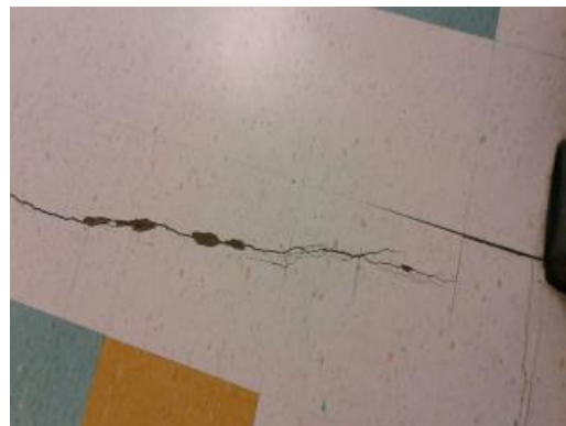
Cracked And Chipped VCT
