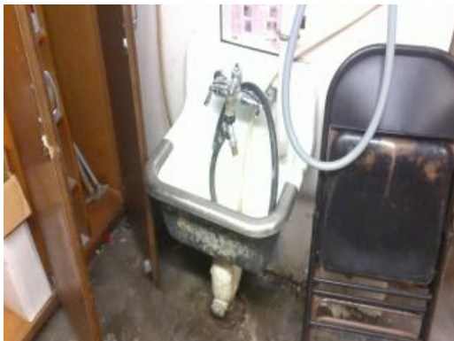
Rusted And Leaking Custodial Sink
