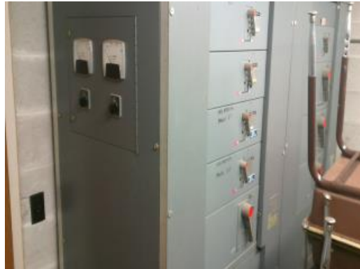
Federal Pacific Switchgear
