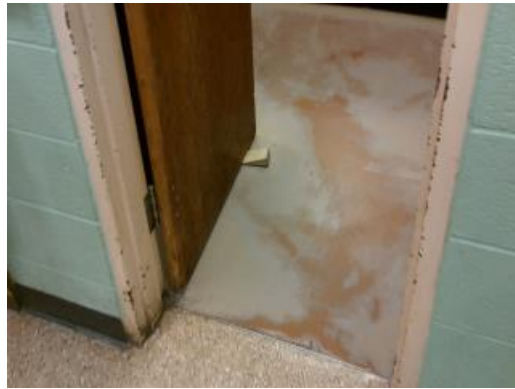
Worn Epoxy Floor
