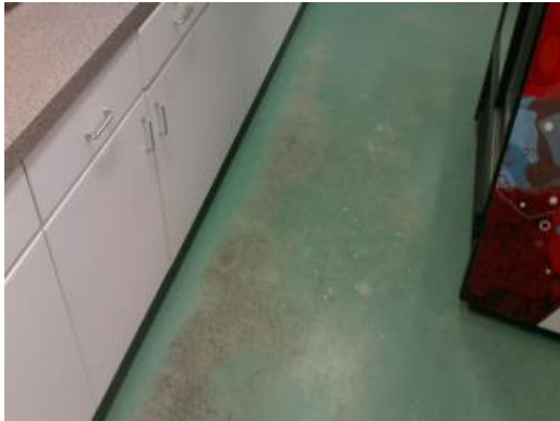
Worn Floor Coating
