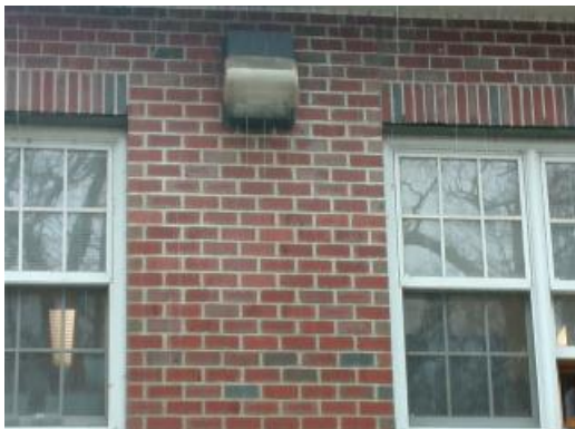
Building Mounted Fixtures
