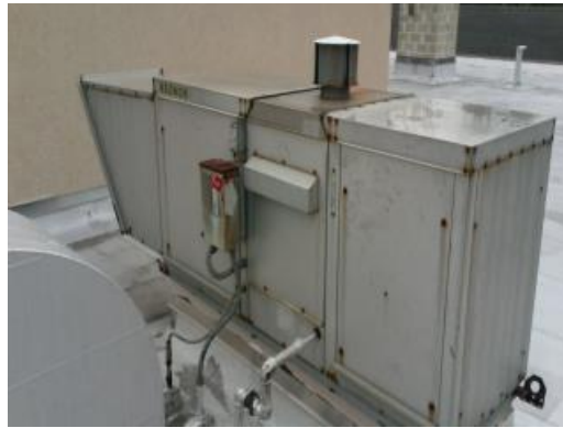
Make Up Air Unit
