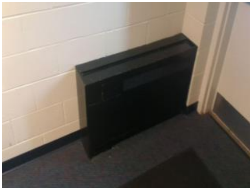
Damaged Heating Unit
