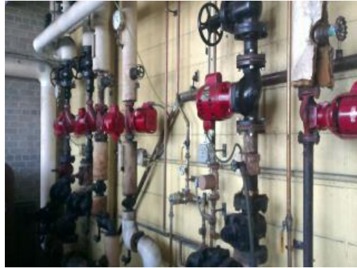
Pumps Rusted And Leaking - Old Section
