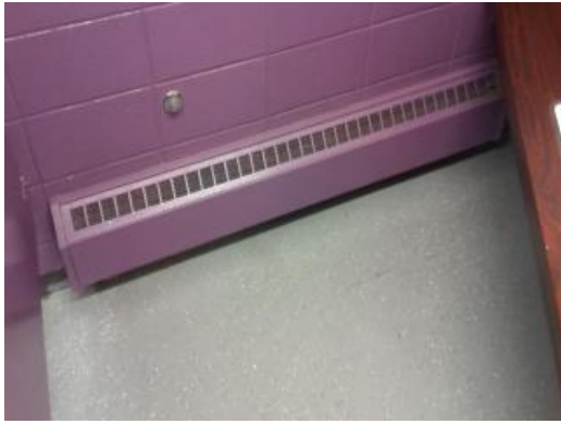
Aged Radiant Heater
