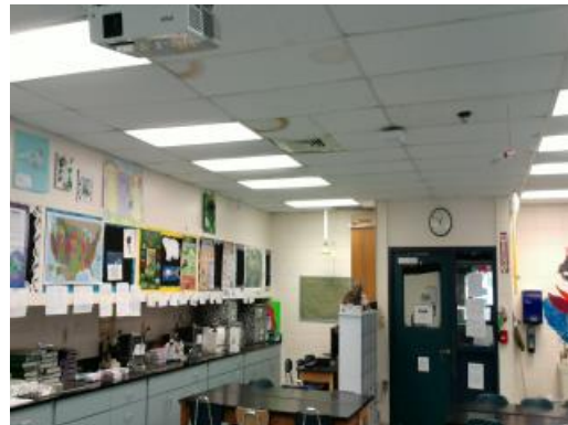
Stained And Broken Ceiling Tiles
