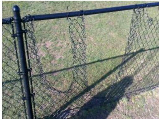
Damaged Chain Link
