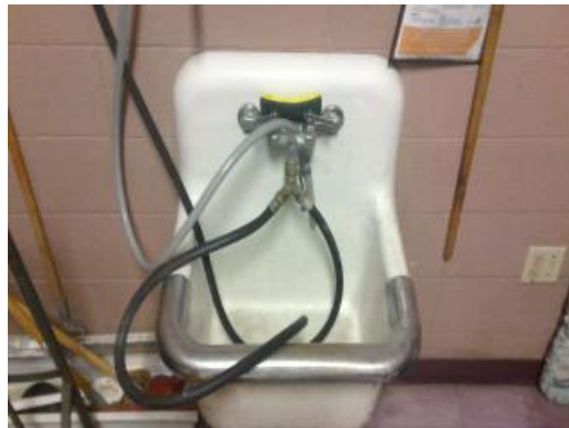
Stained Custodial Sink
