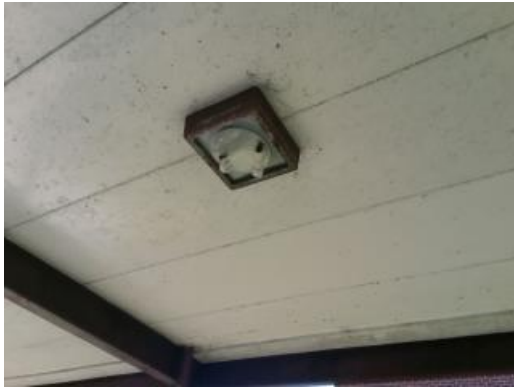
Damaged Canopy Light
