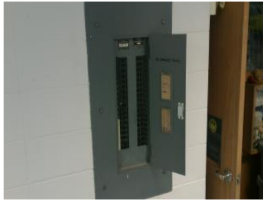
Panelboard With Cracked Breakers
