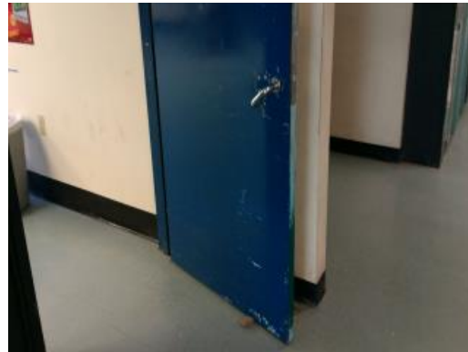
Scratched Door Paint
