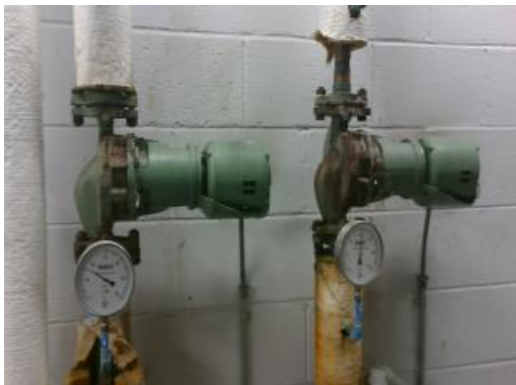
Pumps Rusted And Leaking - New Section
