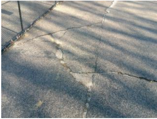
Cracked Asphalt Play Area
