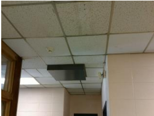
Stained Ceiling Grid
