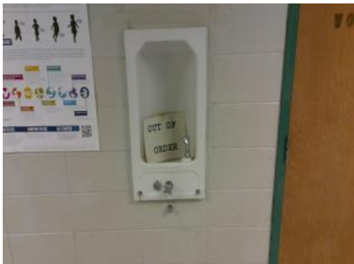
Non-Functional Drinking Fountain
