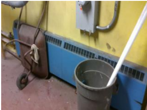
Aged Heating Unit
