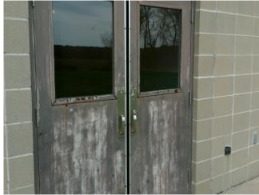
Weathered And Corroded Exterior Doors
