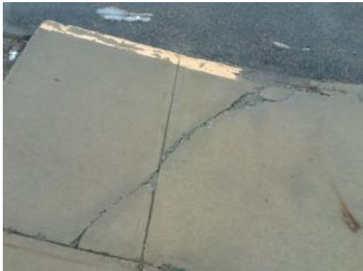
Cracked Concrete Walkway
