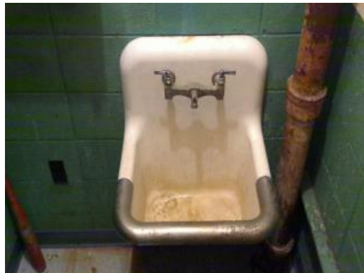
Stained Service Sink
