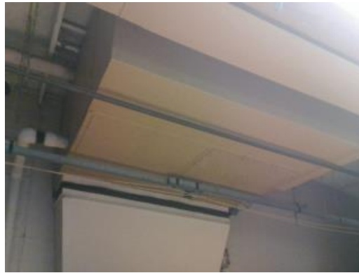
Gym Make Up Air Unit
