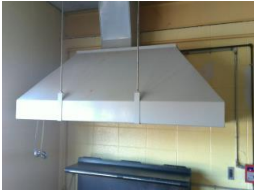
Rusting Kitchen Hood
