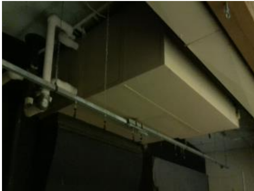
Make Up Air Unit
