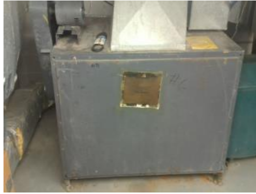
Aged Air Handling Unit
