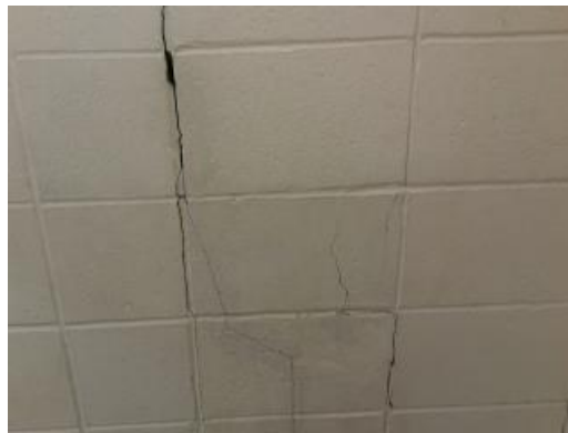
First Floor Northwest CMU Crack
