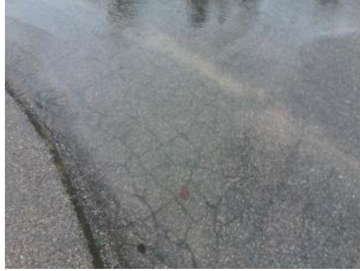
Alligatored Parking Lot Paving
