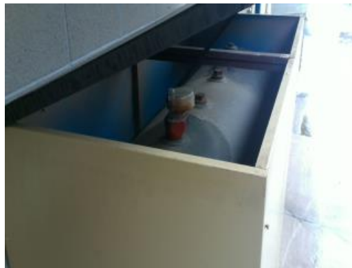
Aged Fuel Storage Tank
