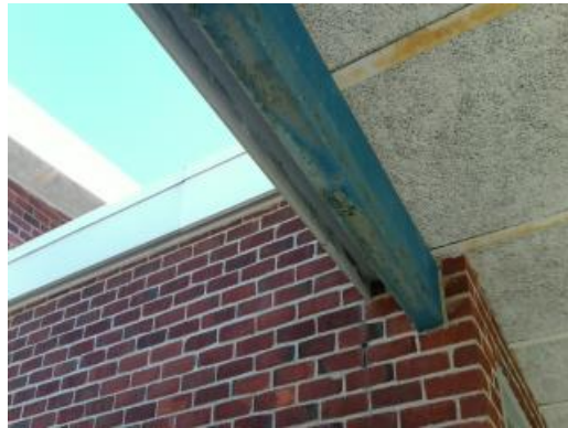
Paint Peeling At Canopies
