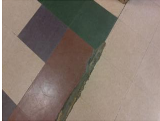
Chipped VCT Flooring
