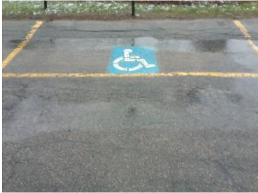
Cracked And Worn Parking
