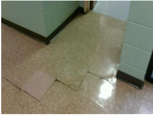
Cracked VCT Floor At Lobby
