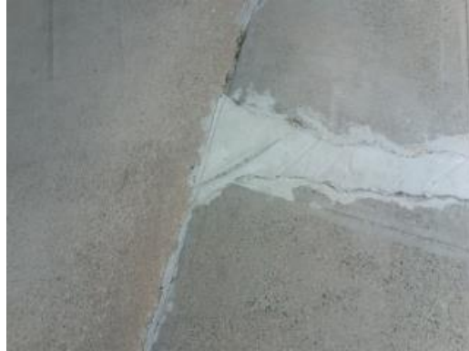
Cracked Concrete Walkway
