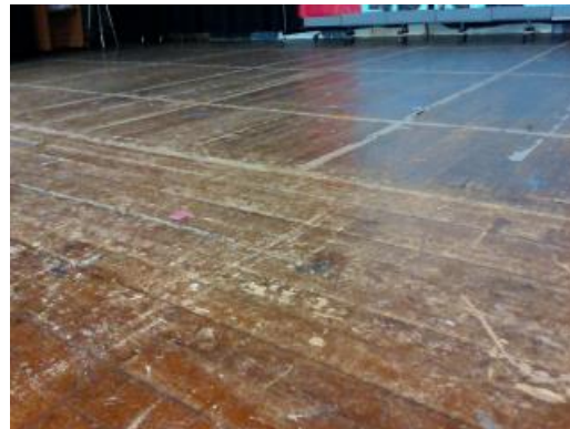
Worn Wood Floor At Stage
