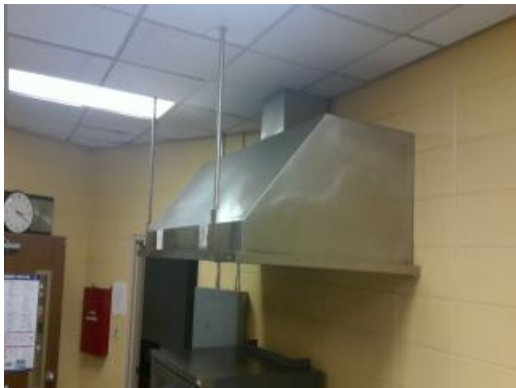
Kitchen Exhaust Hood
