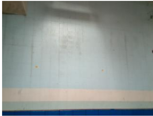
Worn Gym Paint
