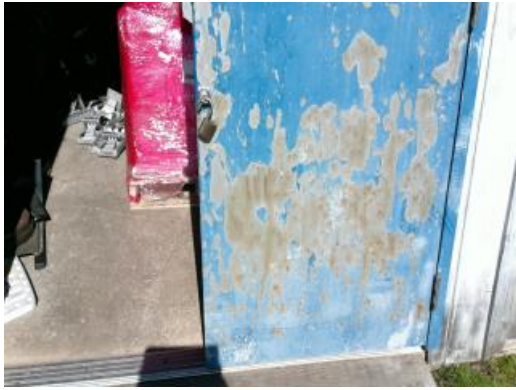
Paint Peeling On Exterior Door
