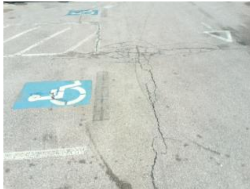
Cracked Parking Lot Pavement
