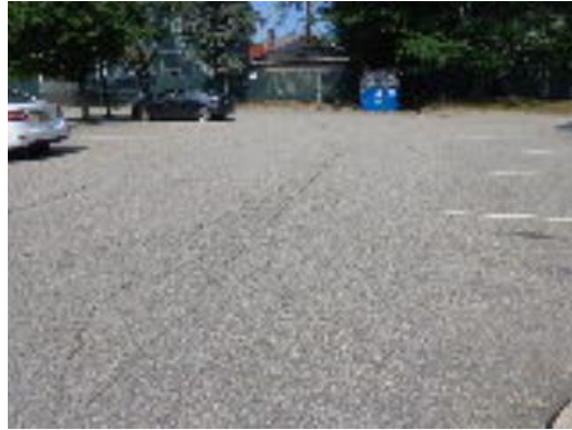
Cracked Asphalt Parking
