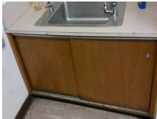
Aged Classroom Cabinetry
