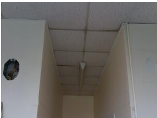
Rusted Ceiling Grid
