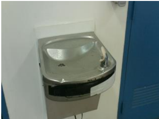
Damaged Drinking Fountain
