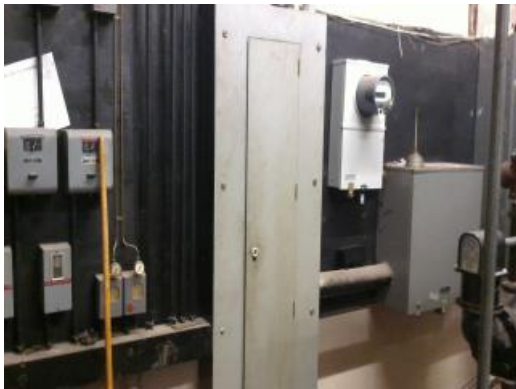
Main Service Panel
