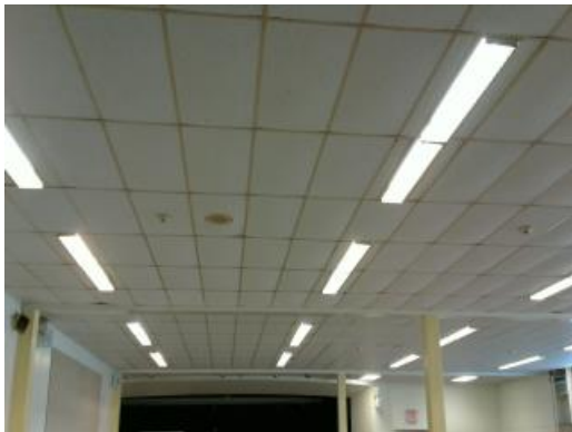
Sagging Ceiling Tiles
