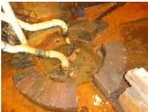
Deficient Sump Pump
