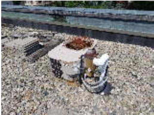
Corroded Condensing Unit
