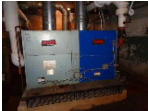
Cast Iron Boilers
