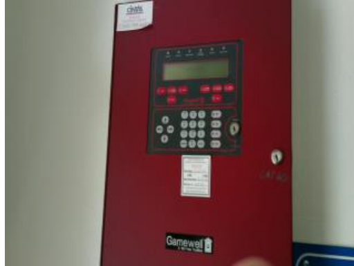
Fire Alarm Control Panel
