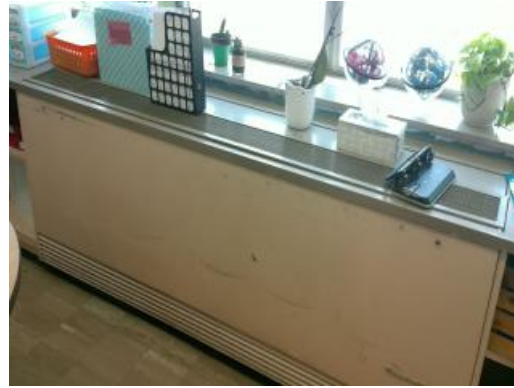
Unit Heater / Ventilator
