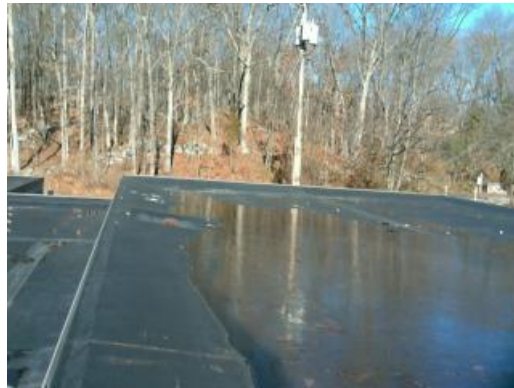
Ponding On Roof
