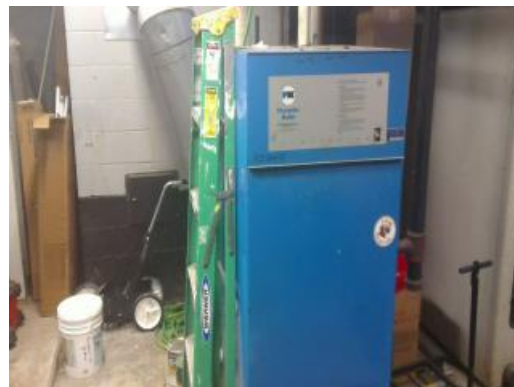
Boiler For Addition
