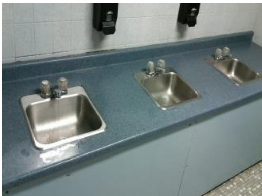
Typical Restroom Lavatories
