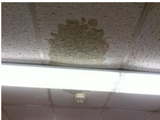
Stained Ceiling Tile
