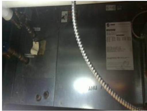
AHU At Addition
