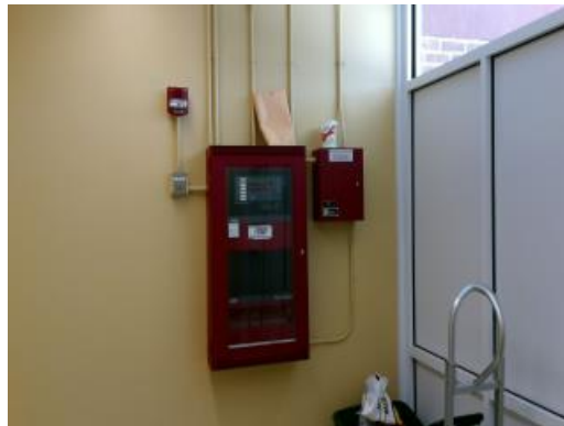
Fire Alarm Panel
