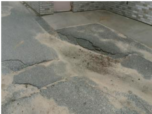
Cracked Asphalt Paving
