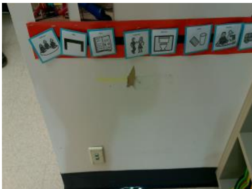
Chipped Interior Wall
