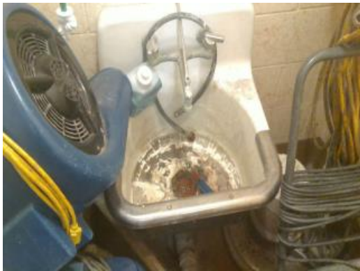
Corroded Janitor Sink
