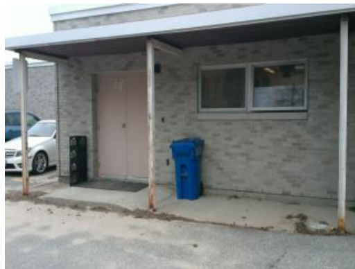
Canopy Beams Rusted
