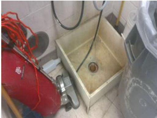
Stained Mop Sink
