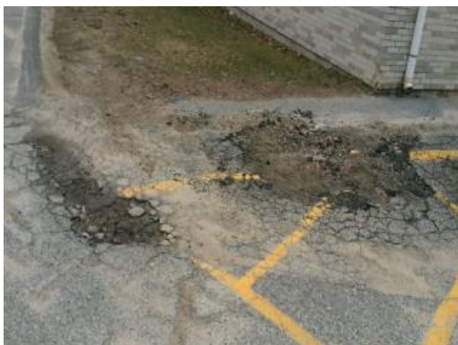
Damaged Asphalt In Parking Lot
