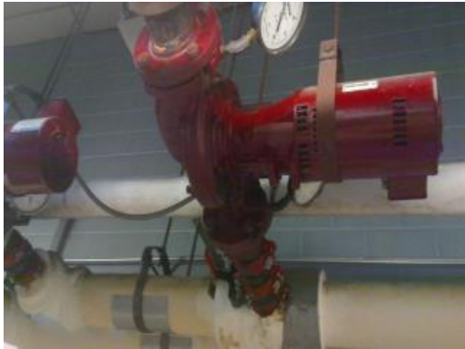
Leaking Circulating Pumps
