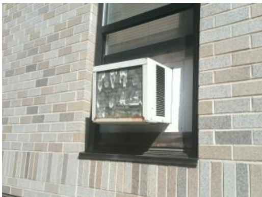
Damaged Window Unit
