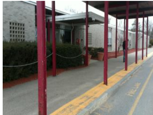
Chipped Paint On Canopy Beams
