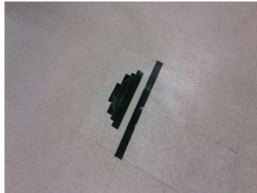
VCT Repaired With Electrical Tape
