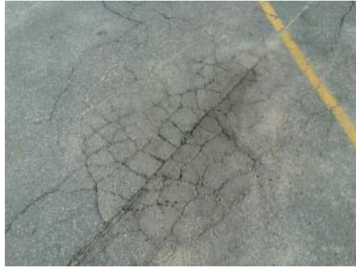
Parking Lot Cracking
