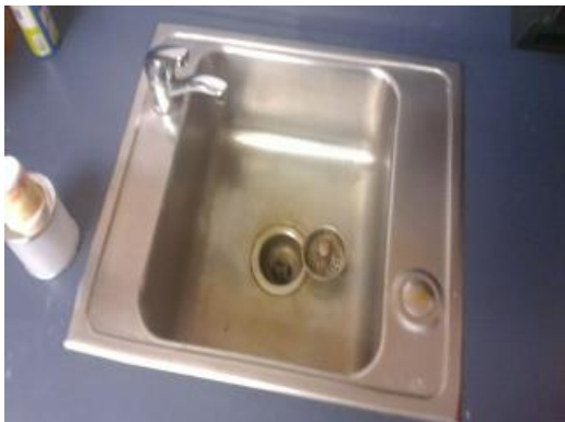
Stained And Rusting Classroom Lavatory
