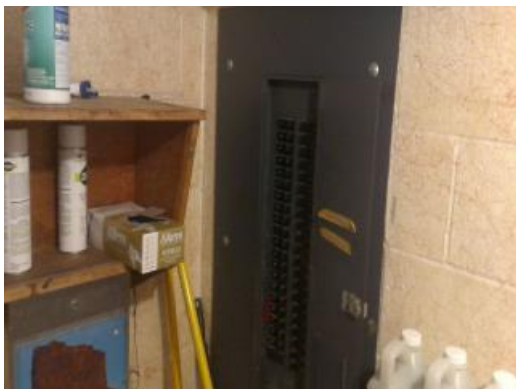
Original 100A Panel
