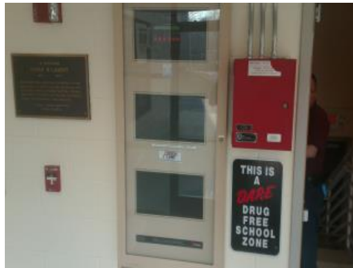
Fire Alarm Panel
