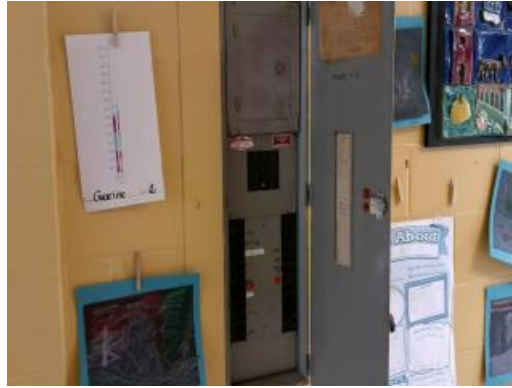
Aged Electrical Panel
