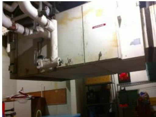
Existing AHU with New Controls
