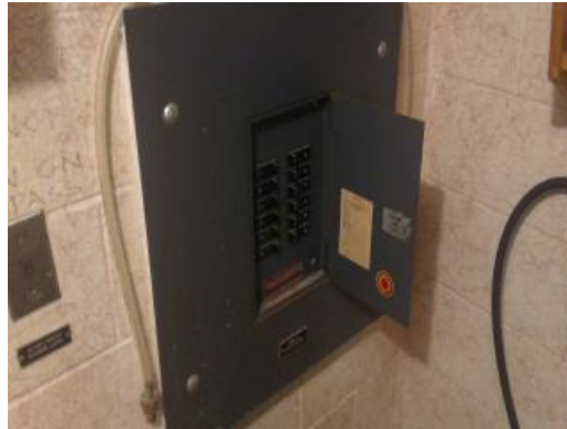
Aged Distribution Panel
