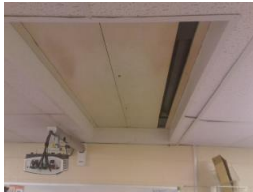
Ceiling Mounted Unit Heater
