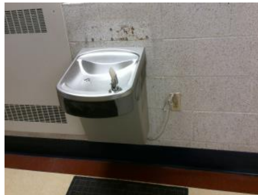
Refrigerated Drinking Fountain
