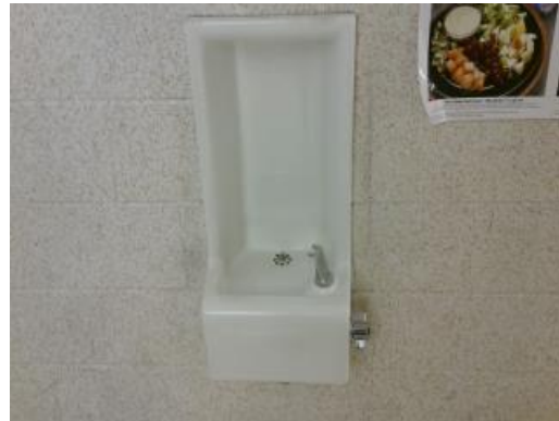
Non-Refrigerated Drinking Fountain
