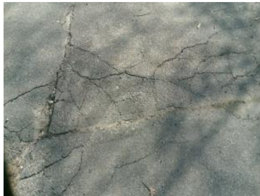
Damaged Roadway Asphalt
