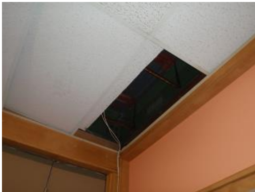
Missing Ceiling Tile
