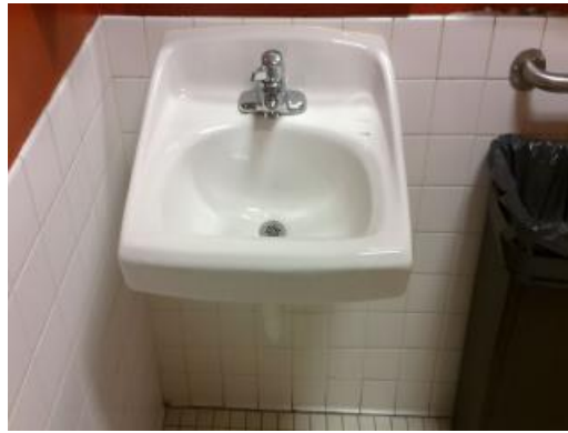
Typical Restroom Sink
