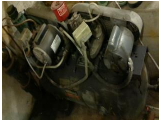
Leaking Air Compressor
