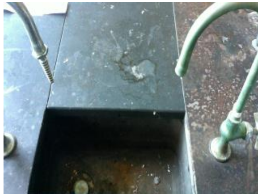
Corroded Classroom Lavatory
