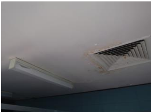
Peeling Plaster Ceiling
