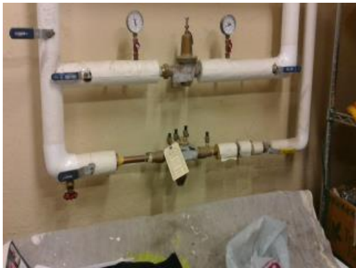
Boiler Make-Up Backflow Preventer
