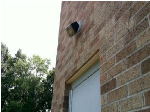
Building Mounted Light
