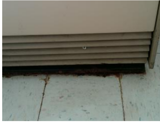
Rusted Unit Vent
