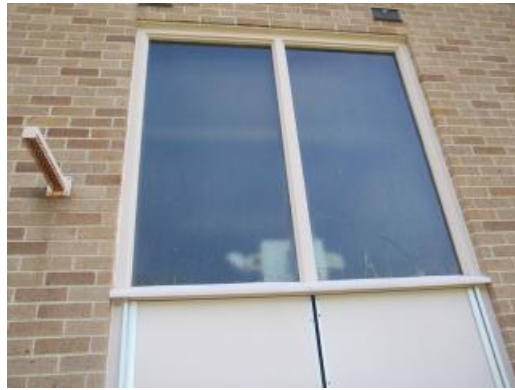
Broken Glass Pane
