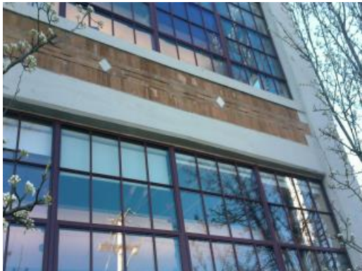
Exterior Brick Walls Require Repointing
