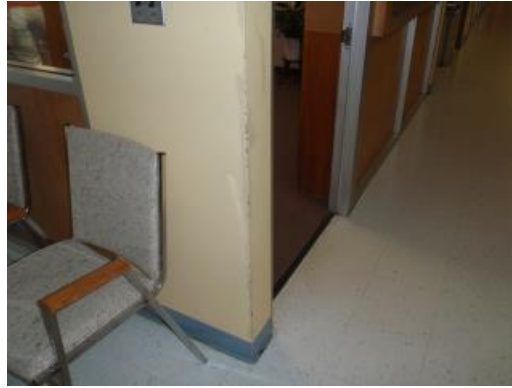
Chipped Wall Paint
