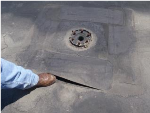
Open Roof Seam
