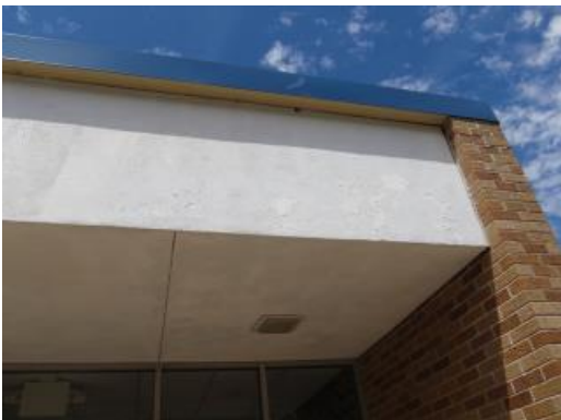
Chipped Stucco Paint
