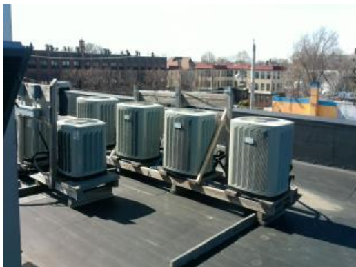
Condensing Unit Group
