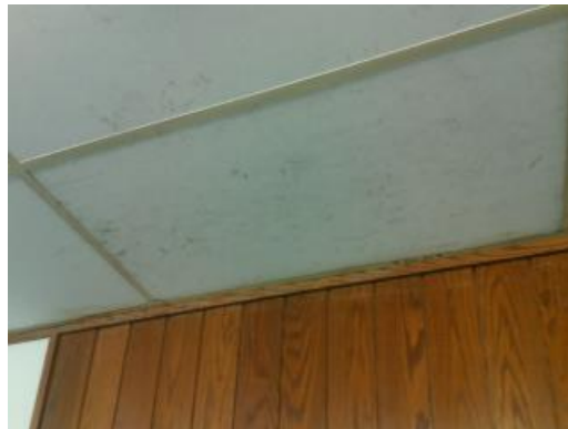
Rusting Ceiling Grid
