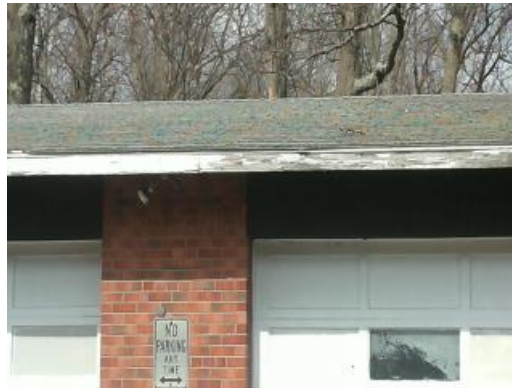
Deteriorating Shingle Roof
