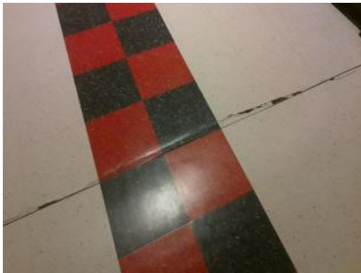
Main Building - Cracked VCT
