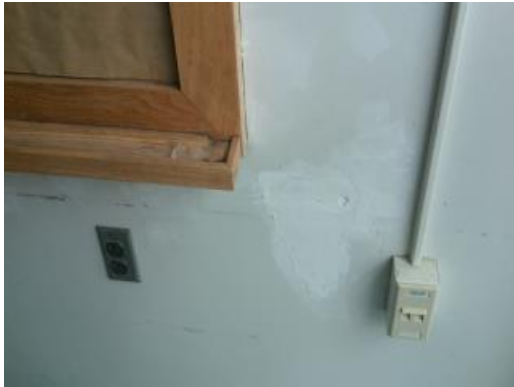
Main Building - Damaged Interior Wall
