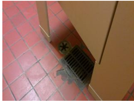
Broken Quarry Tile Flooring
