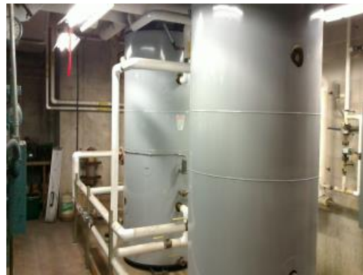
Main Building - Hot Water Storage Tanks
