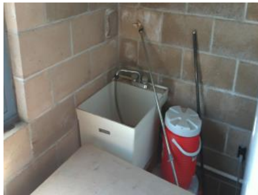
Building 04 - Mop Sink
