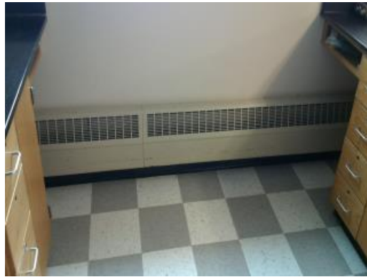
Main Building - Radiant Heaters
