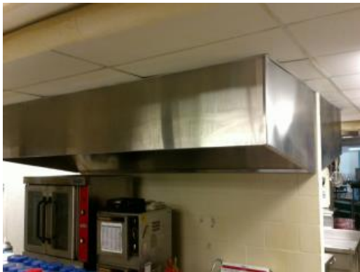
Main Building - Kitchen Hood
