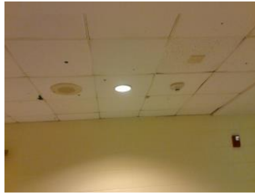
Main Building - Damaged Acoustical Ceiling Tiles
