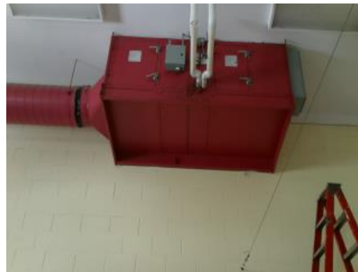
Main Building - Make-up Air Unit
