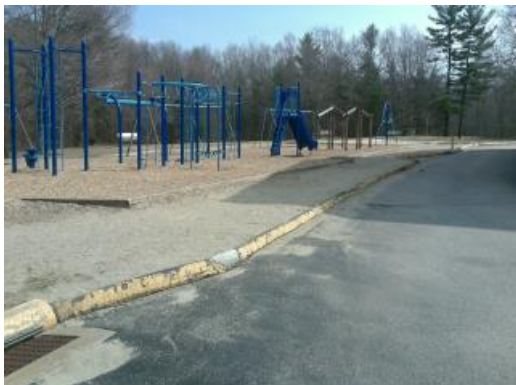
No ADA Playground Access
