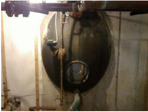
Building 04 - Domestic Water Storage Tank
