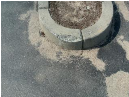
Damaged Concrete Curbs
