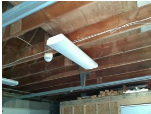
Building 04 - Typical Light Fixture
