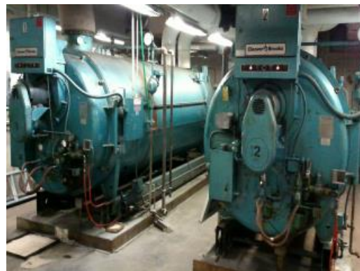
Main Building - Boilers
