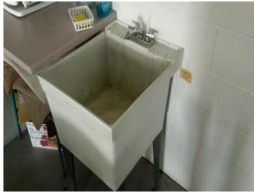
Stained Mop Sink
