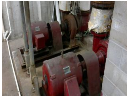
Main Building - Hot Water Pumps
