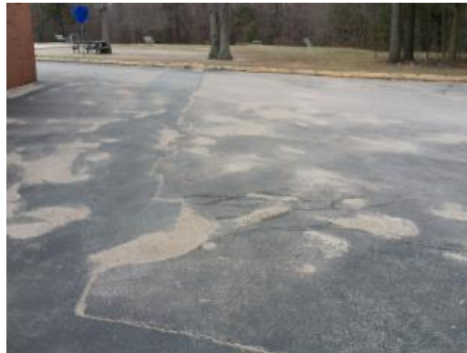
Worn Asphalt Paving
