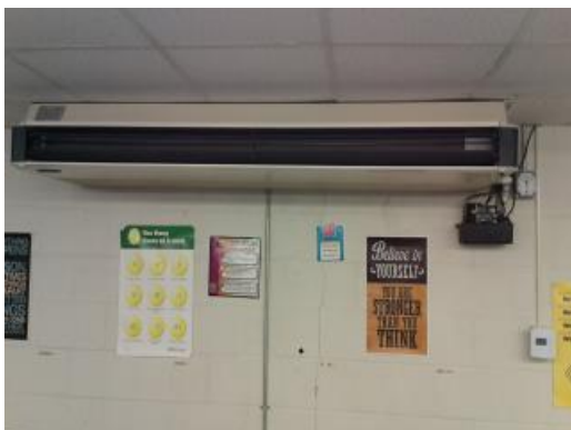
Main Building - Fan Coil
