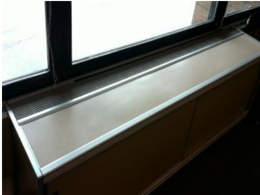
Original Heating Unit
