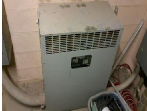
Federal Pacific Transformer
