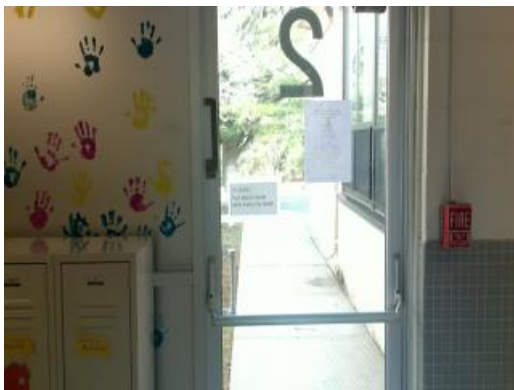
Exterior Door Not Closing Properly
