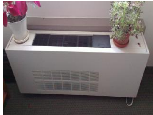
Building 02 - Unit Ventilator
