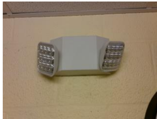
Battery Operated Emergency Lighting
