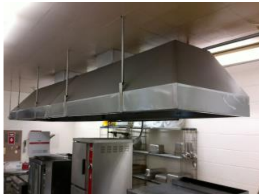
Original Kitchen Exhaust Hood
