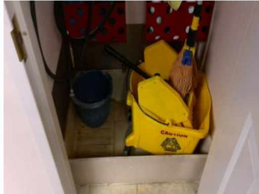
Building 02 - Mop Sink
