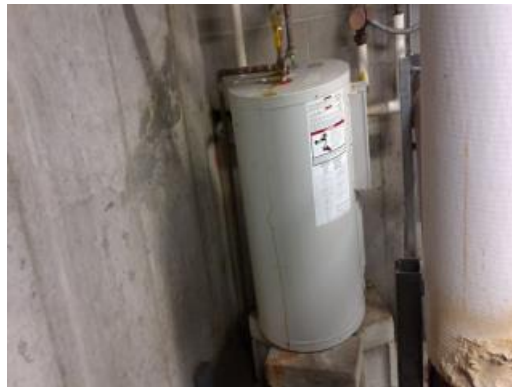
Main Building - Electric Water Heater
