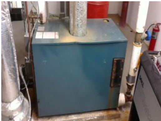
Building 02 - Boiler - Domestic Water
