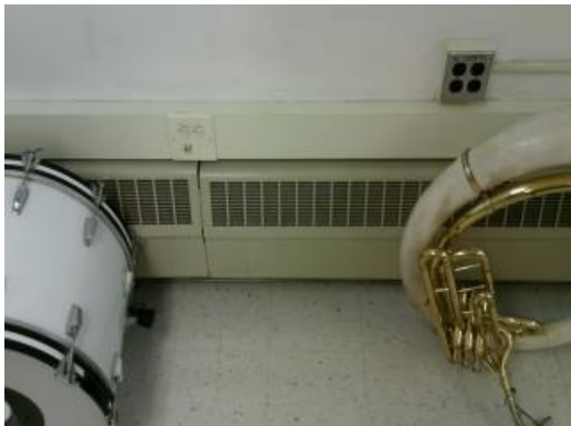
Main Building - Radiant Baseboards
