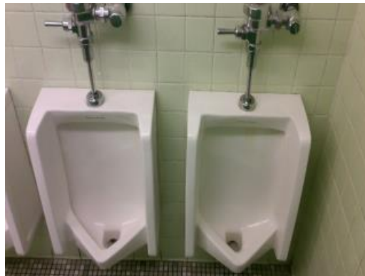
Original Urinal Fixtures
