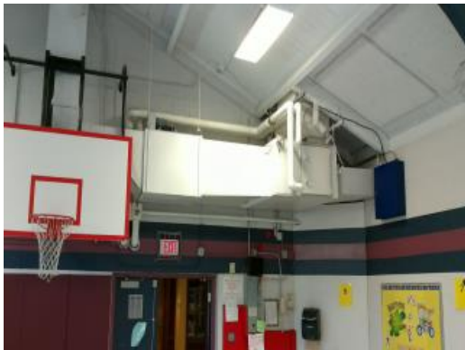
AHU In Gymnasium
