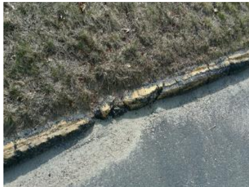
Damaged Asphalt Curbs
