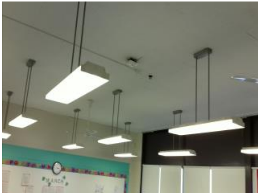
Typical Fluorescent Lighting
