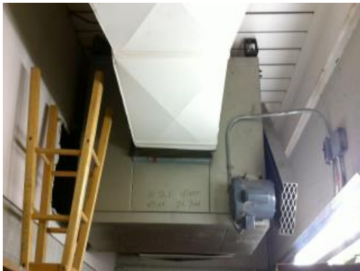
Original Make-up Air Unit
