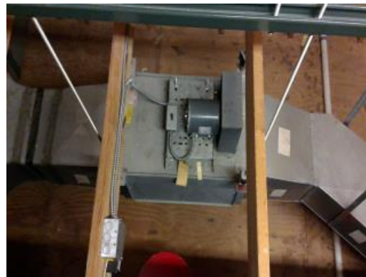
Exhaust System Ventilator For New Wing 4X
