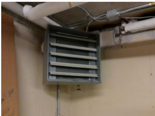
Building 02 - Hot Water Unit Heater
