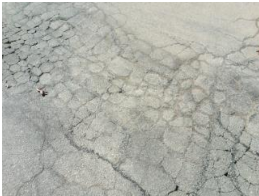
Site - Cracked Asphalt Pavement
