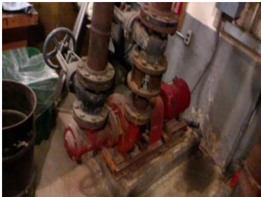
Original Heating Hot Water Pumps
