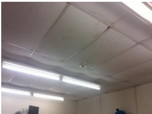
Sagging Ceiling Tiles
