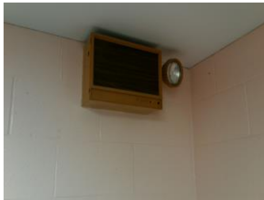
Original Battery Backup Lights
