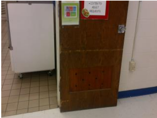
Worn Kitchen Door
