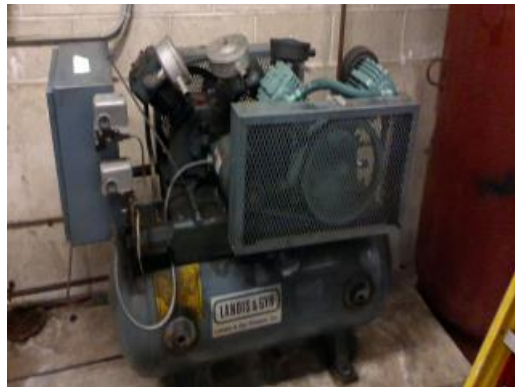
Main Building - Compressor
