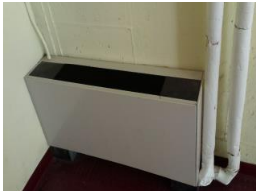
Main Building - Classroom Unit Heater
