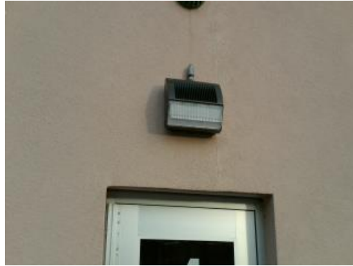
Building Mounted Lighting
