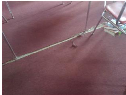
Main Building - Worn And Bubbling Carpet
