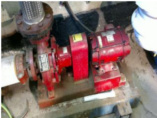
Hot Water Distribution Pump
