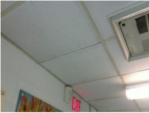
Ceiling Grid Missing Pieces
