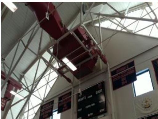
Main Building - Make-up Air Unit
