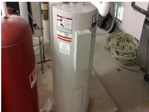
Building 02 - Water Heater
