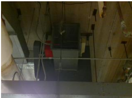
Make-up Air Unit
