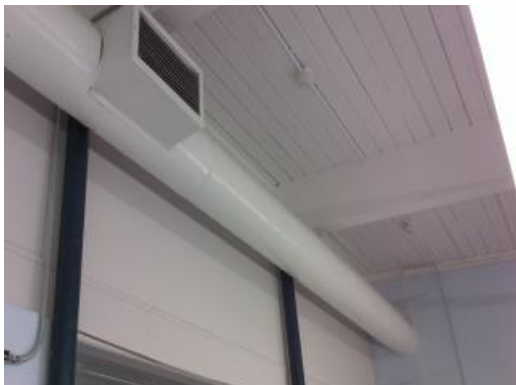
Ductwork For Exhaust
