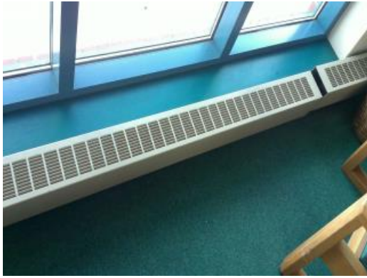
Main Building - Radiant Heaters
