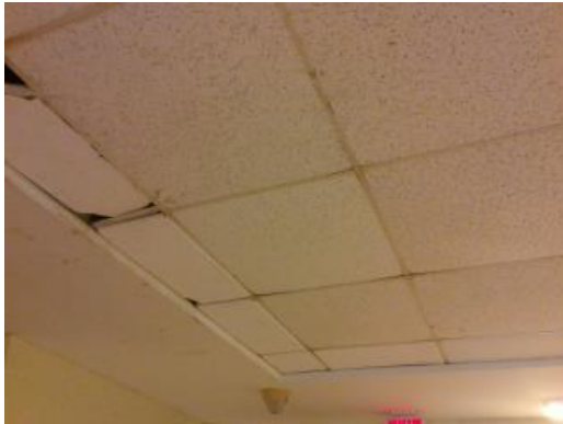
Main Building - Rusted Ceiling Grid
