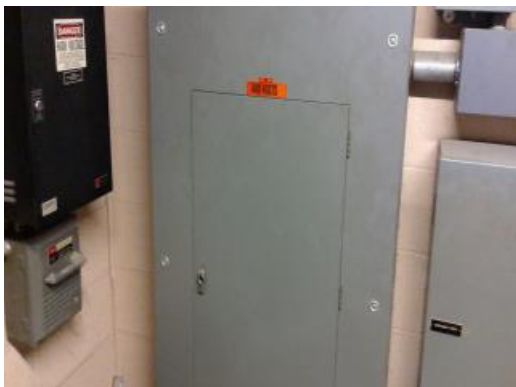
Federal Pacific Panelboard
