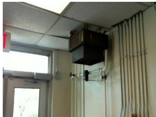
Entry Unit Heater
