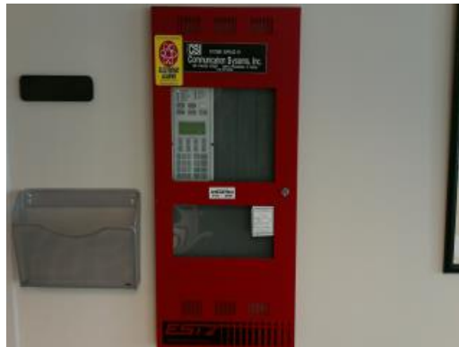
Building 02 - Electronic Alarm System
