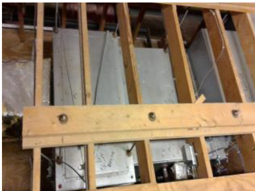
Office Air Handler With DX Coil And Heating Coil
