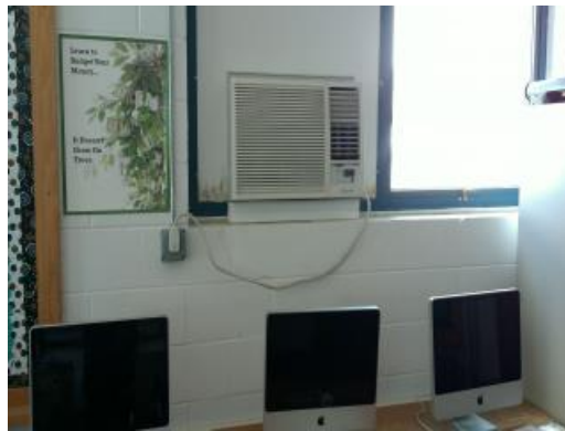
Main Building - Window AC Unit
