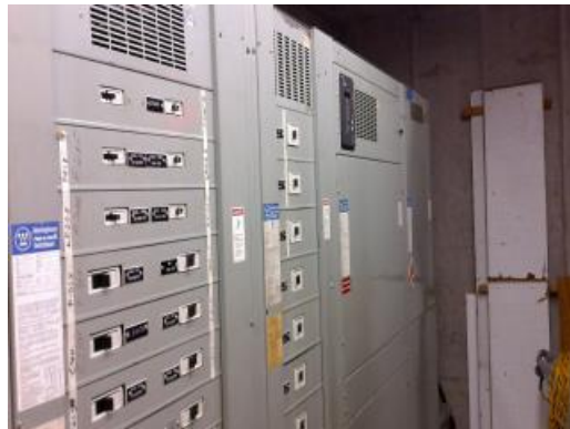
Main Electrical Service
