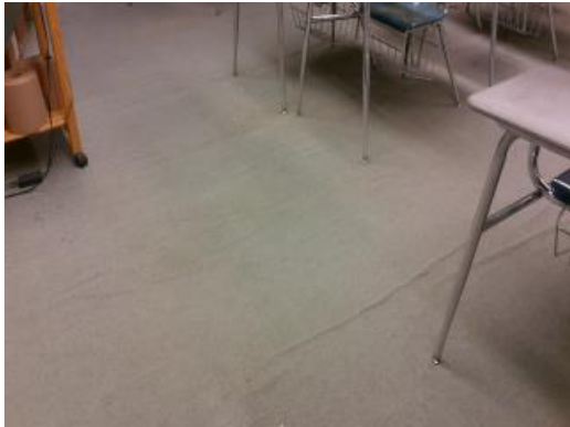
Worn Classroom Carpet
