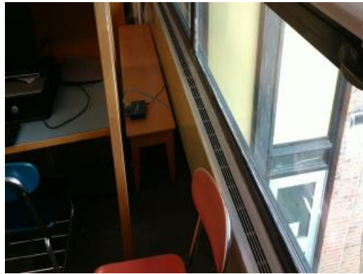
Original Radiant Heater
