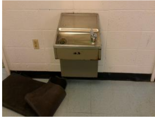
Damaged Refrigerated Drinking Fountain
