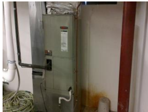
Building 02 - Air Handling Unit
