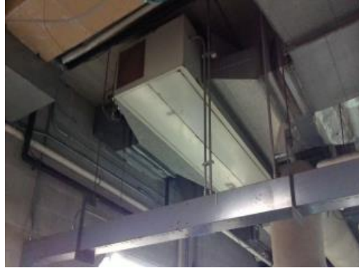
Main Building - Ducted Ceiling Hung Unit Heater
