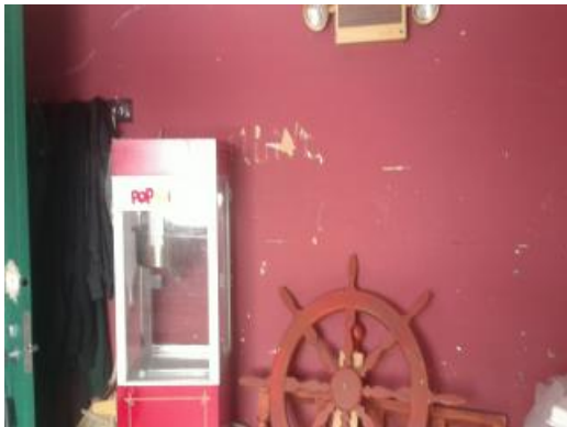
Main Building - Chipped Wall Paint
