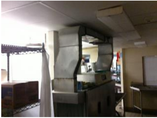
Main Building - Dishwasher Exhaust
