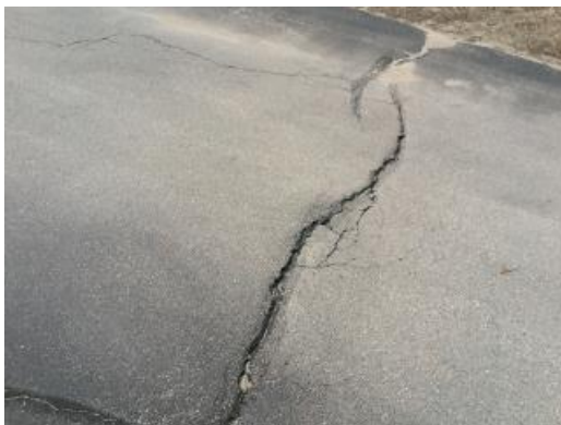
Cracked Asphalt Roadway
