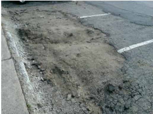
Fully Deteriorated Asphalt
