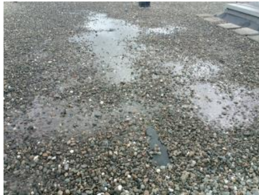
Ponding On Roof
