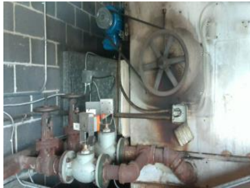
Failing Belt At AHU
