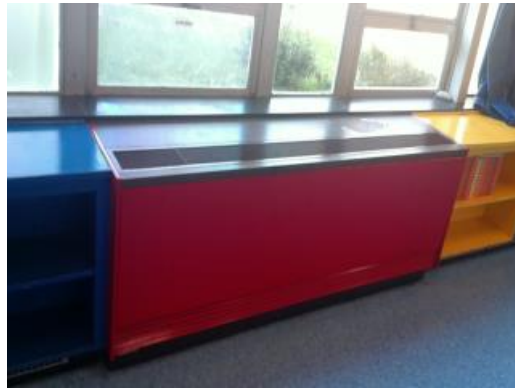
Cabinet Unit Ventilator
