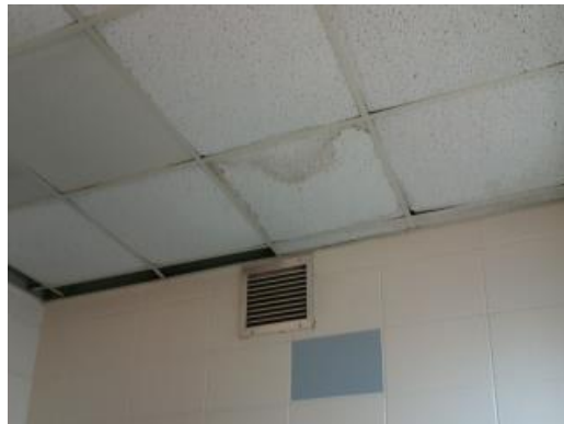
Stained Ceiling Tiles
