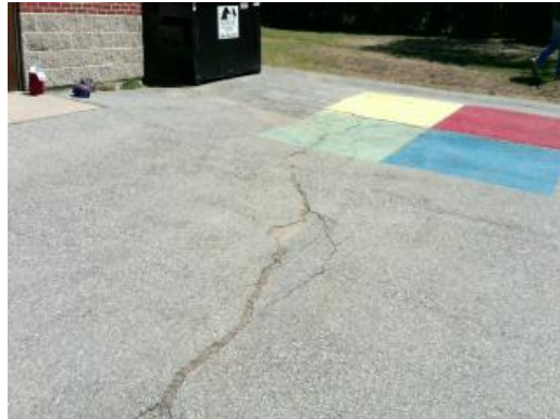
Cracked Paved Play Area
