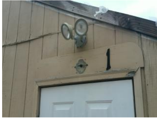
Building Mounted Lights
