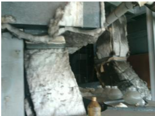
Failing AHU Insulation
