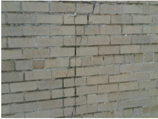
Cracked Exterior Brick
