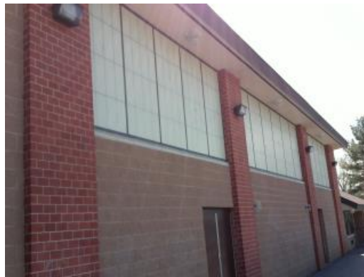
Aged Building Lights
