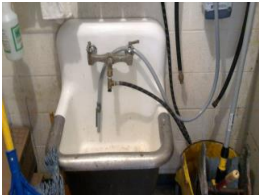
Aged Service Sink
