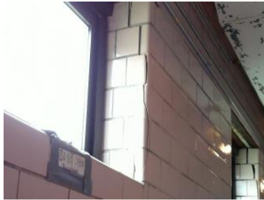
Cracked Tile Wall
