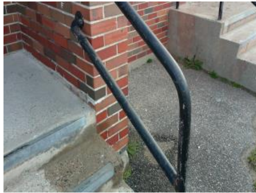
Worn Paint On Handrail
