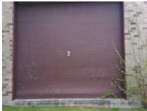
Aged Overhead Door
