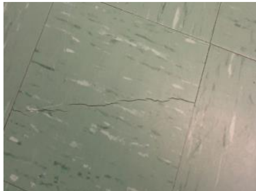
Cracking In VCT
