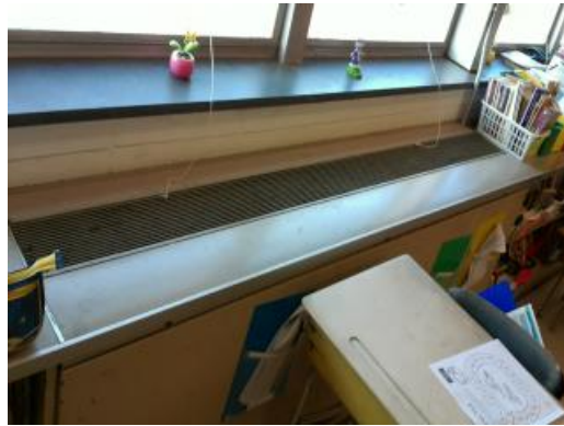
Cabinet Unit Heater
