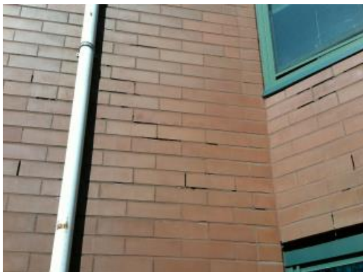
Brick Repointing Required
