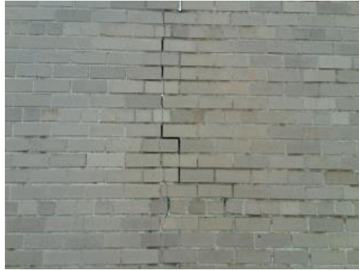
Cracked Exterior Brick
