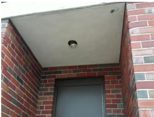
Damaged Canopy Light
