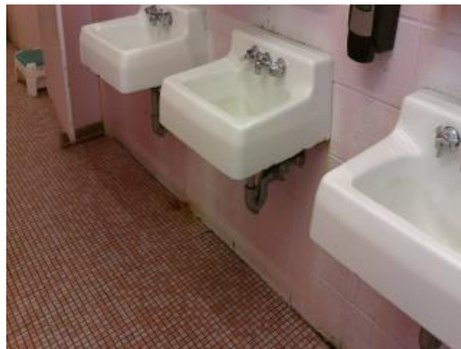
Pipe Insulation Missing
