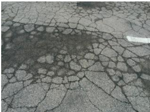
Parking Lot Asphalt Alligating
