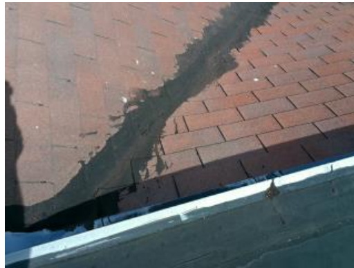
Failed Roof Repairs
