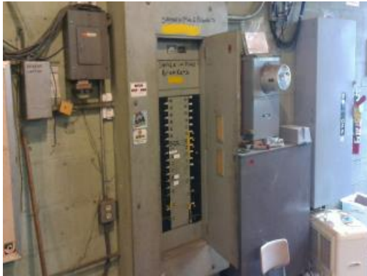
600 Amp Distribution Panel
