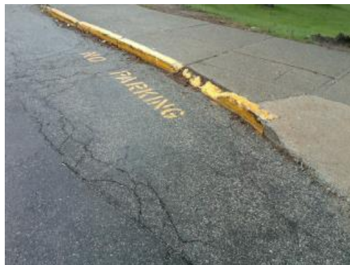
Alligatoring Roadway Pavement
