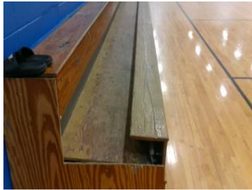
Worn Wood Bleachers
