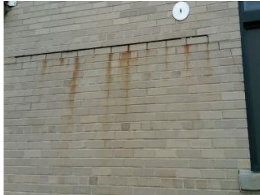
Cracked Exterior Brick
