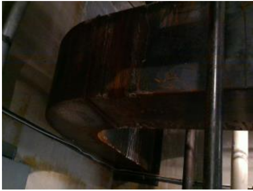
Aged Rusted Ductwork
