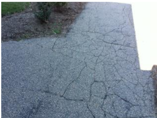
Cracking At Sidewalk
