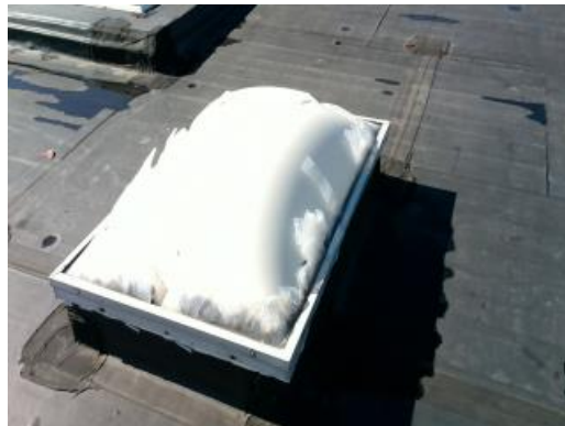
Typical Damaged Skylight
