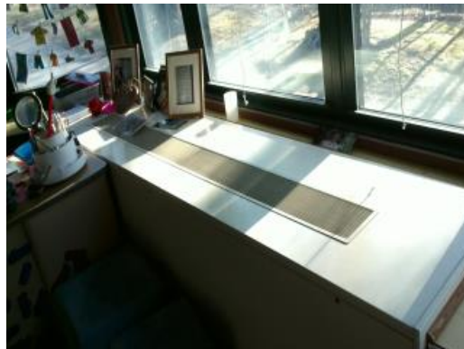
Cabinet Unit Heater
