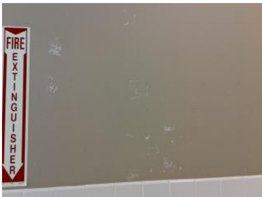
Scuffed Wall Paint
