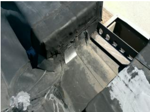
Hole In Membrane
