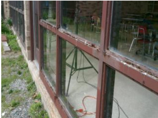
Leaking Steel Windows
