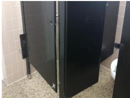
Damaged Restroom Partition
