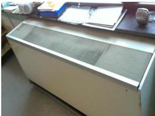
Aged Heating Unit
