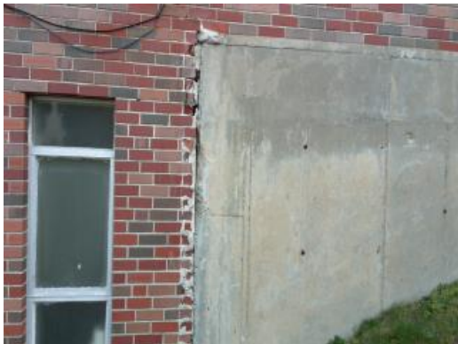
Damaged Brick At Concrete Wall
