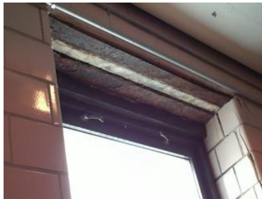
Rusted Steel Lintel
