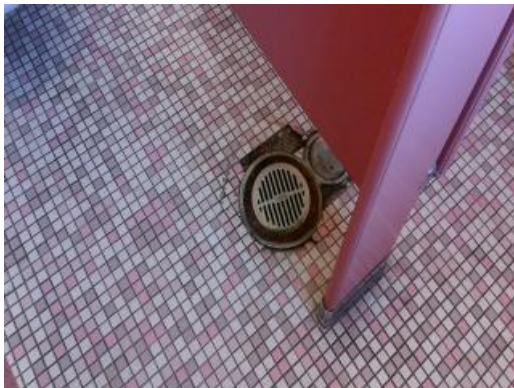
Damaged Ceramic Tile
