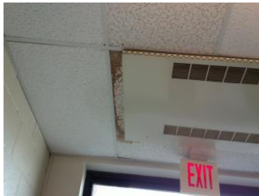
Stained Ceiling Tile
