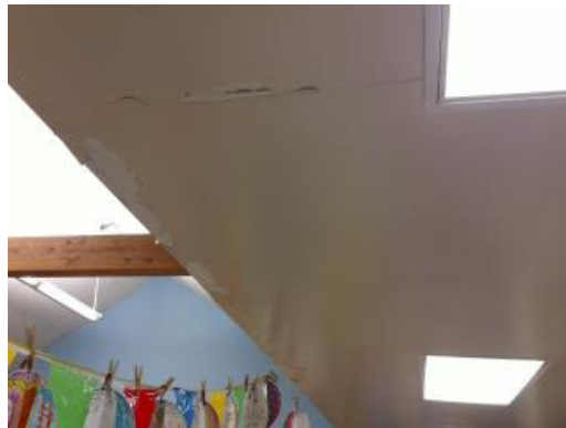
Chipped And Peeling Paint
