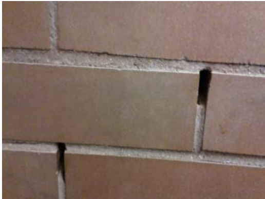
Brick Repointing Required
