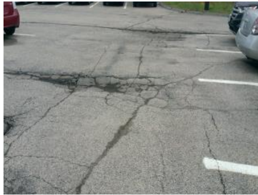
Large Potholes In Asphalt Parking
