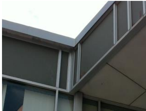
Rusted Metal Panels
