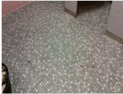
Chipped And Missing Ceramic Tiles
