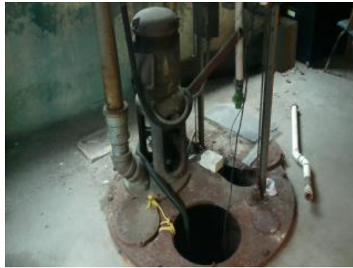
Aged Sump Pump
