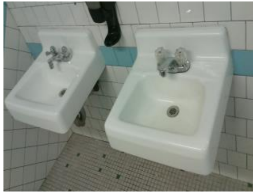
Typical Restroom Lavatories
