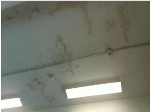
Peeling Ceiling Paint
