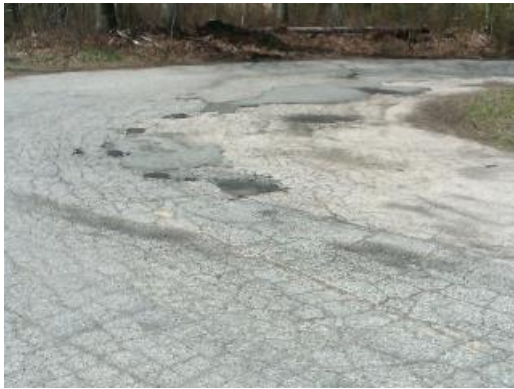
Alligatoring Asphalt And Potholes
