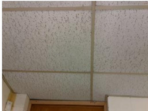
Broken Ceiling Tile
