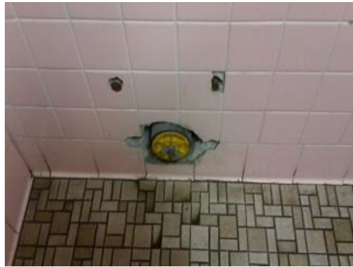
Missing Drinking Fountain
