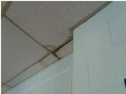
Stained Ceiling Tile
