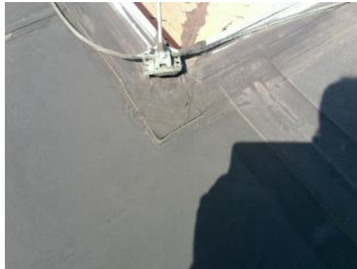
Typical Holes In EPDM
