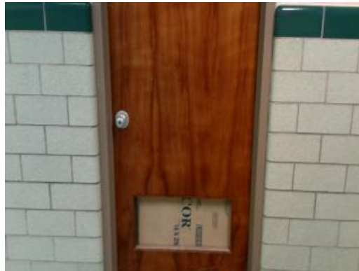
Aged Interior Door With Non-Compliant Hardware
