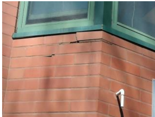
Brick Repointing Required
