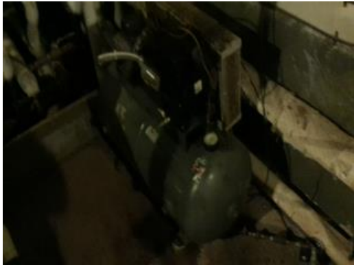
Aged Air Compressor
