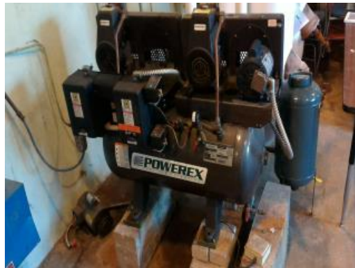
Aged Air Compressor
