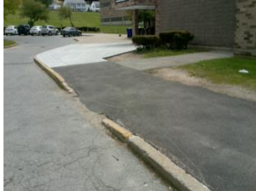
Weathered Roadway Asphalt
