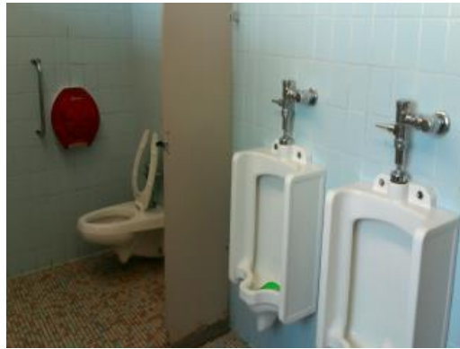
Urinals And Toilet
