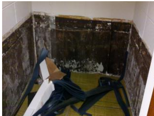
Worn Wall Painting
