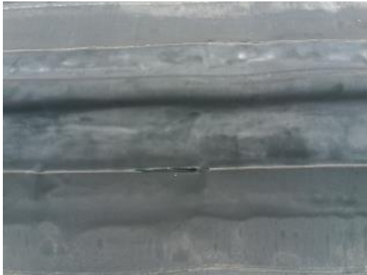
Torn Membrane Roof
