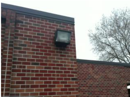
Typical Building Mounted Light
