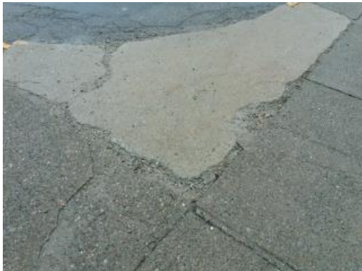
Damaged Concrete Walkways
