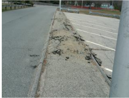
Typical Asphalt Sidewalk Condition
