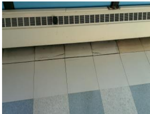
Separating VCT Flooring
