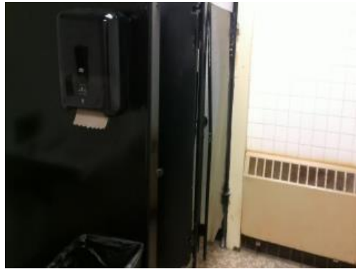
Damaged Toilet Partition
