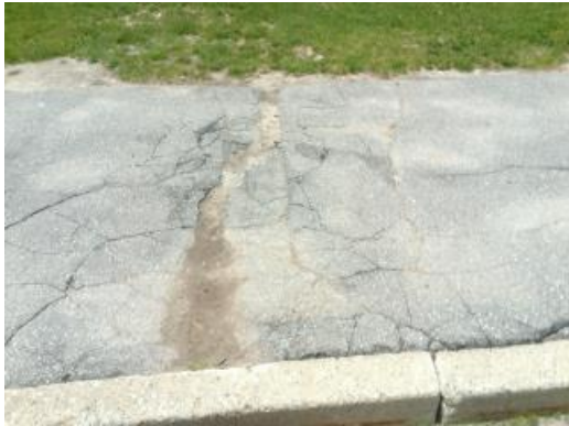
Alligatoring Asphalt Walkway
