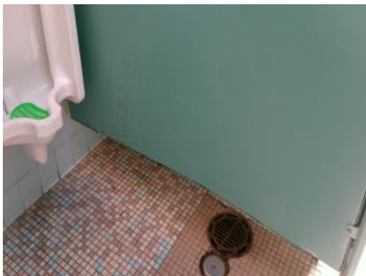
Rusted Toilet Partition
