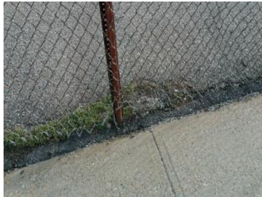
Damaged Chain Link
