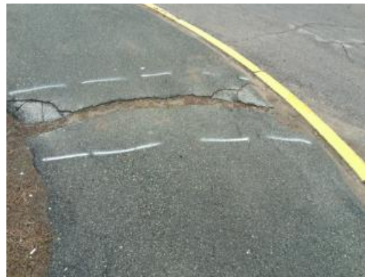
Cracked Asphalt Walkway
