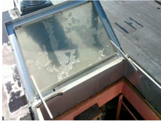
Broken Roof Hatch
