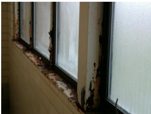
Corroded Steel Windows
