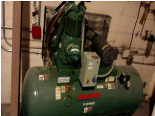
Aged Air Compressor
