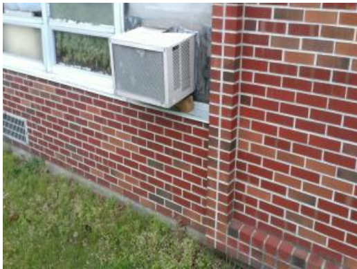
Old Window Unit
