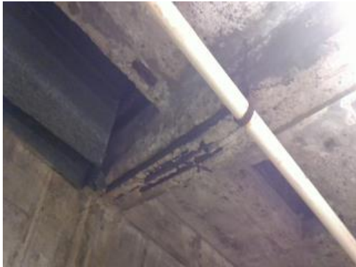
Damaged Concrete Deck
