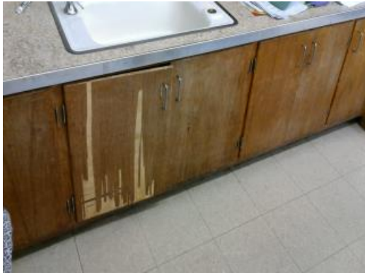
Typical Worn Casework
