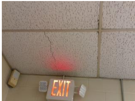
Cracked Ceiling Tile
