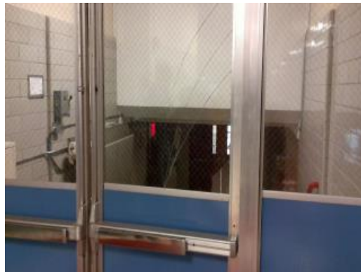
Damaged Storefront Door
