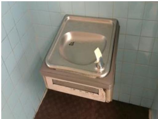
Refrigerated Water Cooler
