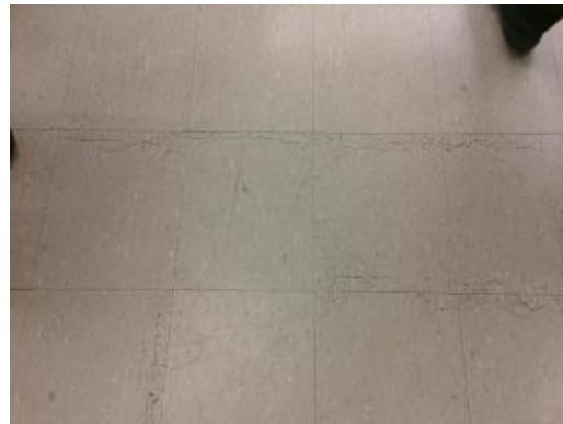
Cracked And Worn VCT
