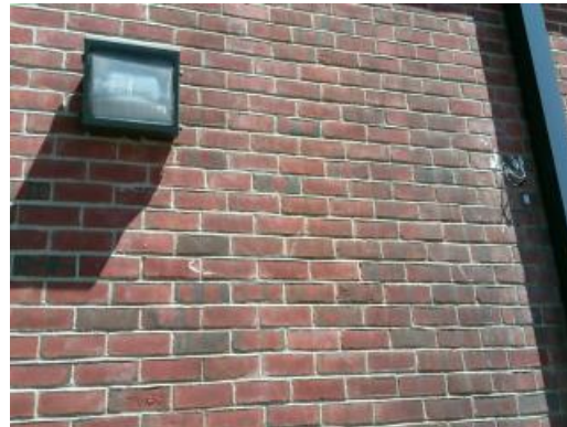
Building Mounted Light
