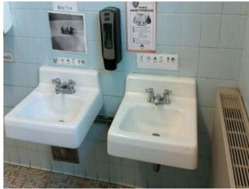
Non-ADA Restroom Plumbing Fixtures
