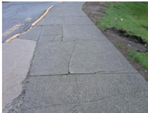
Cracked Concrete Walkway
