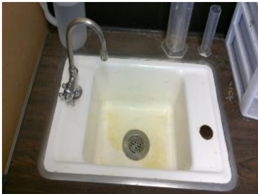
Stained Classroom Sink
