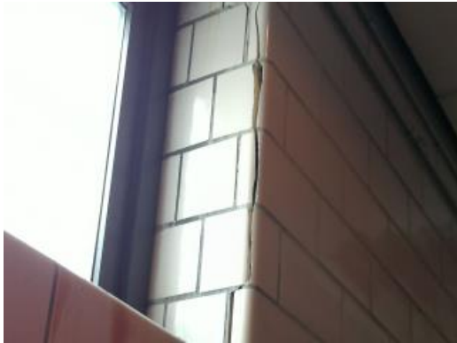
Cracked Tile Wall
