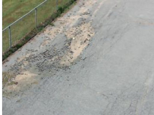
Deteriorated Roadway Asphalt
