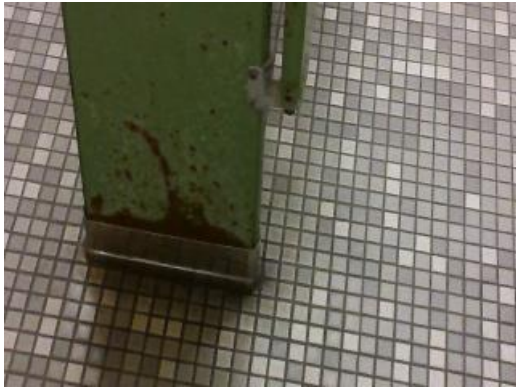
Toilet Partition Damage
