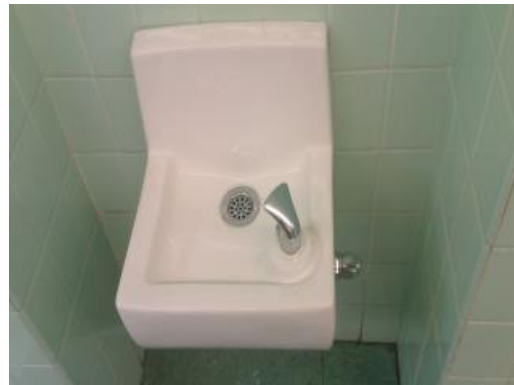
Non-Refrigerated Water Fountain
