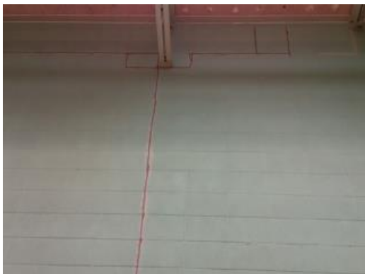
Cracked CMU Wall
