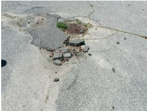
Damaged Asphalt Paving
