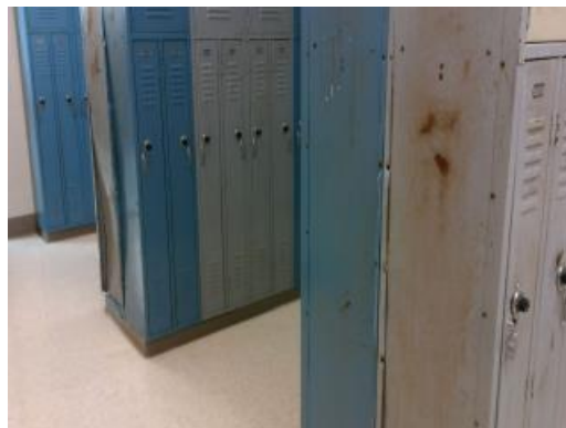
Damaged And Rusted Lockers
