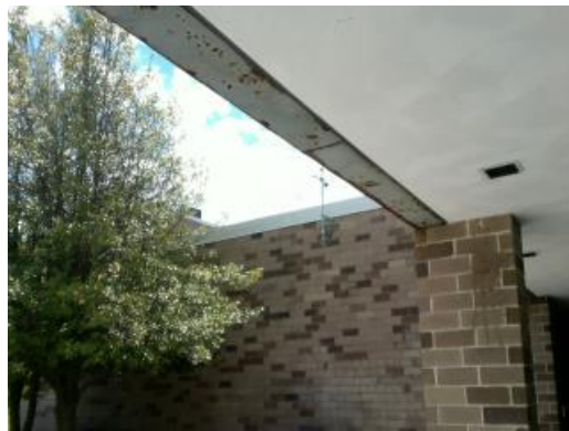
Corroded Soffit Lintel
