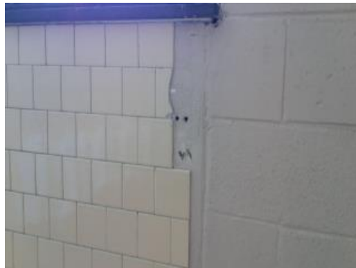
Chipped And Missing Ceramic Tiles
