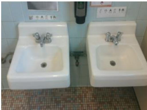
Restroom Lavatories Plumbing Fixtures
