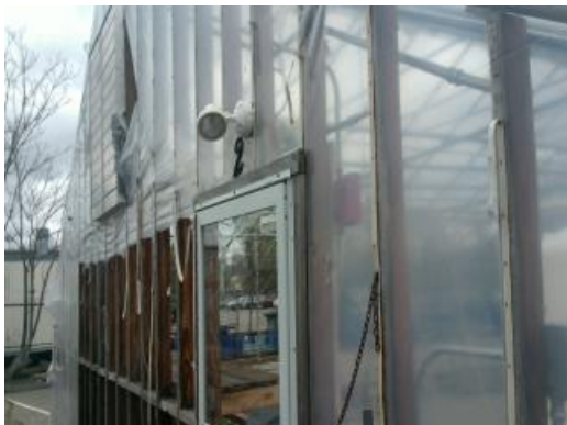
Building Mounted Lights
