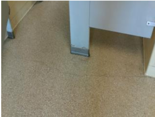
Cracked And Worn Terazzo
