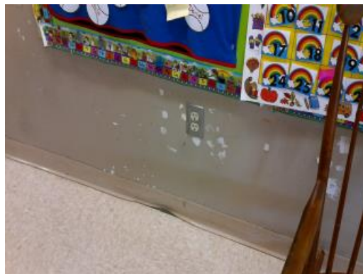
Chipped And Stained Wall Paint
