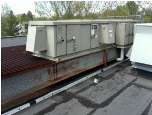
Aged Air Handling Unit
