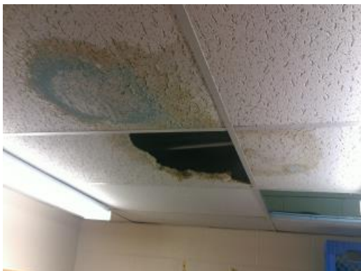
Stained And Broken Tiles
