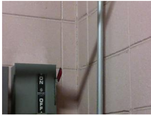
Crack In CMU
