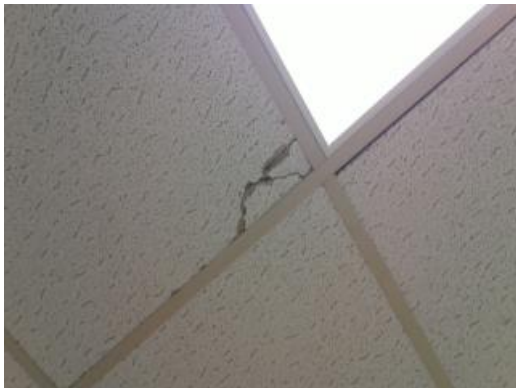
Broken Ceiling Tile
