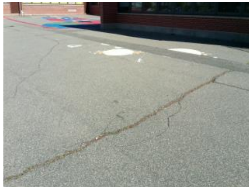
Cracks In Play Area Asphalt
