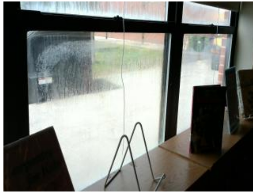
Damaged Window Pane
