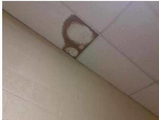
Stained Ceiling Tile
