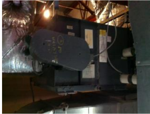
Air Handling Unit
