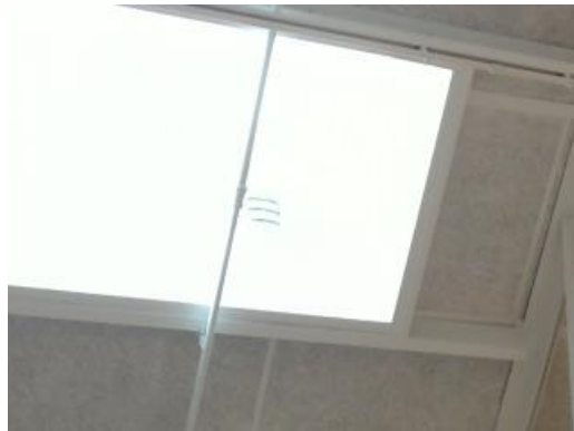
Typical Damaged Skylight
