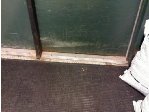
Rusted Entry Doors
