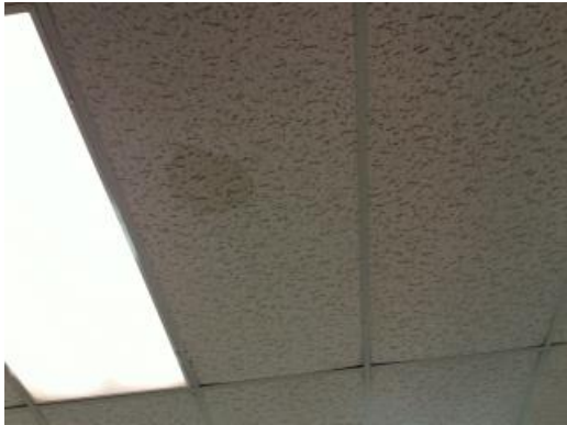
Stained And Sagging Ceiling Tiles
