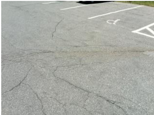
Cracked Asphalt Parking
