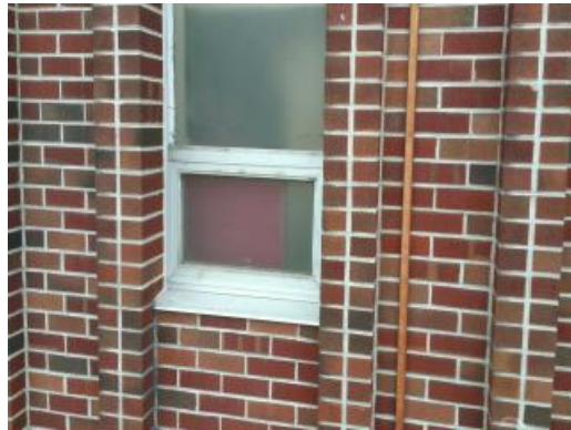
Aged Window With Weathered Seals
