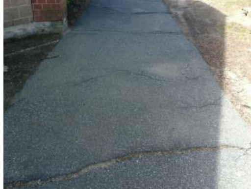
Cracked Asphalt Walkway
