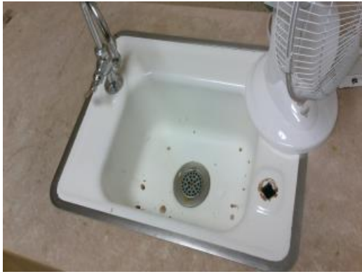
Typical Classroom Lavatory
