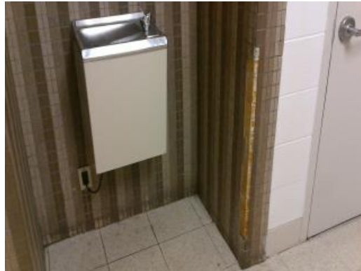
Damaged Ceramic Wall
