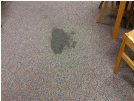
Stained And Worn Carpet
