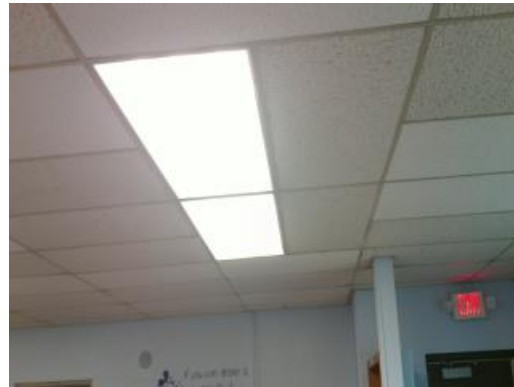
Typical Interior Lights
