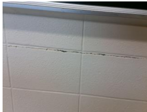
Cracks In CMU
