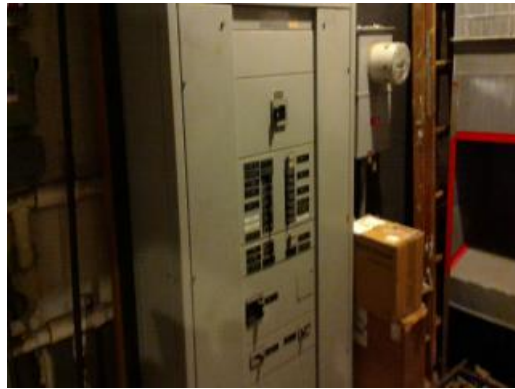
Aged Distribution Panel
