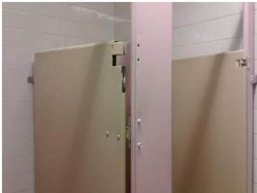
Damaged Toilet Partition
