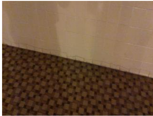
Chipped And Cracked Ceramic Tile Wall
