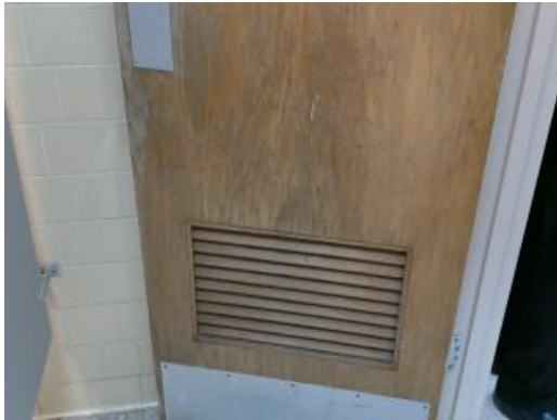
Worn Interior Door
