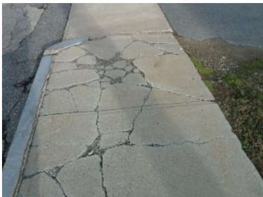
Severely Cracked Sidewalks
