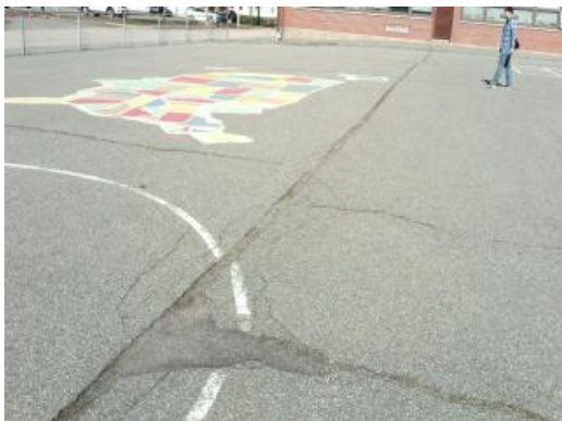
Cracks in Play Area Asphalt
