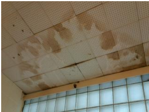
Failing Grid System
