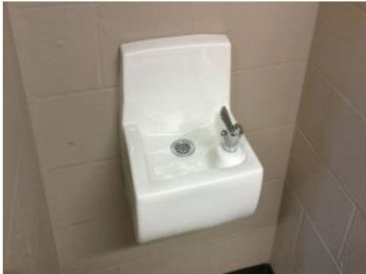
Non-Refrigerated Water Fountain
