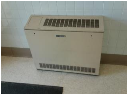
Cabinet Unit Ventilator
