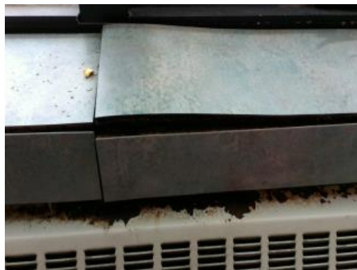
Delaminating Window Ledge
