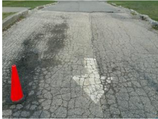
Alligatored Roadway Asphalt
