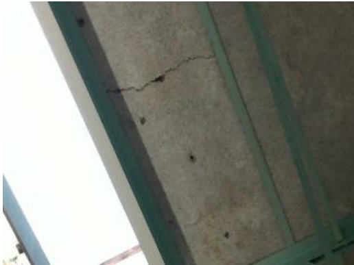
Cracked Tectum Ceiling
