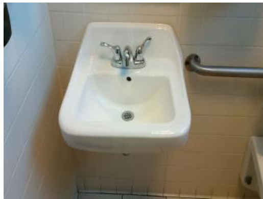
Aged Restroom Lavatory
