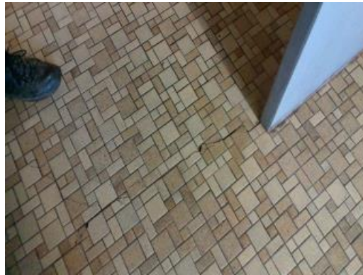
Cracked Ceramic Floor
