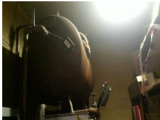
Aged Water Heater
