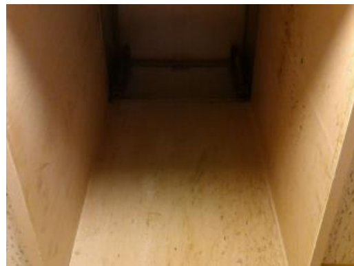
Roof Hatch 20 Feet
