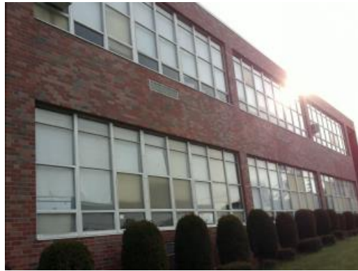
Typical Single Pane Windows
