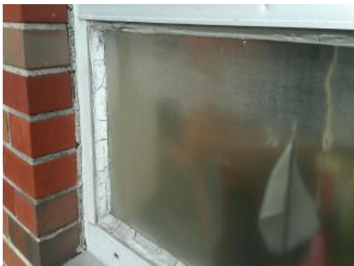
Single Pane Window With Deteriorated Sealant
