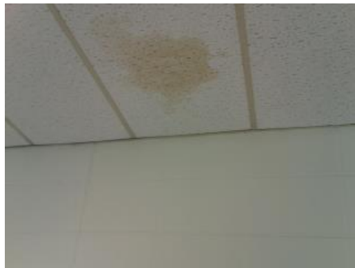
Stained Ceiling Tile
