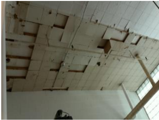
Failing Ceiling Tiles
