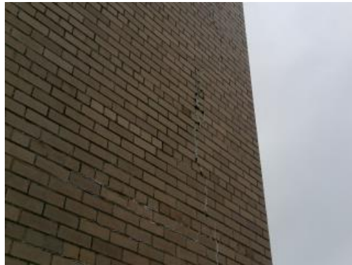
Cracked Exterior Brick
