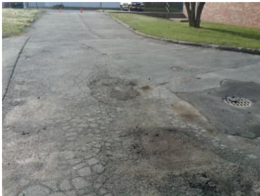
Pot Holes In Asphalt Drive
