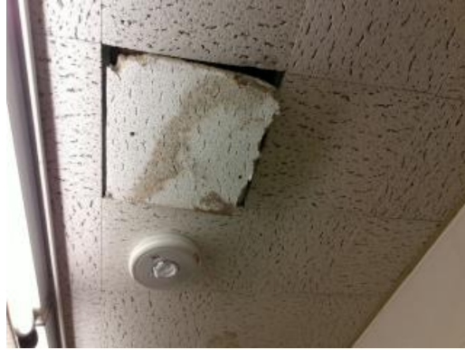
Damaged Ceiling Tiles
