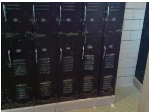
Aged And Rusted Lockers
