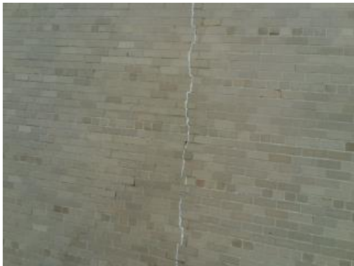
Cracked Exterior Brick
