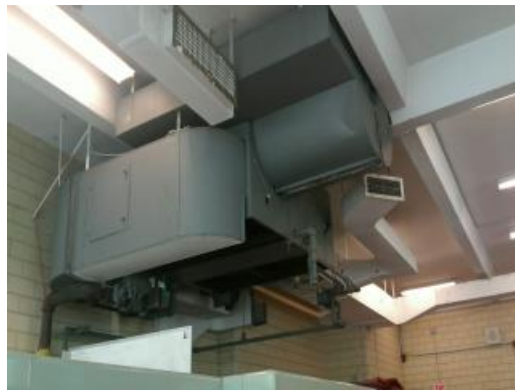
Make Up Air Unit
