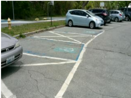
Cracked Parking Lot Pavement
