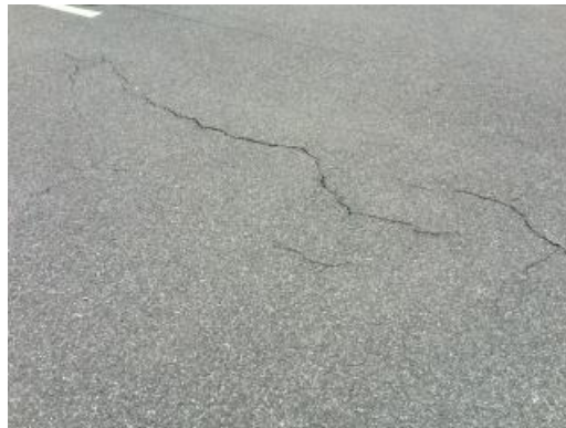
Cracked Asphalt Paving
