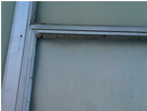
Damaged Aluminum Window
