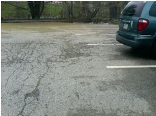
Alligatoring Parking Lot Pavement
