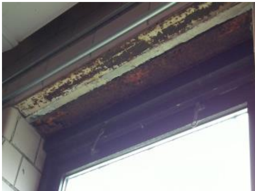
Rusted Steel Lintel
