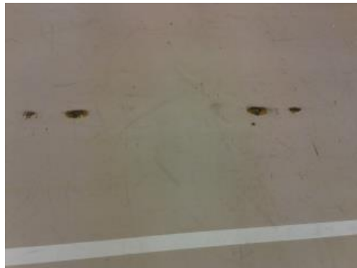
Holes In Sport Flooring
