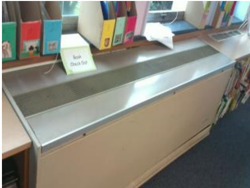
Cabinet Unit Ventilator
