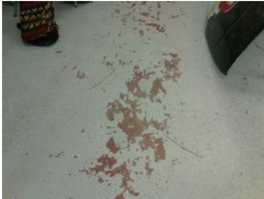
Chipped Concrete Paint
