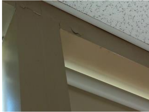
Water Damaged Gypsum Board
