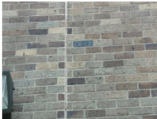
Weathered Expansion Joint Caulking
