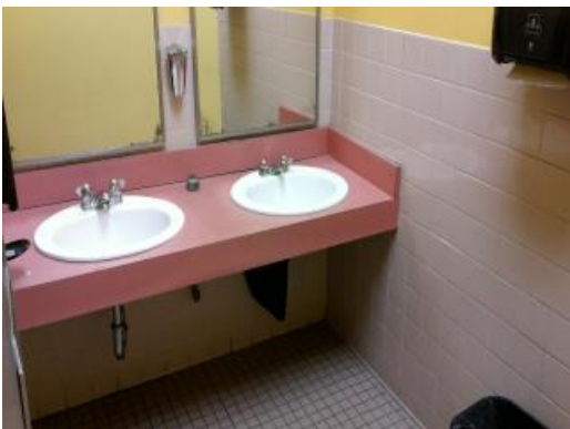
Uninsulated Drain Pipe
