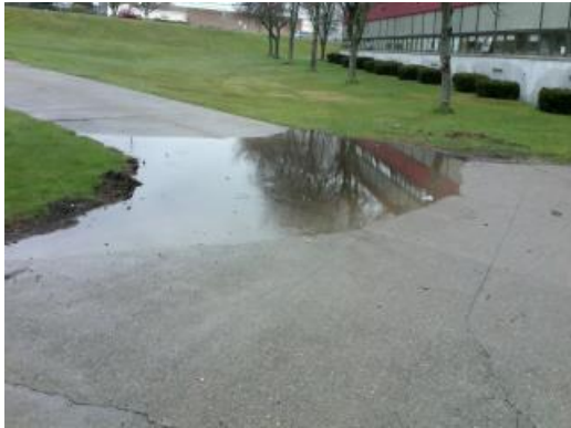
Front Entry Drainage
