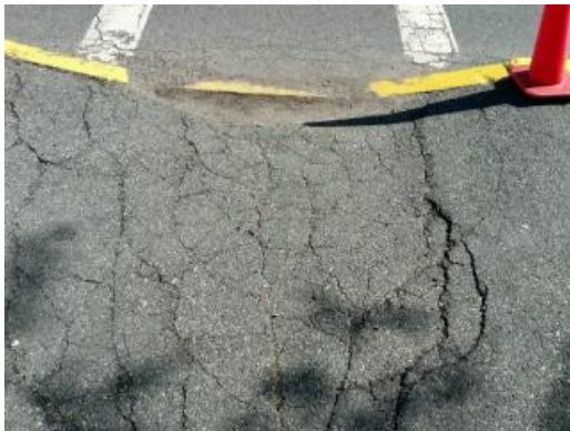
Alligatoring Asphalt Walkway
