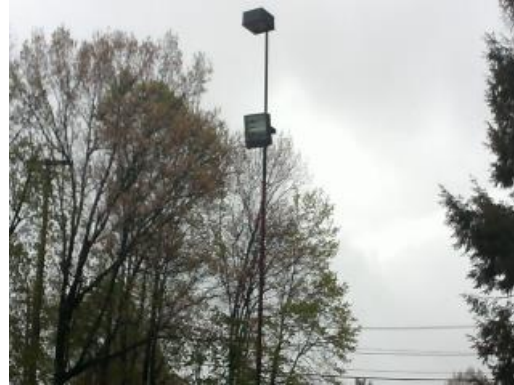
Aged Pole Lighting
