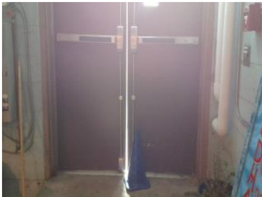
Missing Weather Stripping At Boiler Room Doors
