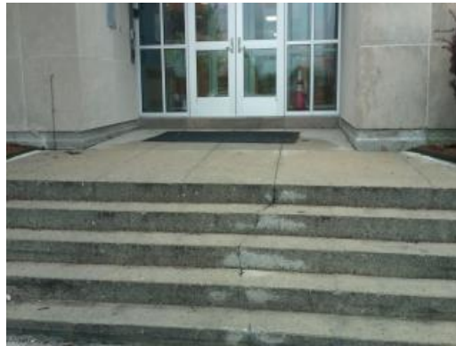
Non-Compliant Front Entrance
