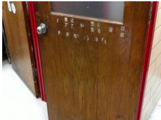
Aged Door And Hardware
