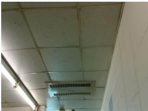
Aged And Stained Ceiling Tiles
