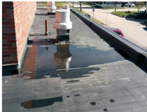
Ponding On Roof
