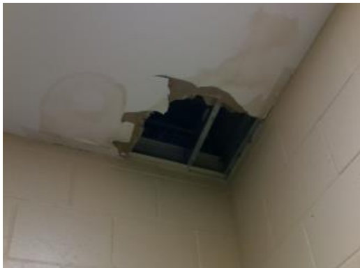
Hole in Ceiling
