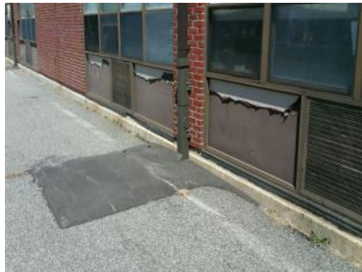
Damaged Metal Panels
