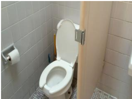
Non-ADA Toilet Stall
