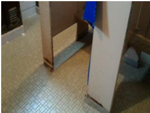
Damaged Toilet Partitions
