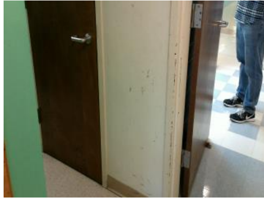
Chipped Wall Paint
