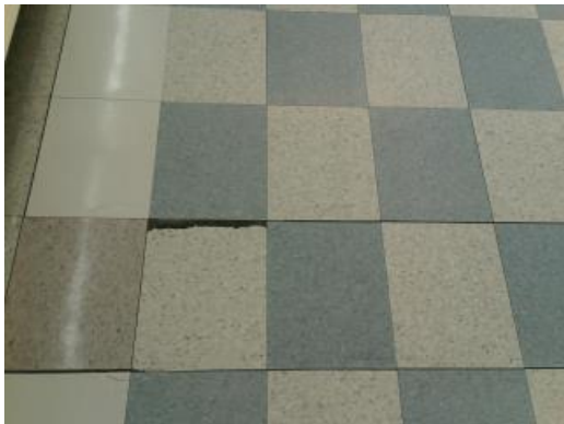
Separating VCT Flooring
