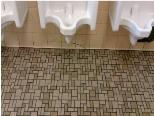
Ceramic Tile Wall Crack
