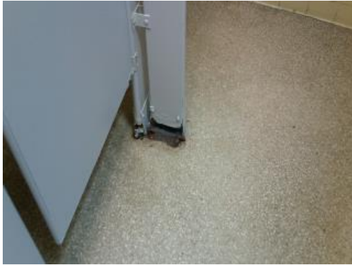
Damaged Toilet Partition
