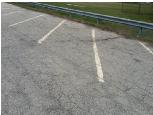
Alligatoring Parking Lot Pavement
