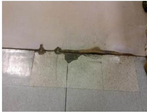
Chipped And Separating VCT
