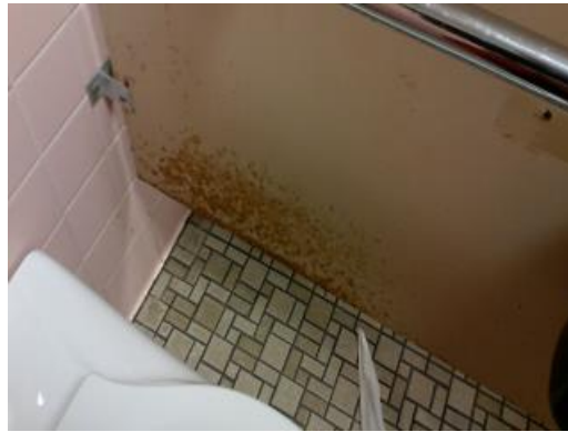
Toilet Partition Damage
