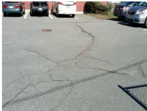
Cracked Asphalt Parking Lot
