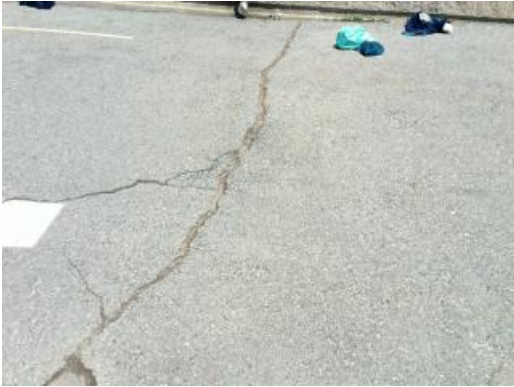
Cracked Paved Play Area
