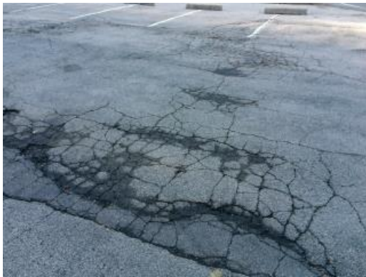
Cracks And Alligating
