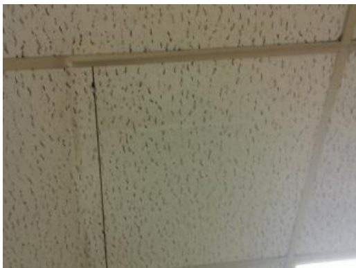
Missing Grid Piece
