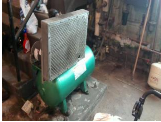
Aged Air Compressor
