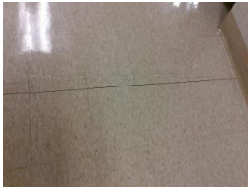
Cracked And Separated Vinyl Tiles
