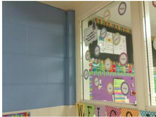
Crack In CMU Wall
