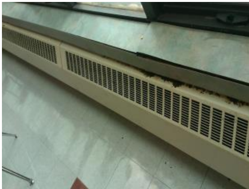
Rusted Finned Tube Radiator
