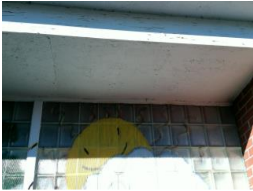
Peeling Paint At Soffit
