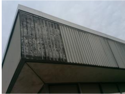
Missing And Damaged Concrete Panels
