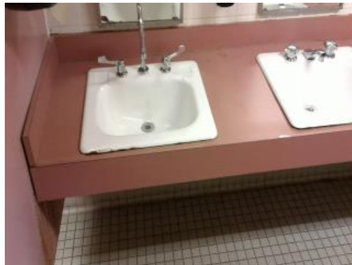
Typical Restroom Lavatories
