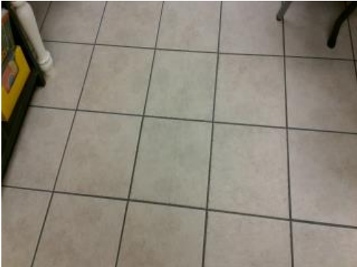
Cracked Ceramic Tile
