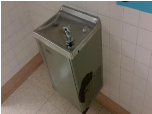
Refrigerated Water Fountain
