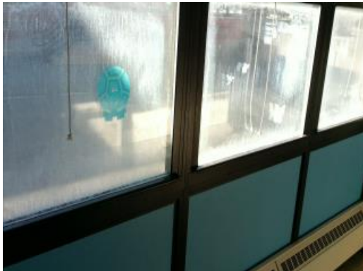
Damaged Window Panes
