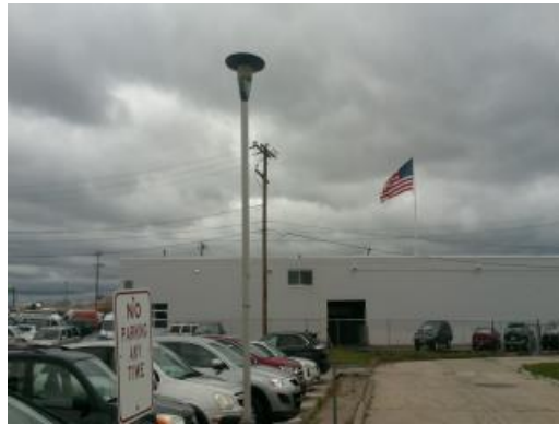
Damaged Pole Lights
