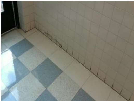
Cracked Ceramic Tile Wall
