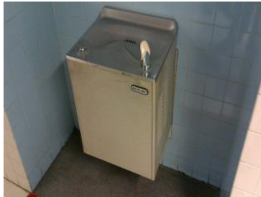
Aged Refrigerated Drinking Fountain
