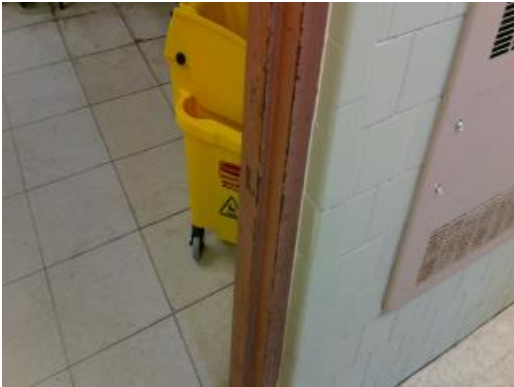
Worn Door Frame Painting
