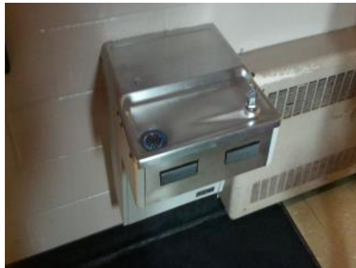
Refrigerated Water Fountain
