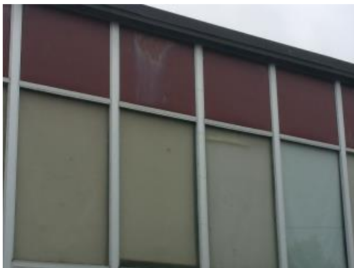
Weathered Metal Panel
