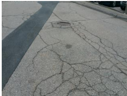
Alligatored Asphalt Roadway
