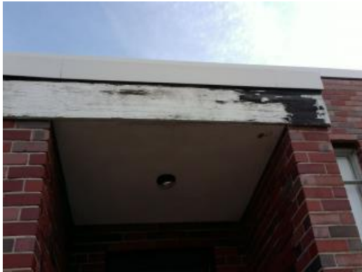
Exterior Soffit Paint
