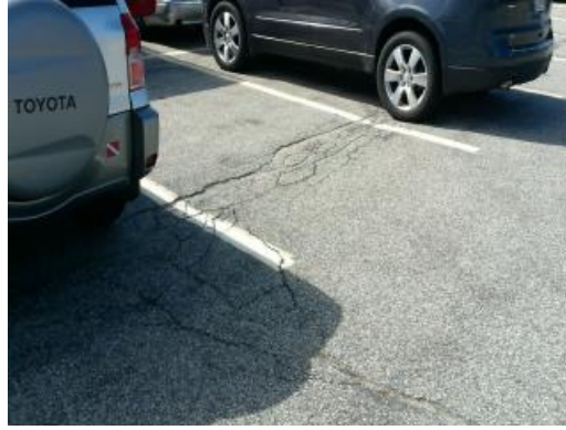
Cracked Asphalt Parking Lot
