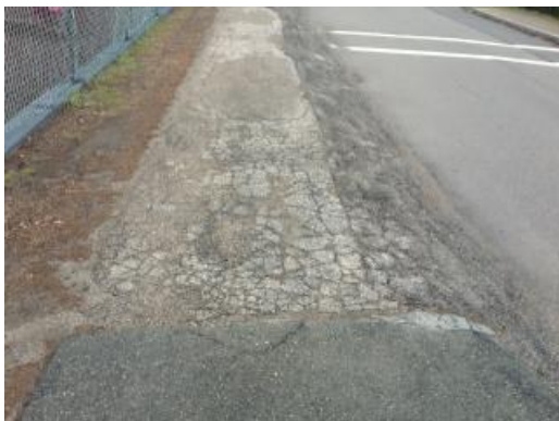
Deteriorated Asphalt Walkway
