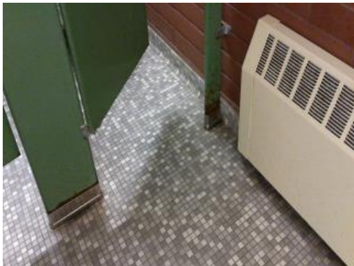
Toilet Partition Damage
