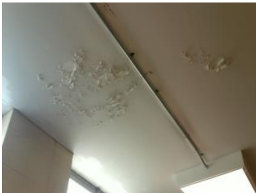
Paint Peeling On Ceiling
