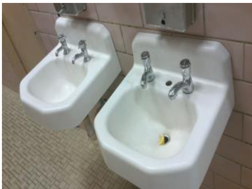
Aged And Stained Restroom Lavatories
