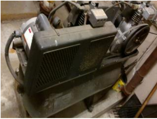
Aged Air Compressor
