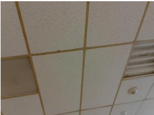
Aged And Stained Grid System
