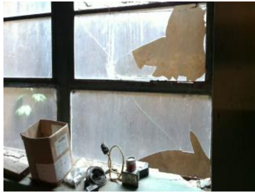
Broken Basement Windows
