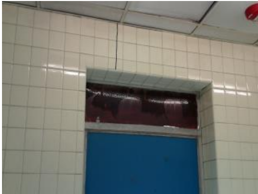
Cracked Ceramic Tile Wall
