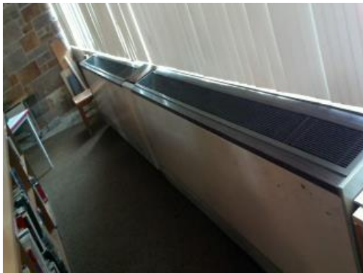
Cabinet Heating Unit
