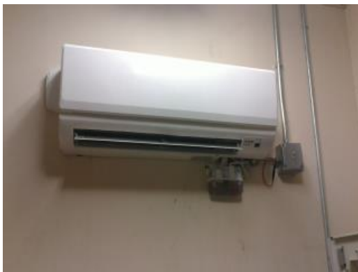
Ductless Split System
