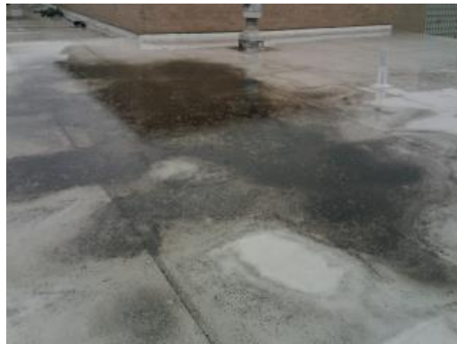
Ponding On Roof
