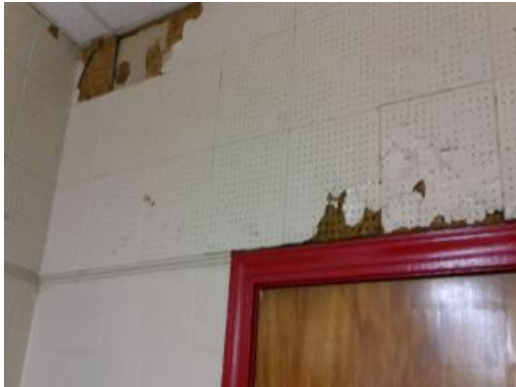
Broken Acoustic Wall Panel
