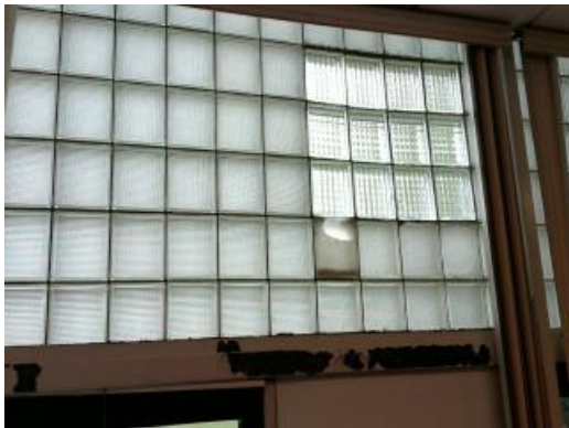
Leaking Glass Block Wall
