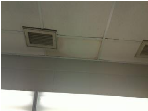
Stained Ceiling Tiles
