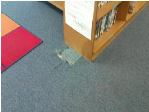
Worn And Frayed Carpet
