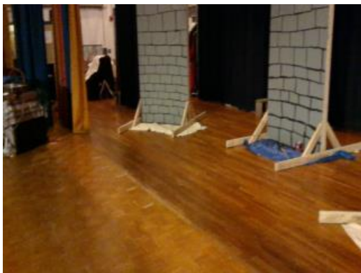
Worn Stage Floor
