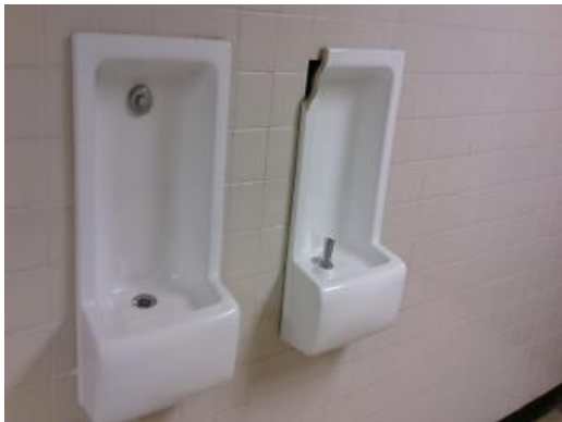
Damaged Drinking Fountain
