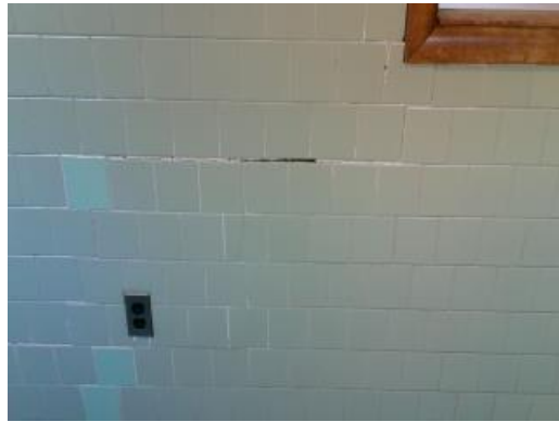
Cracked Ceramic Tile Wall
