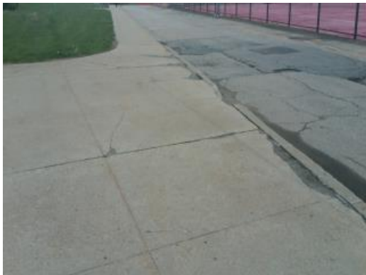
Cracked Concrete Walkway
