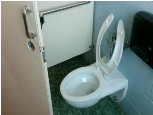
Stall Not Accessible
