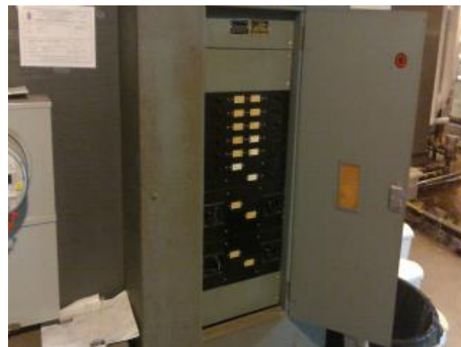
Main Distribution Panel
