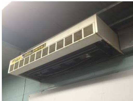
Aged Heating Unit
