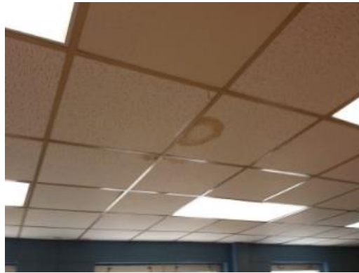
Stained Acoustical Ceiling Tiles
