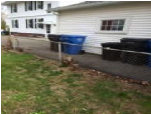
Typical Rusted Fence
