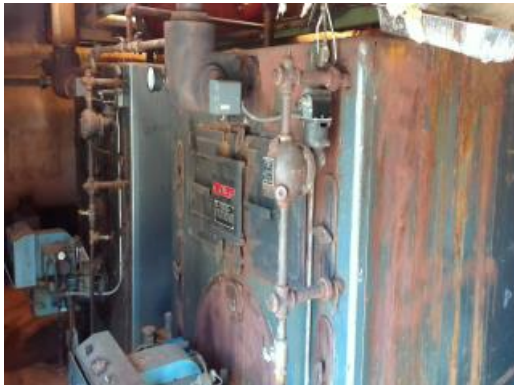
Aged And Corroded Boiler
