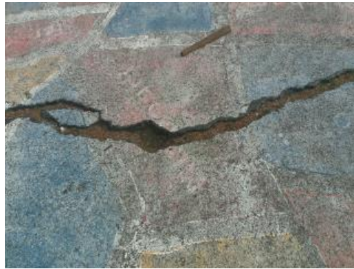
Cracked Asphalt Play Area
