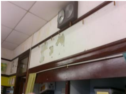
Peeling Wall Paint
