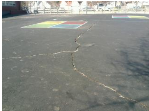
Worn Paved Play Area
