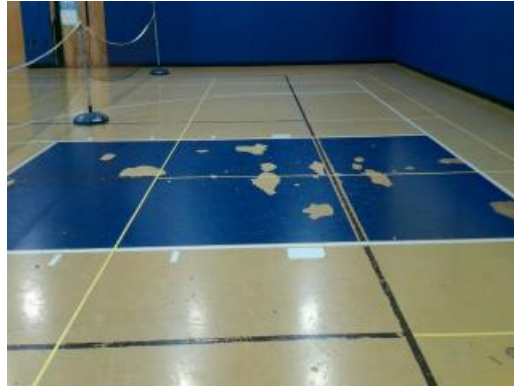
Chipped Gym Floor Paint
