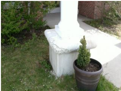
Spalled Column Base
