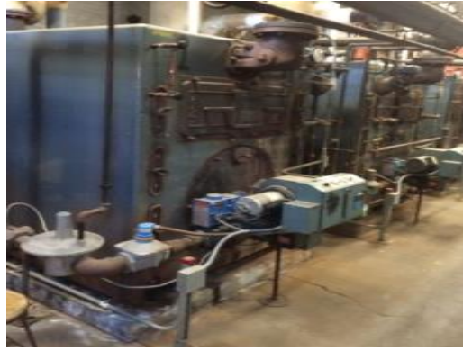
Aged Steam Boilers
