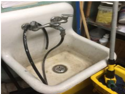
Aged Service Sink
