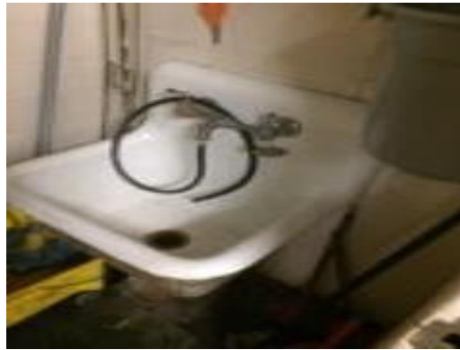
Typical Mop Sink
