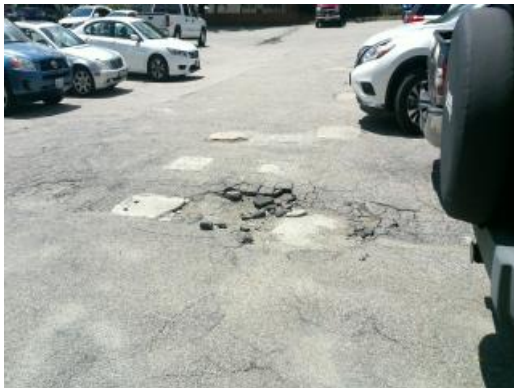
Deteriorated Asphalt Parking
