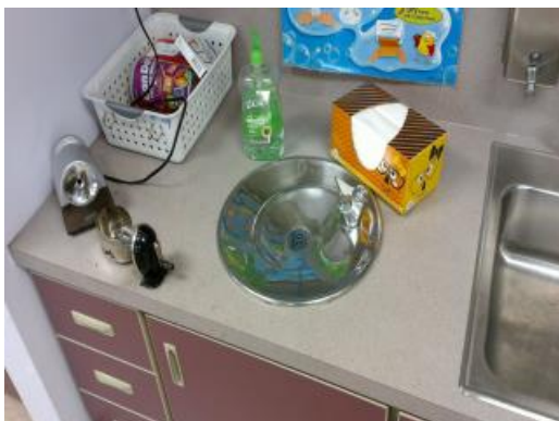
Classroom Drinking Fountain
