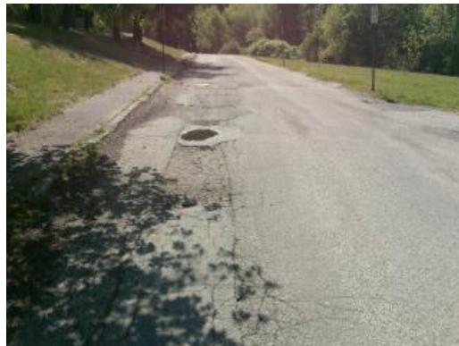
Alligatored Roadway Paving
