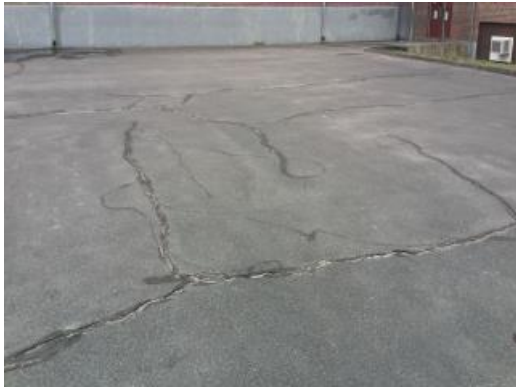
Large Cracks In Play Area Paving
