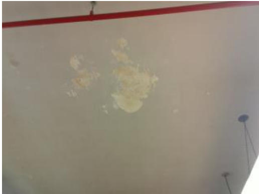
Peeling Ceiling Paint
