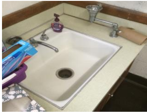
Aged Classroom Sink
