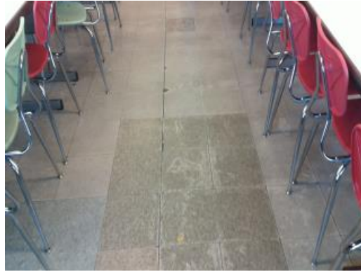
Chipped And Worn VCT
