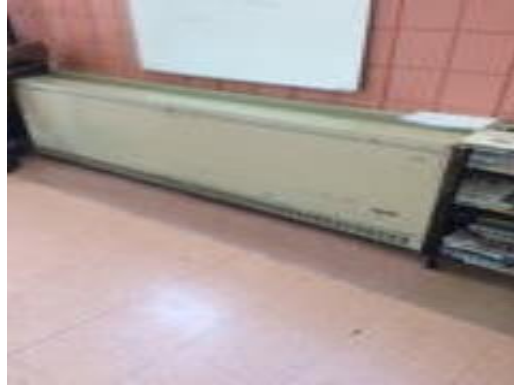
Heating And Ventilating Unit
