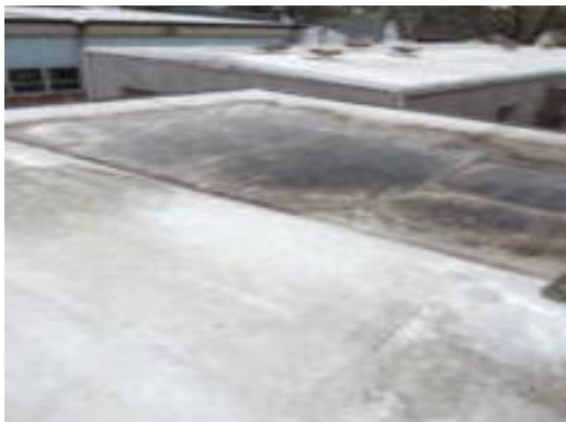
Evidence Of Ponding On Roof
