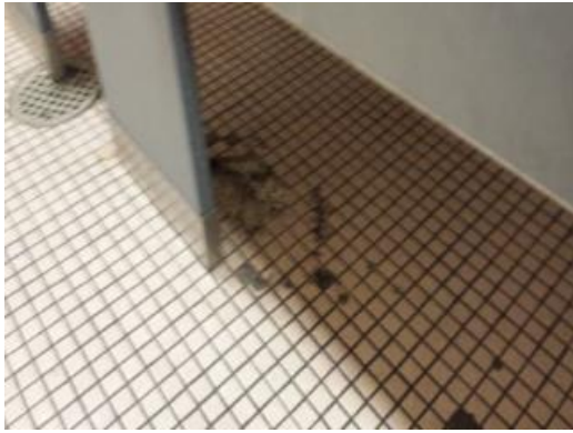
Damaged Ceramic Tile
