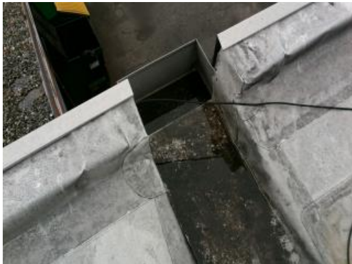
Conductor Box With Debris
