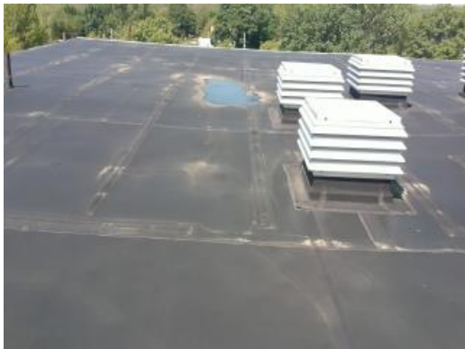
Stained Roof Membrane
