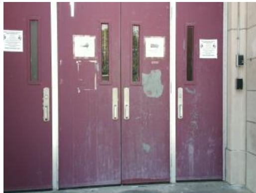
Weathered Exterior Doors
