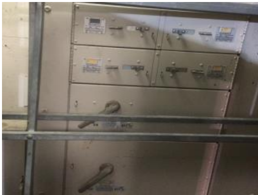
Aged Electrical Distribution
