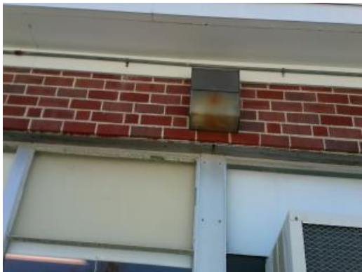
East Side Building Lighting
