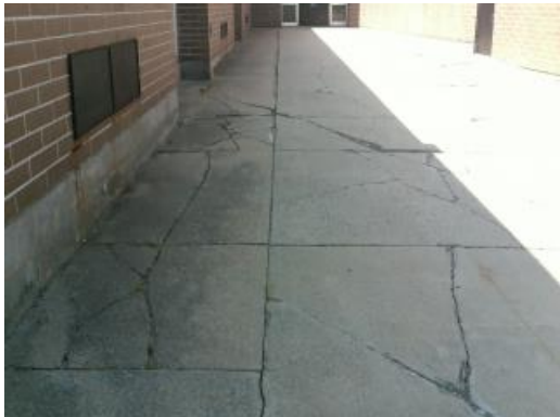
Cracked Concrete Walkway
