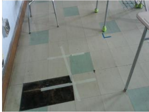
Damaged VCT In Classrooms
