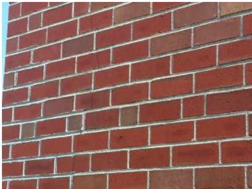
Cracks On Southwest Corner
