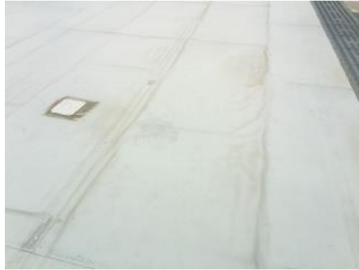
Weathered Gym Roofing
