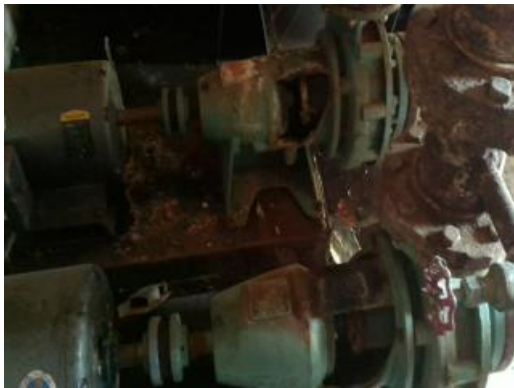
HVAC Circulating Pump
