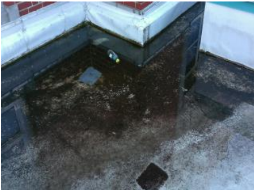
Ponding And Debris On Roof
