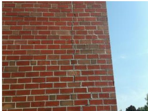
Cracks On Southeast Corner
