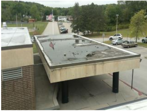
Ponding On Canopy
