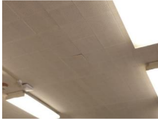
Ceiling Tiles - Falling Down
