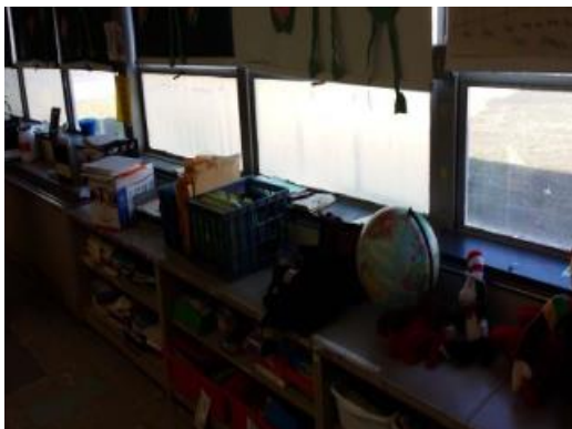
Windows (Broken Seals)
