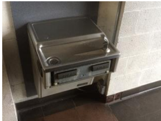
Drinking Fountain Missing Front Casing
