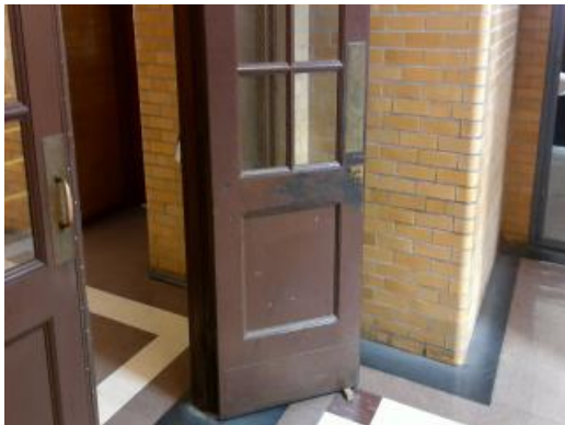
Worn Finish On Interior Door
