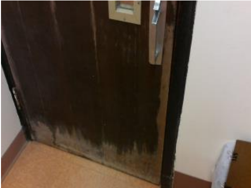
Worn Finish On Wood Door
