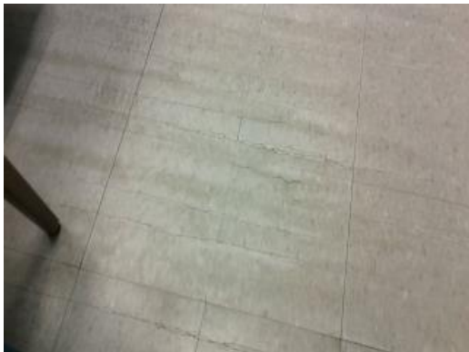
Cracked And Lifting VCT
