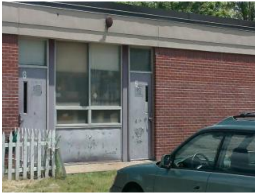
Weathered Exterior Doors
