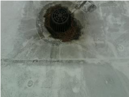
Debris At Roof Drain
