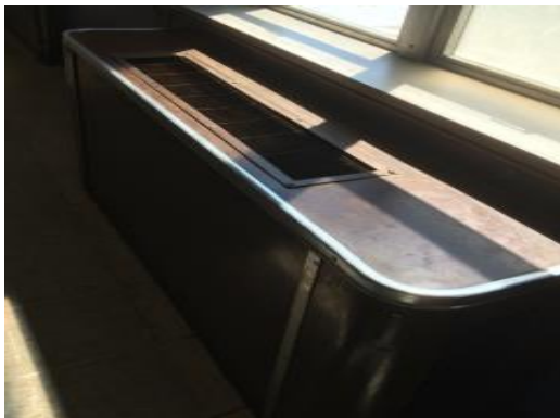
Non-Functional Unit Vent
