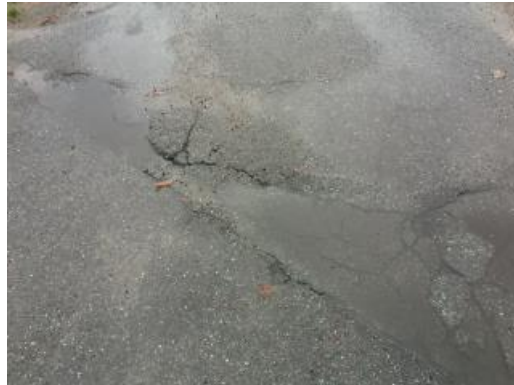
Asphalt Cracks And Potholes
