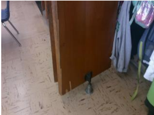
Chipped And Worn Wood Door
