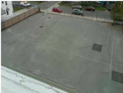
Cracked Play Area
