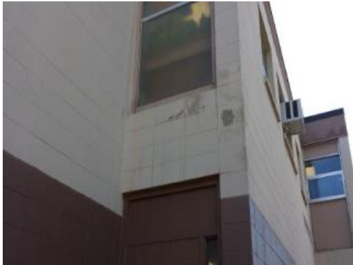
Peeling Exterior Paint
