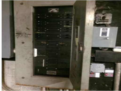
Aged Distribution Panel
