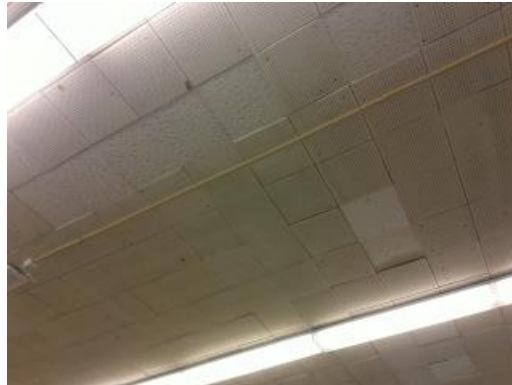
Acoustical Tiles Require Replacement
