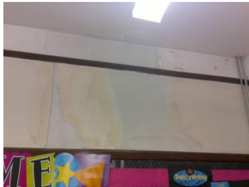
Peeling Classroom Paint
