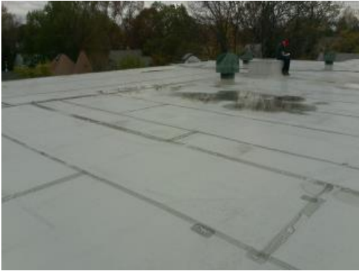
Weathered Roof With Ponding
