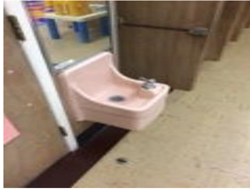
Typical Drinking Fountain
