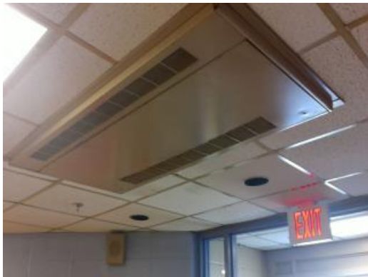
Hot Water Unit Heater
