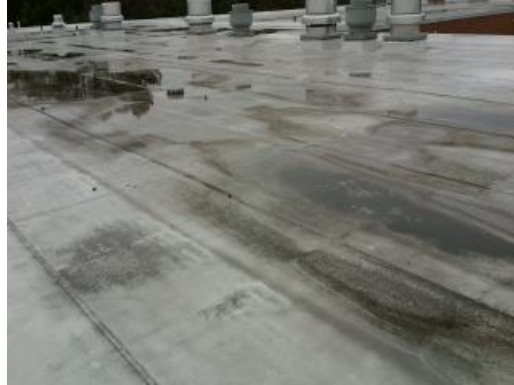
Weathered Roof With Ponding
