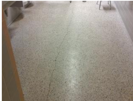
Cracked Terrazzo Flooring
