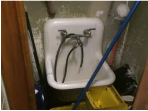
Aged Service Sink
