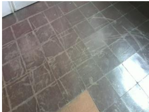
Scratched And Worn VCT
