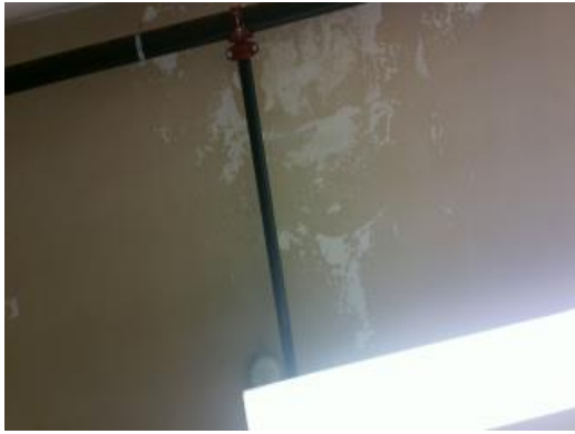
Chipped Ceiling Paint
