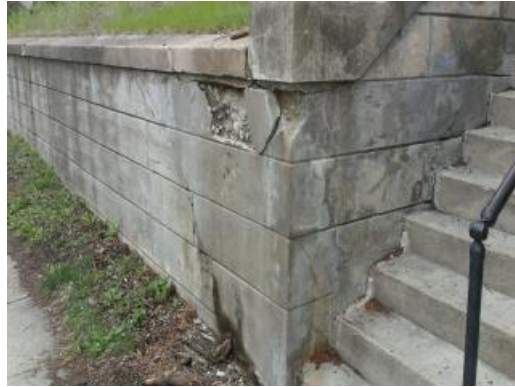
Damaged Retaining Wall
