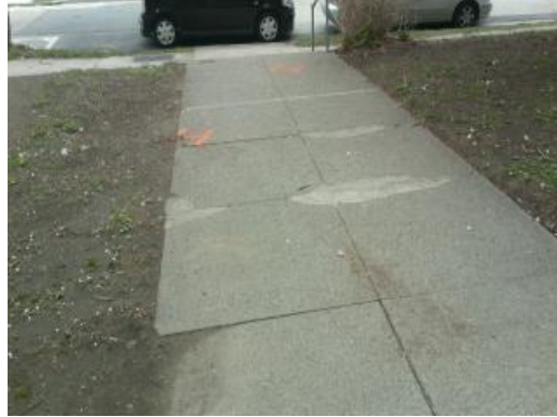
Cracked And Spalled Sidewalk
