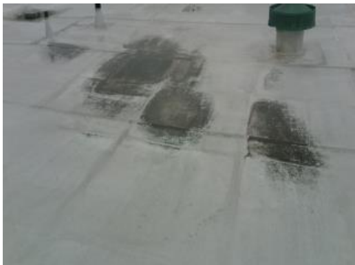
Evidence Of Ponding On Roof
