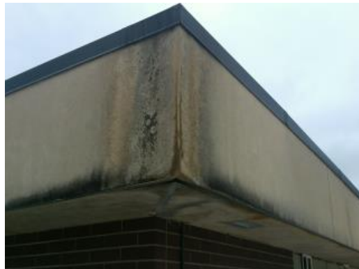
Deteriorated And Stained Stucco
