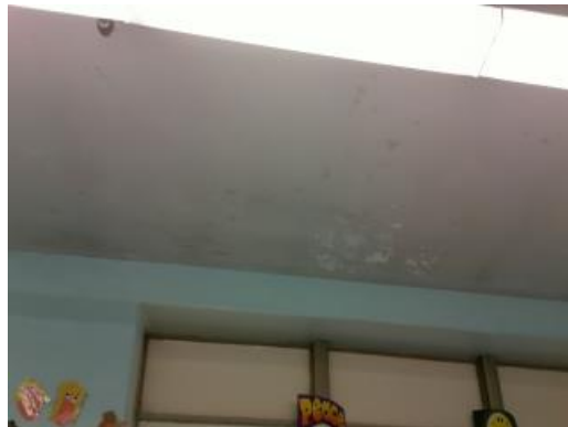
Stained And Peeling Paint
