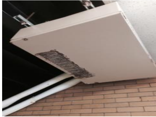
Original Unit Heater
