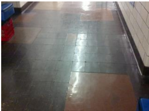
Aged VCT Flooring
