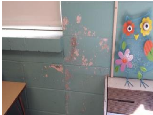
Chipped Interior Paint
