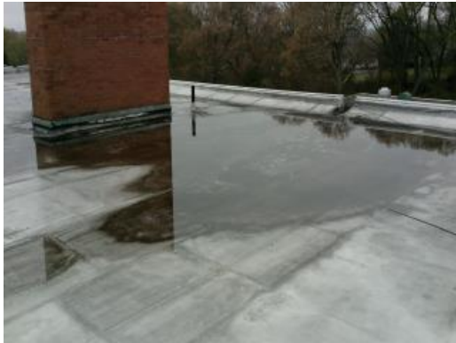
Ponding On Roof
