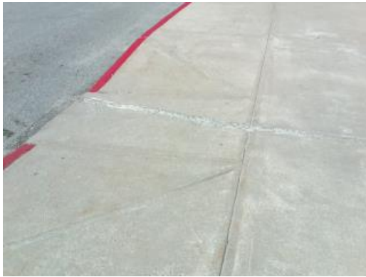
Cracked Concrete Walkway
