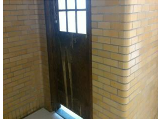
Damaged Wood Door
