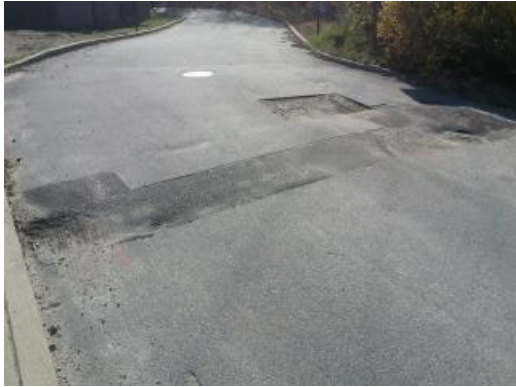
Patched Asphalt Roadway Deteriorating
