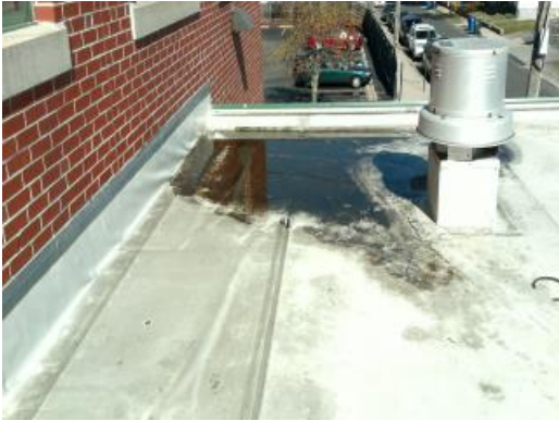
Ponding On Roof
