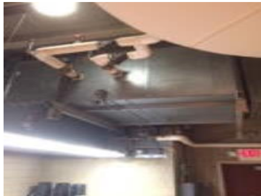
Air Handling Unit
