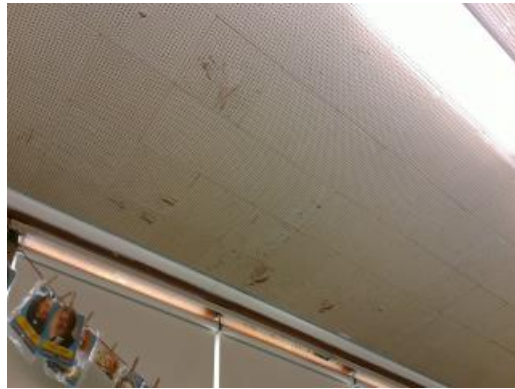
Damaged Ceiling Tiles
