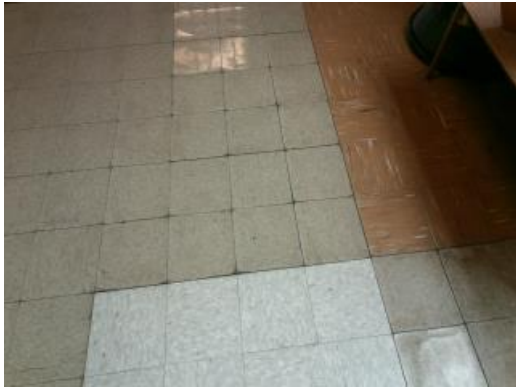
VCT Lifting At Seams
