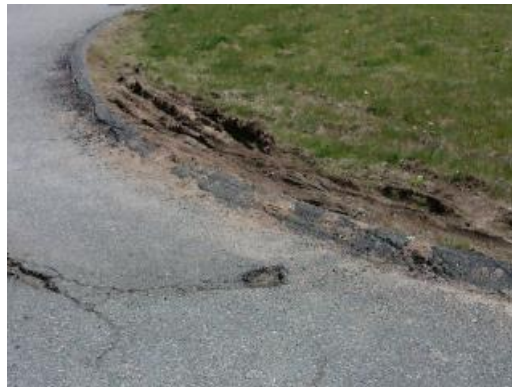
Deteriorated Asphalt Curb
