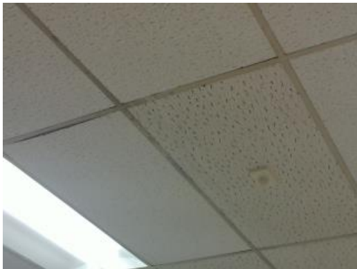
Stained Ceiling Grid
