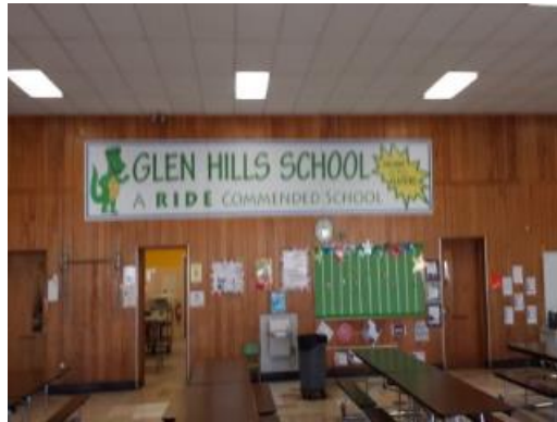
Damaged Wood Panel Wall
