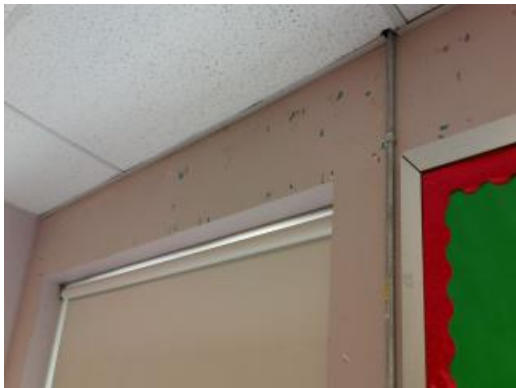
Peeling/chipped Paint Throughout School
