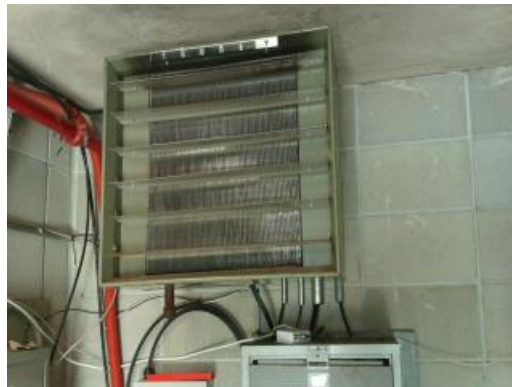
Electric Unit Heater
