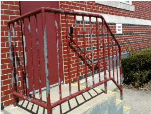
Chipped Handrail Painting
