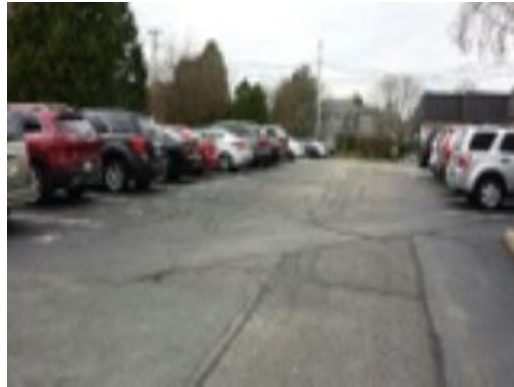
Cracked Asphalt Pavement
