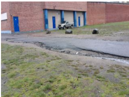
Deteriorated Asphalt Roadway
