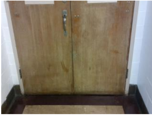
Interior Doors Require Refinishing
