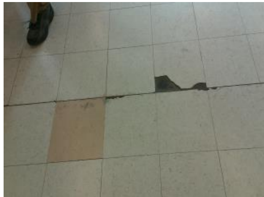
Chipped And Separating VCT Flooring
