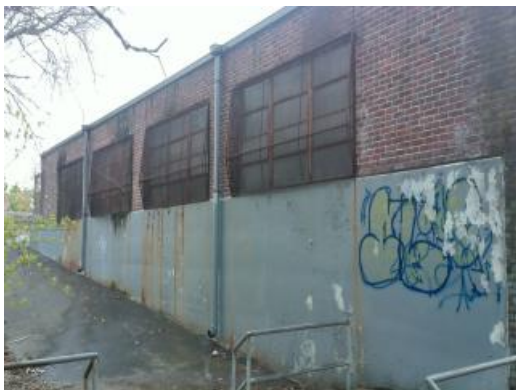
Vandalized Exterior Wall
