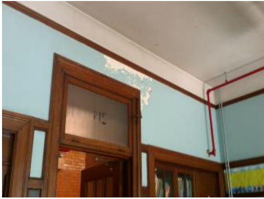
Peeling Classroom Paint
