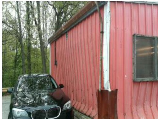
Damaged Metal Facade
