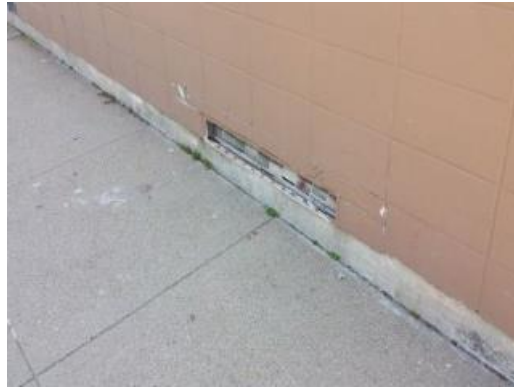
Damaged Exterior CMU
