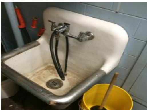
Aged Service Sink
