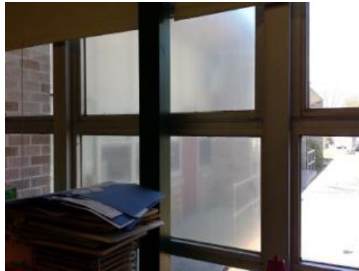
Broken Window Seals
