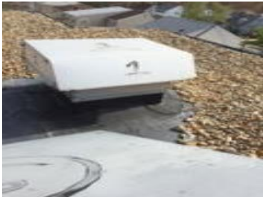
Typical Exhaust Hood
