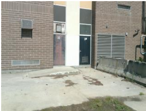
Weathered Exterior Doors
