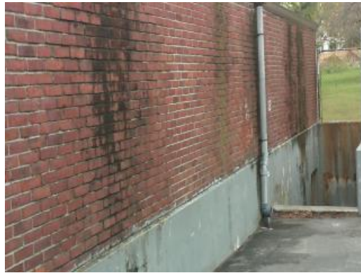
Dirty Exterior Walls
