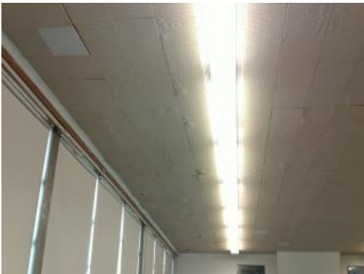
Damaged Ceiling Tiles
