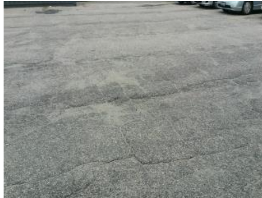
Weathered Roadway Asphalt
