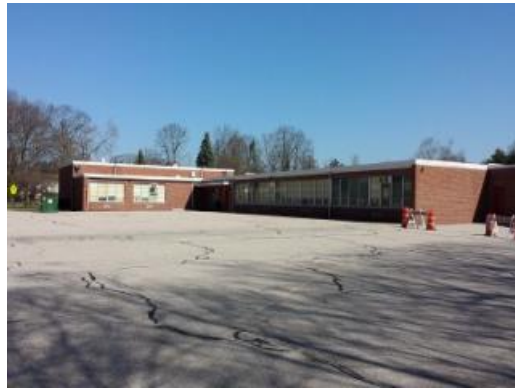
Cracked and Damaged Pavement
