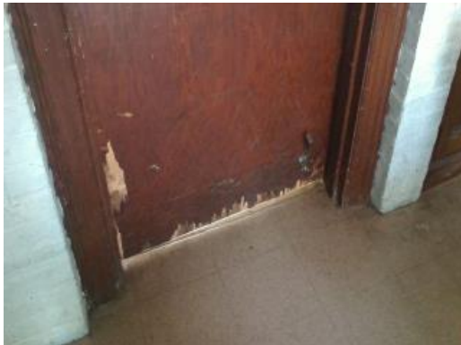
Damaged Interior Door
