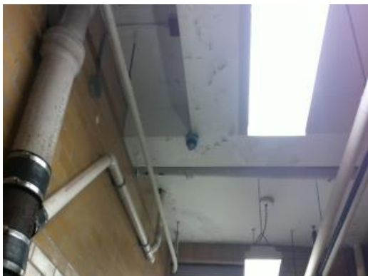
Peeling Ceiling Paint
