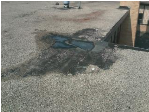
Ponding At Roof Edge
