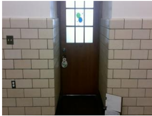
Non-Compliant Door Hardware
