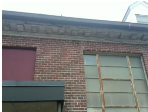
Dentil Molding At Soffit Worn Paint
