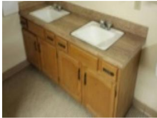
Delaminating Wood Base Cabinet
