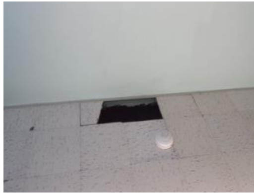
Missing Ceiling Tiles
