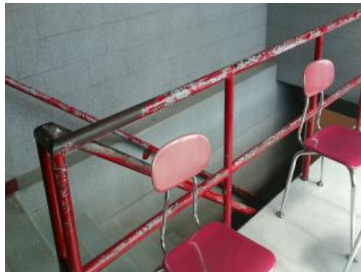
Chipped Handrail Paint
