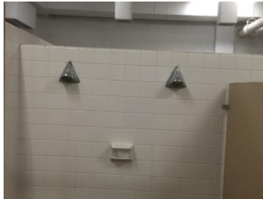
Aged Shower Fixtures
