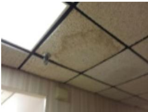
Stained and Sagging Ceiling Tiles
