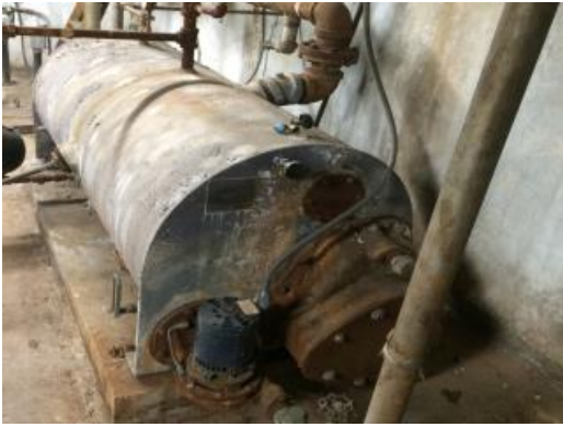
Corroded Condensate Receiver
