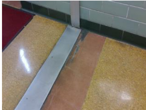
Damaged Corridor VCT
