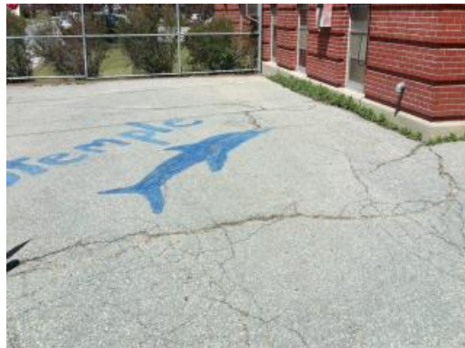
Cracked And Weathered Play Area
