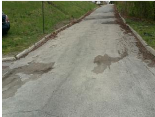
Weathered Asphalt Roadway
