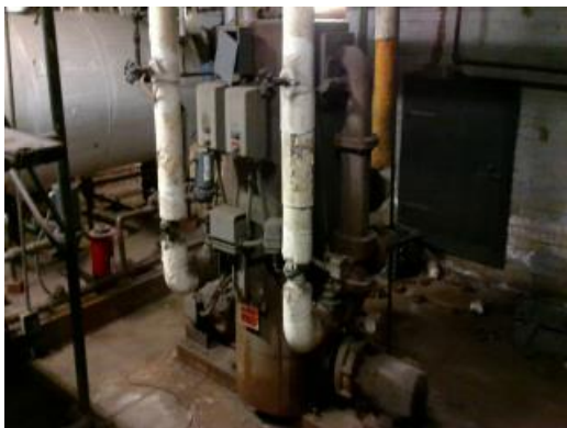
Abandoned Fuel Pump
