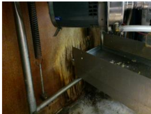
Rotted Wood Panel- Kitchen
