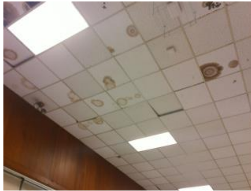
Cafe/Gym Ceiling Tiles
