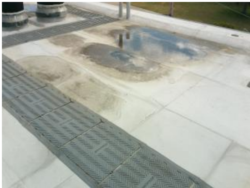
Ponding On Roof
