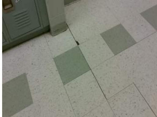
Chipped And Separating VCT
