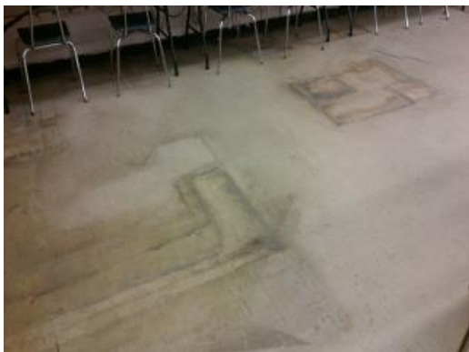
Worn And Stained VCT
