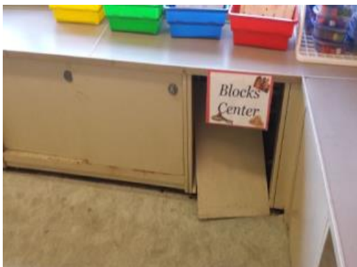
Casework Requires Replacement
