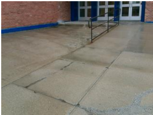
Cracked And Spalled Concrete
