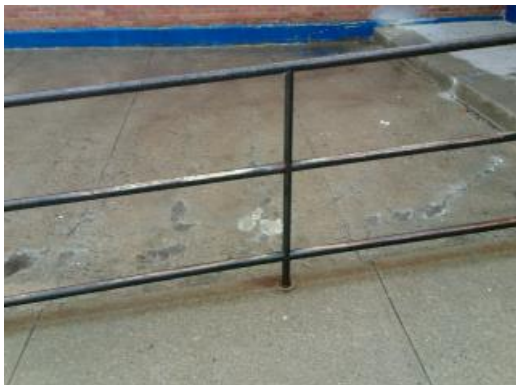
Chipped And Worn Handrail
