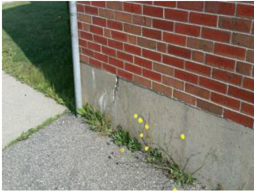
Cracks On Southwest Corner
