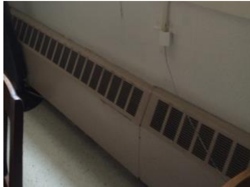
Aged Radiant Heaters
