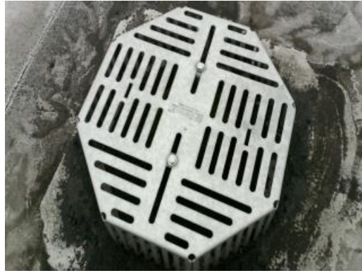
Vegetation In Roof Drain
