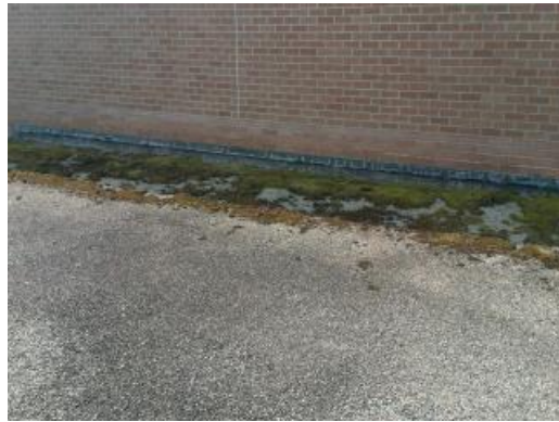
Vegetation Growing On Roof
