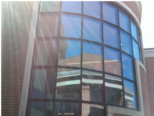
Windows With Broken Seals
