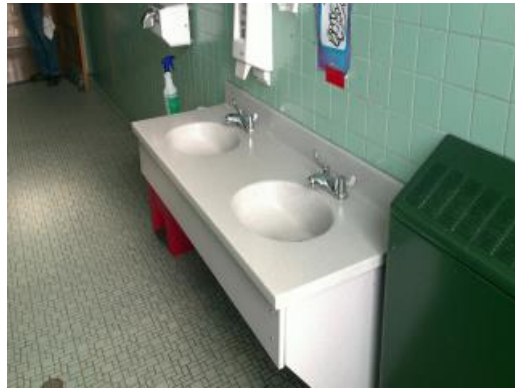
Typical Restroom Lavatories
