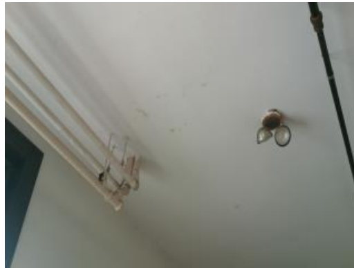
Chipped And Bubbled Ceiling Paint
