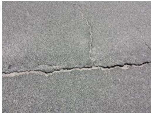
Cracked Parking Lot Pavement
