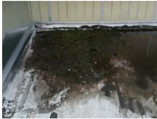
Ponding And Vegetation On Roof
