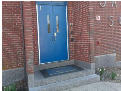
Main Entry Without ADA Access
