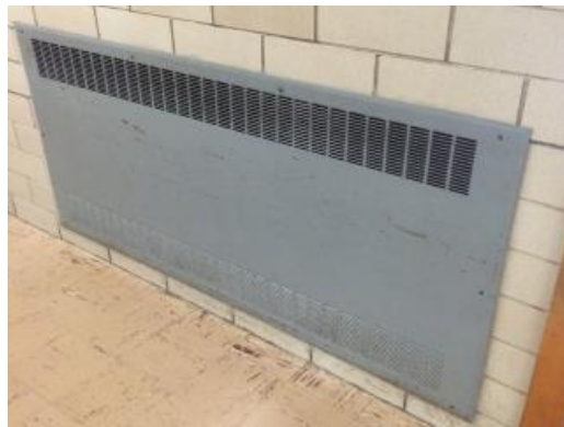
Original Radiant Heater
