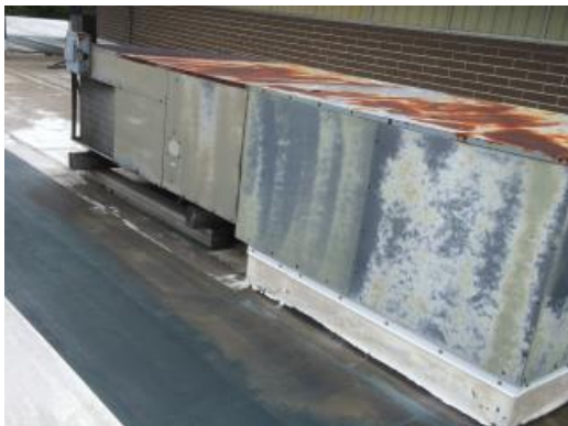
Weathered And Rusted Rooftop Unit
