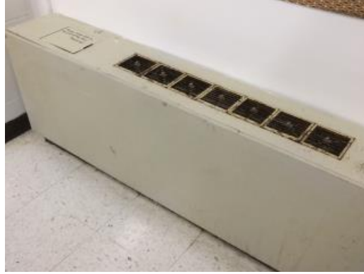
Rusting Unit Heater
