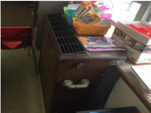
Aged Heating Unit
