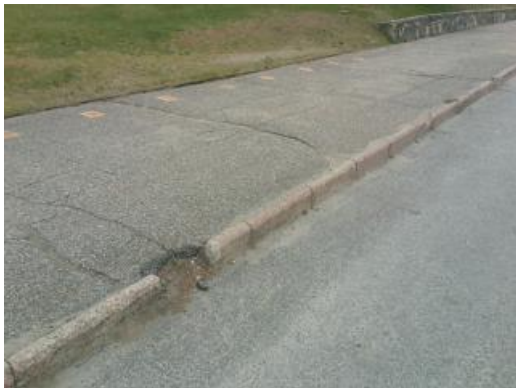
Damaged Curb At Main Entrance
