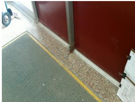
Corroding Storefront Window Frame
