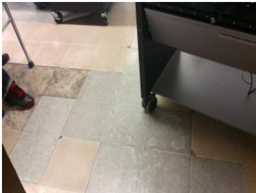
Chipped, Mismatched, And Missing VCT
