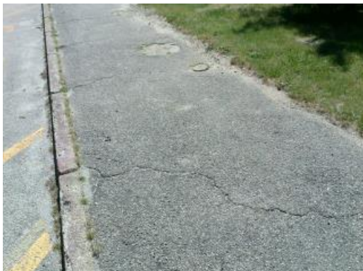
Cracked And Weathered Sidewalk
