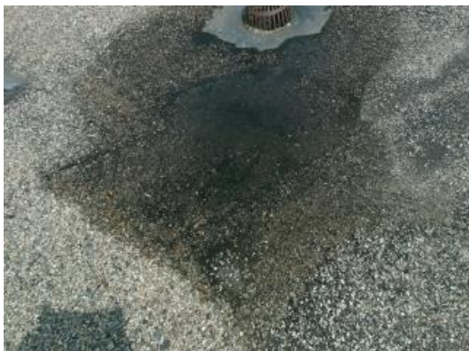
Ponding At Roof Drain
