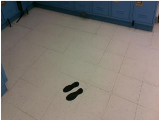
VCT Flooring Lifting At Seams
