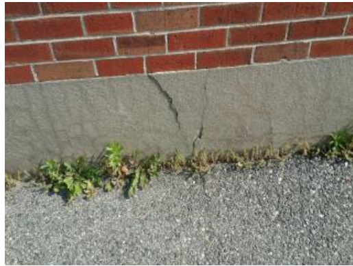
South Wall Foundation Cracks
