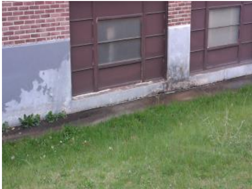
Peeling Exterior Paint
