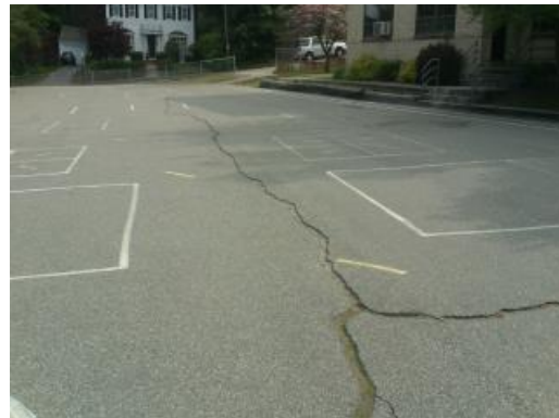
Cracked Play Area
