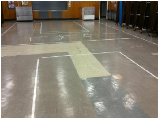
Worn Gymnasium Floor
