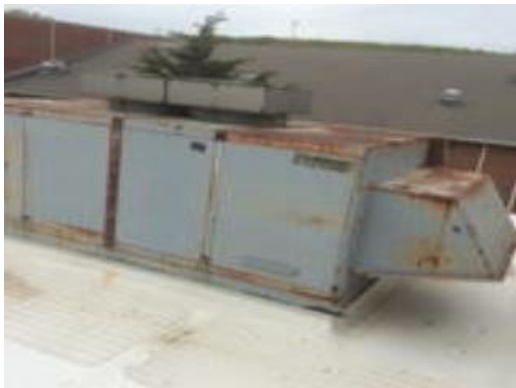
Rusted Roof Top Unit
