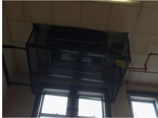
Aged Air Handling Unit
