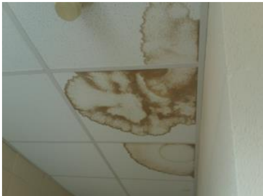
Stained Ceiling Tiles
