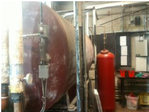
Hot Water Heater
