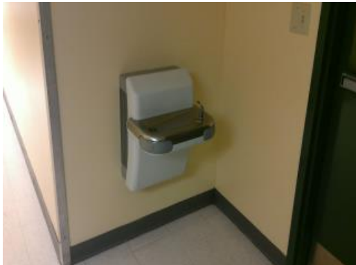
Electric Water Cooler
