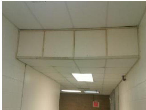
Stained And Warped Ceiling Grid
