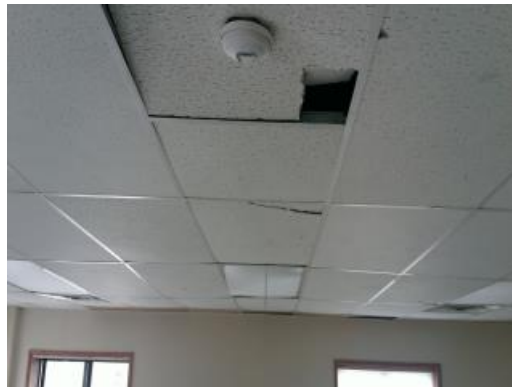
Broken Ceiling Tiles
