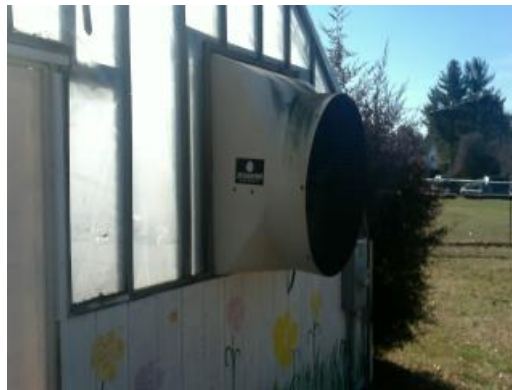
Greenhouse Wall Exhaust
