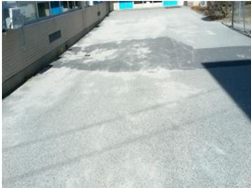
Patched Asphalt Paving
