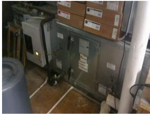
Air Handling Unit
