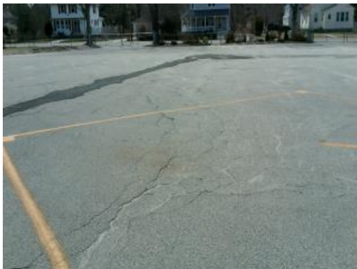
Cracked Asphalt Paving
