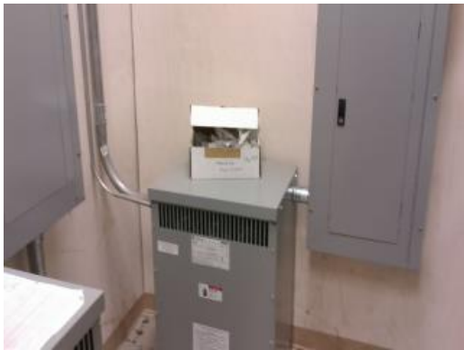
Building 2 Transformer and EPS
