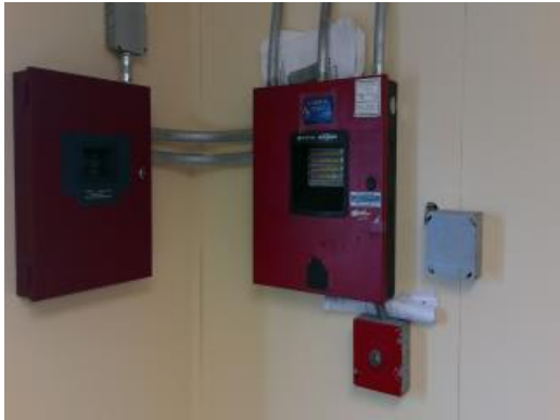
Fire Alarm Panel
