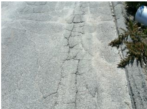
Cracked Asphalt Pavement
