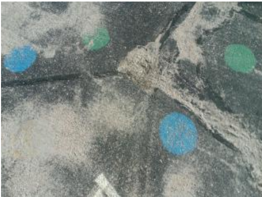
Worn Play Area Paving
