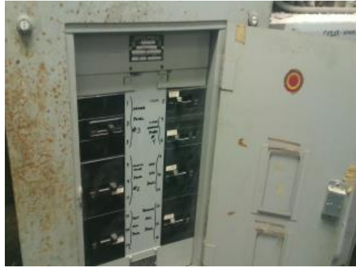
Aged Distribution Panel
