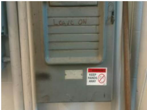
Federal Pacific Electrical Disconnect
