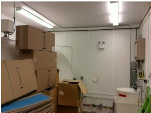
Water Tank Room
