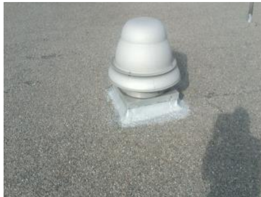
Cracked Flashing At Exhaust
