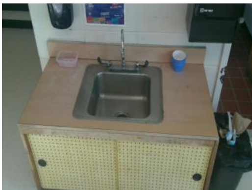
Stained Classroom Lavatory
