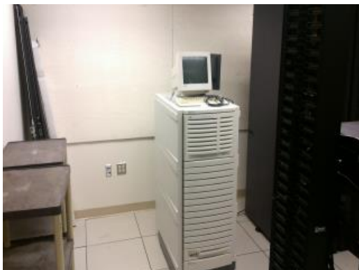
Building 2 Data Server Room
