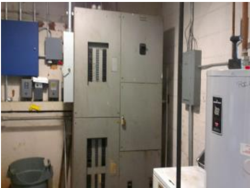
Main Electrical Service
