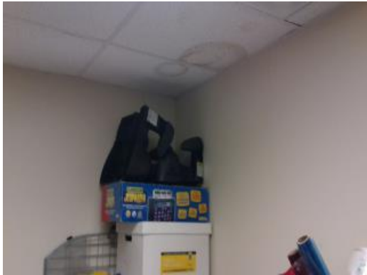
Stained Ceiling Tiles
