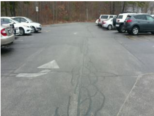
Weathered Asphalt Paving
