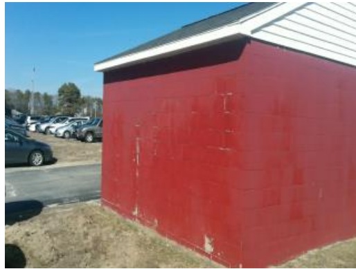
Storage Building Faded Paint
