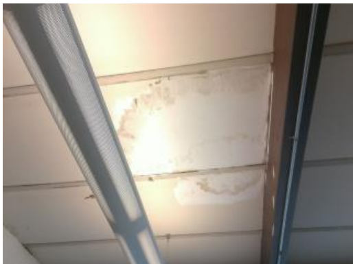
Stained Ceiling Tiles
