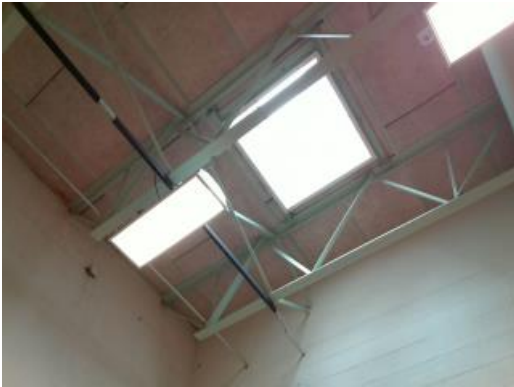
Water Damage At Skylights
