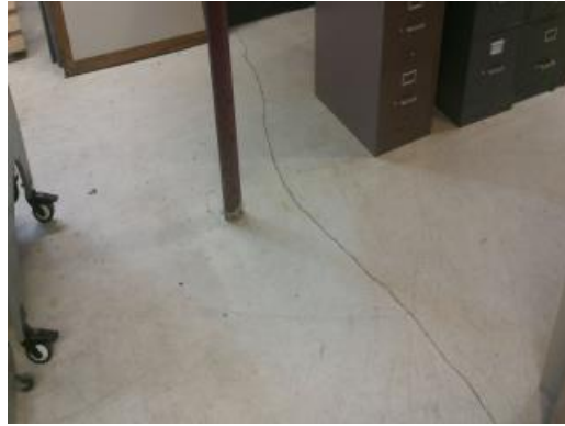
Admin Building Cracked Concrete Floor
