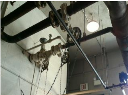
Corroded HVAC Piping
