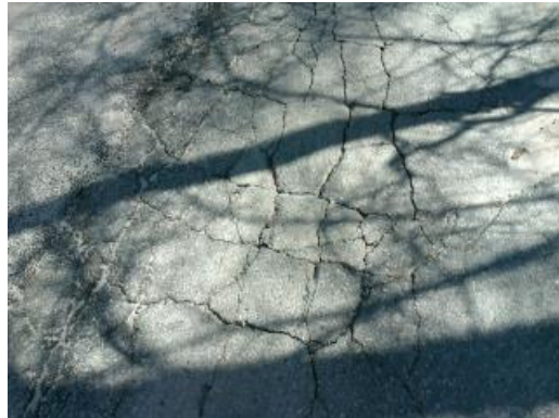
Alligatored Asphalt Pavement
