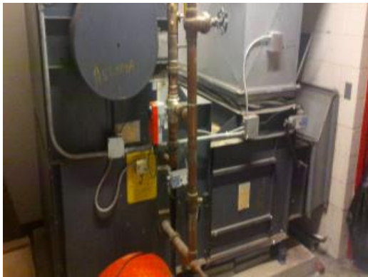
Make Up Air Unit
