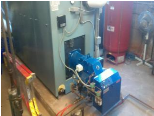
Oil Fired Boiler
