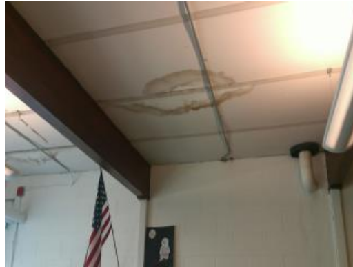
Stained Ceiling Tiles
