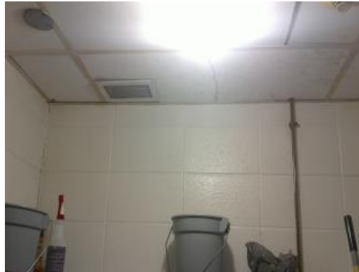
Cracked Ceiling Tile
