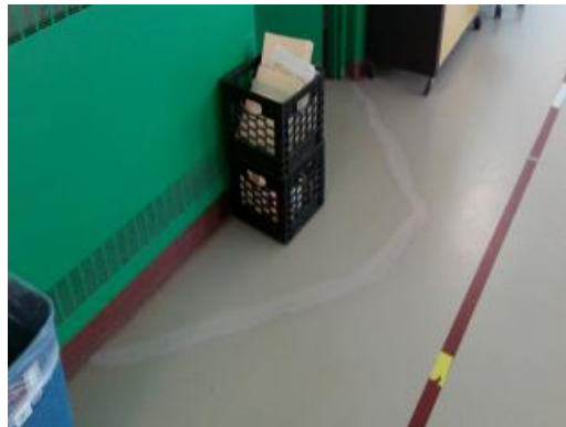
Cracked Athletic Flooring
