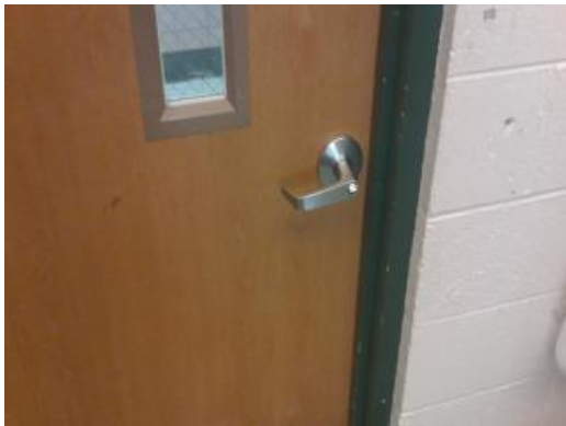
Typical Door Hardware
