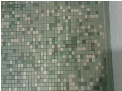
Missing Ceramic Tile
