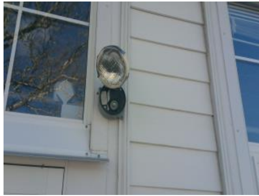
Broken Building Mounted Light
