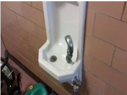
Non-Functional Drinking Fountain
