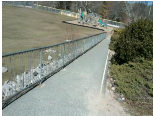
Broken Spindles At Ramp
