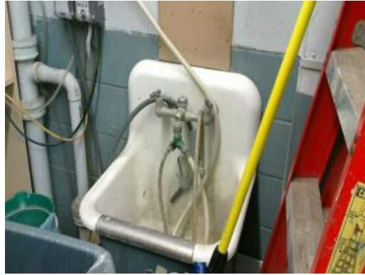
Stained Janitor Sink
