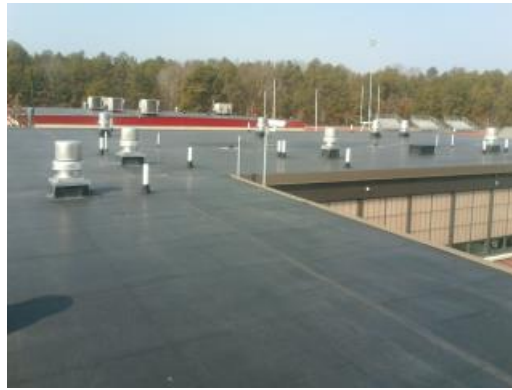
Roof Exhaust Fans
