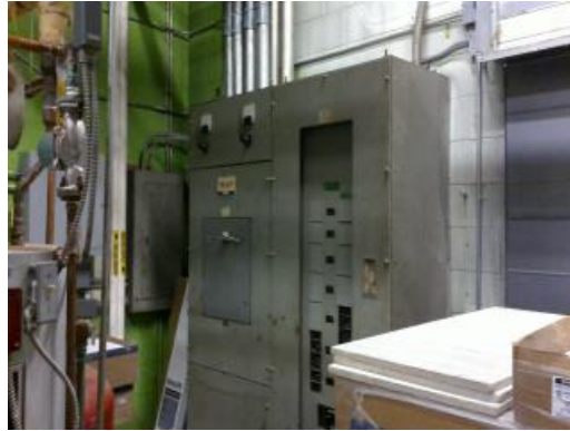
Main Distribution Panel
