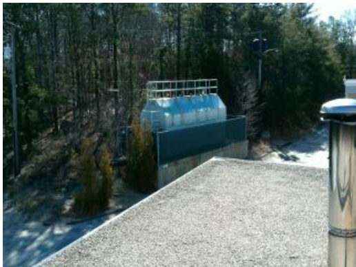
Fuel Storage Tank
