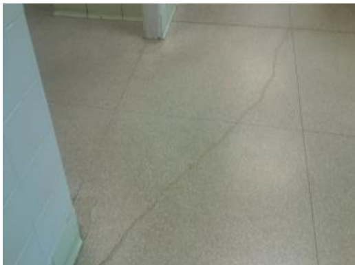
Cracked Terrazzo Floor
