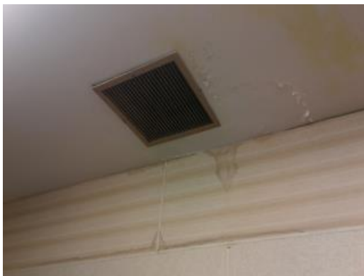
Stained And Peeling Gypsum Ceiling
