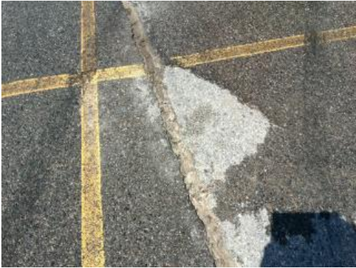
Worn Asphalt Paving
