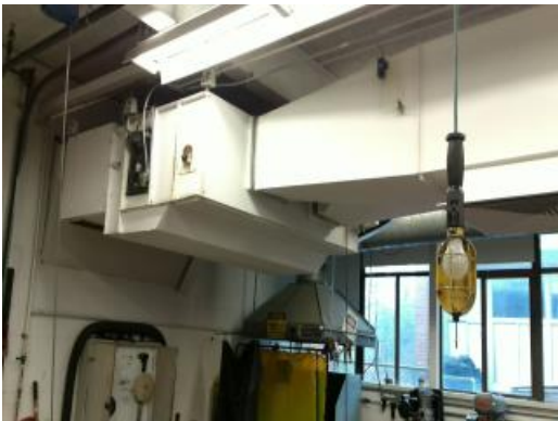
Air Handling Unit
