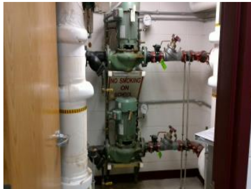
Heating Hot Water Circulating Pumps
