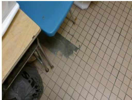
Damaged Ceramic Tile
