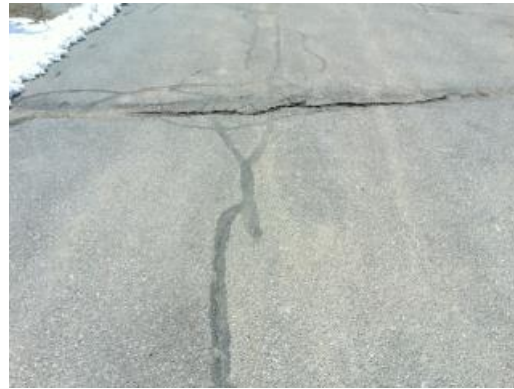
Parking Lot Damage
