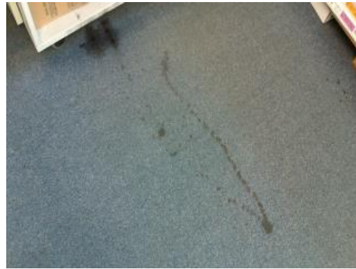
Worn and Stained Carpet
