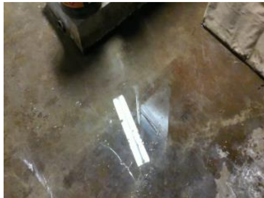
Flood in Boiler Room
