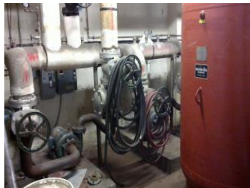
Heating Hot Water Circulating Pumps
