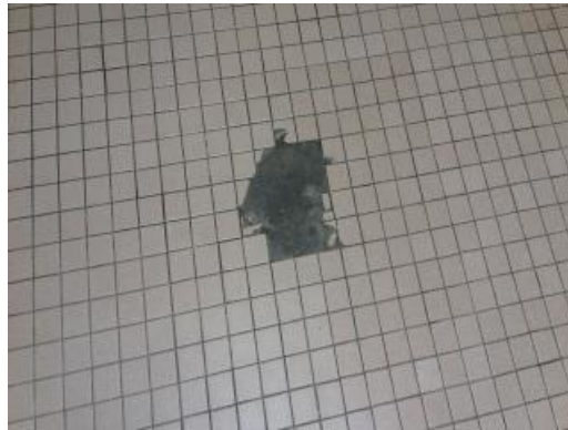
Damaged Ceramic Tile
