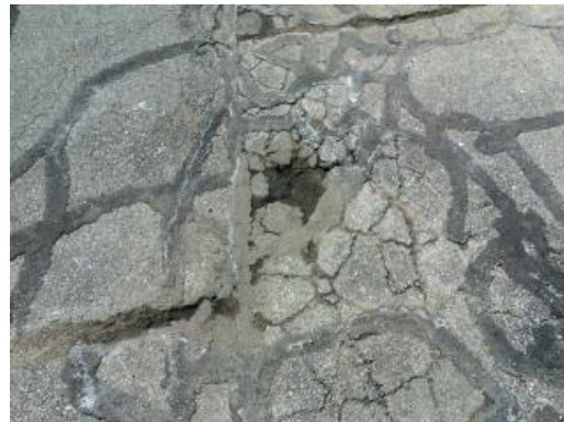
Parking Lot Damage
