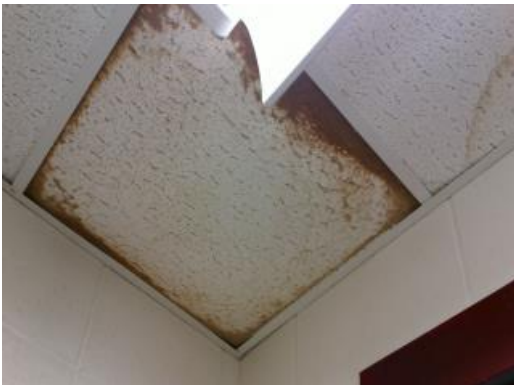
Stained Ceiling Tile
