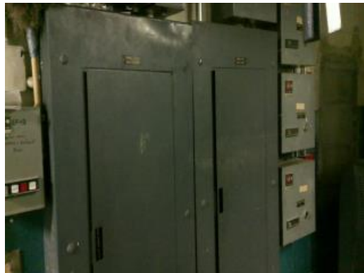
Electrical Panel Board
