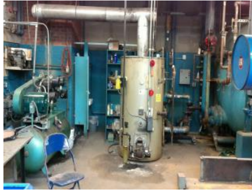
Domestic Hot Water Heater and Air Compressor
