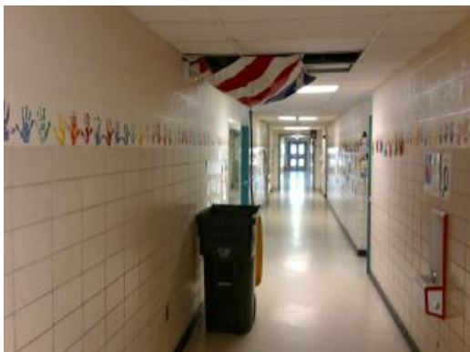
Roof Leak Damage To ACT
