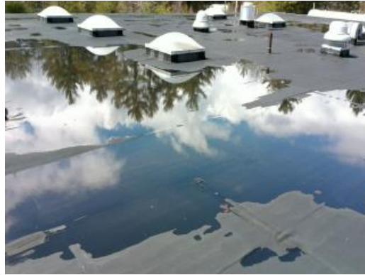
Ponding On Roof
