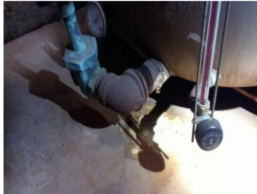
Leakage And Corrosion At Steam Condensate Receiver
