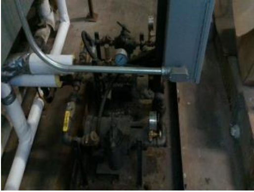
Fuel Oil Pumps
