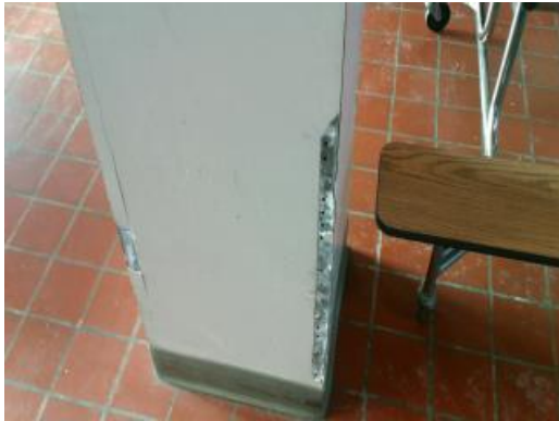
Damaged Gypsum Board
