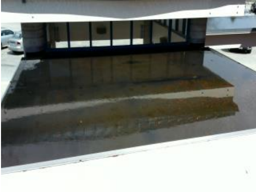
Ponding On Roof
