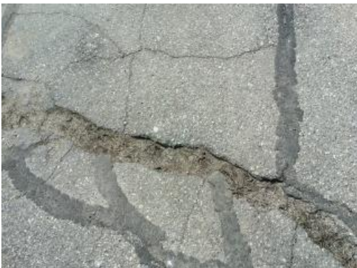
Parking Lot Damage
