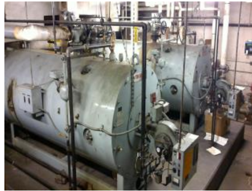
Heating Hot Water Boilers
