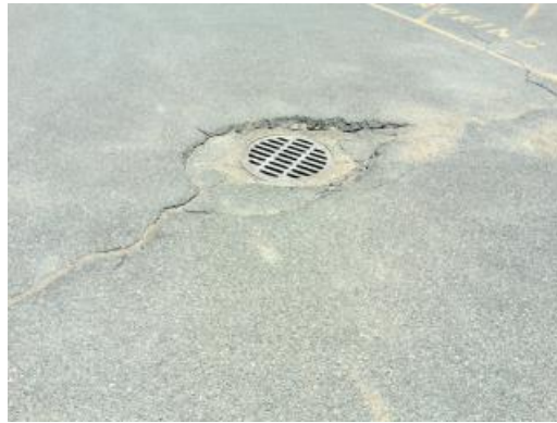
Parking Lot Damage
