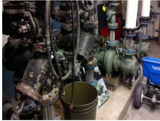
Heating Hot Water Circulating Pumps
