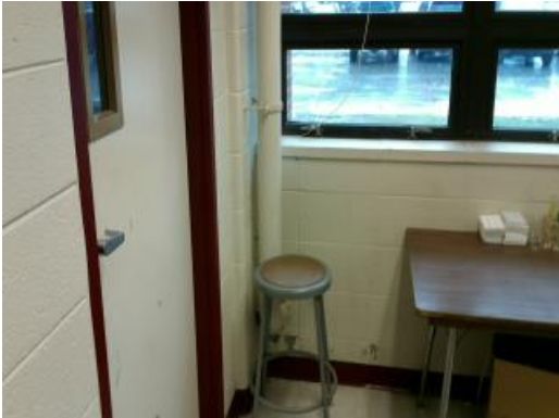
Non-Insulated Storm Drain Piping
