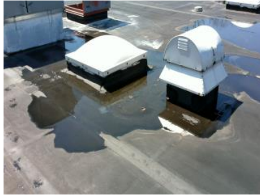
Roof With Ponding
