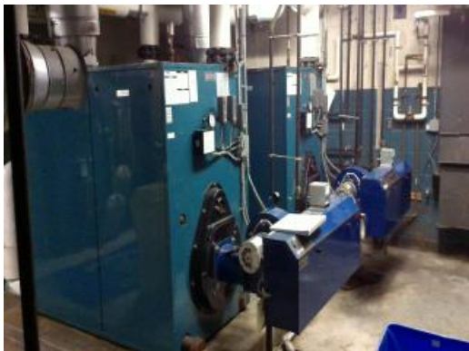
Heating Hot Water Boilers
