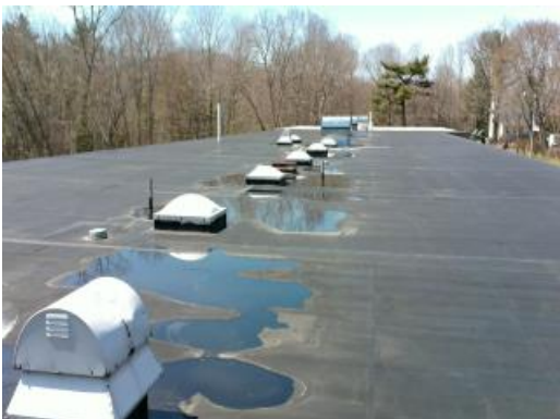
Roof With Ponding
