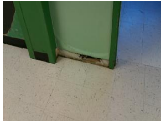
Damaged Gypsum Board
