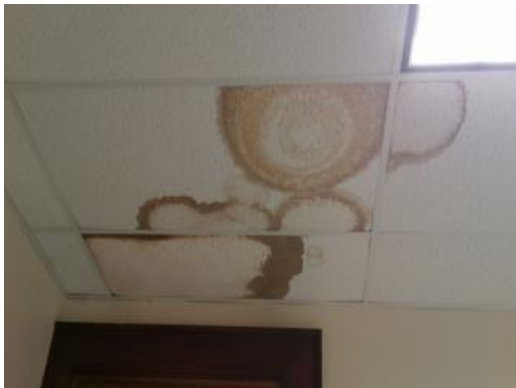
Damaged Ceiling Tile
