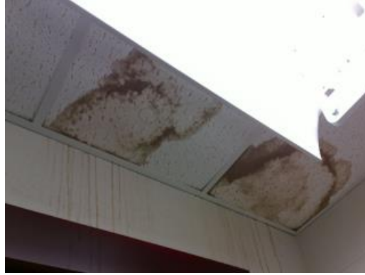
Stained Ceiling Tiles
