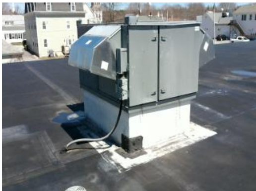
Fan and Outdoor Air Unit
