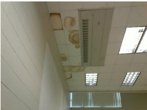
Stained Ceiling Tiles
