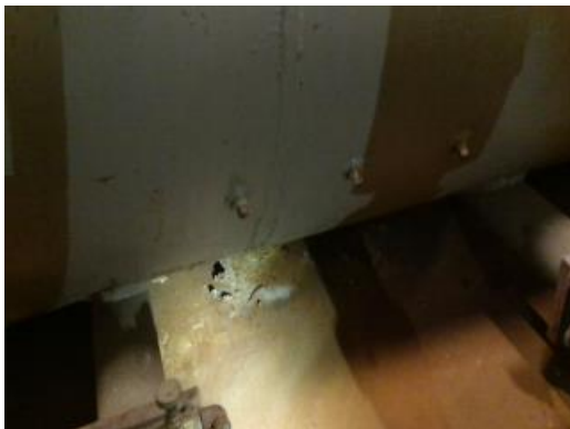
Leakage And Corrosion At Steam Condensate Receiver
