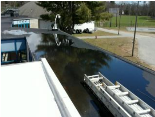
Ponding On Roof
