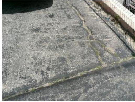
Cracked And Weathered Parking
