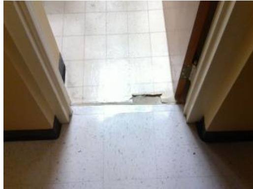
Broken Tile At Doorway
