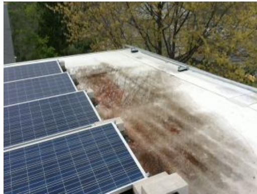
Ponding On Roof
