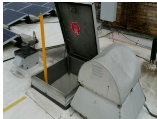
Abandoned Exhaust Fan On Roof
