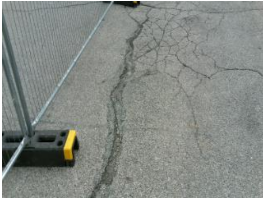
Damaged Parking Lot Pavement
