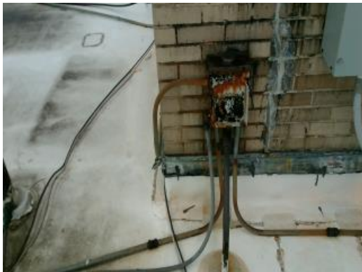
Roof Abandoned Equipment
