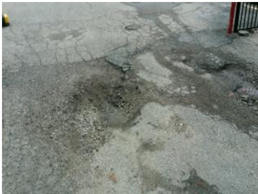
Damaged Parking Lot Pavement
