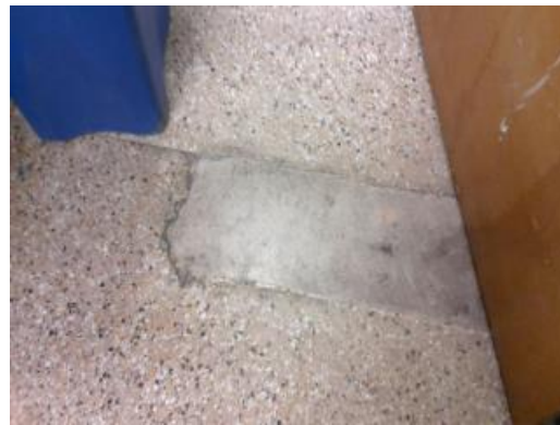
Damaged Terrazzo Flooring
